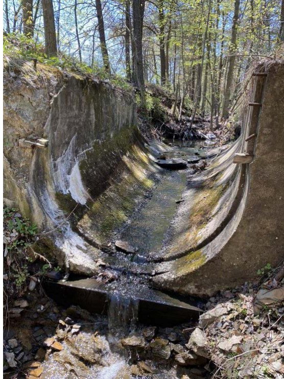
Figure 4-33: E41186777597290 “Lueders Creek Dam” looking at flow in overflow channel between pond and road
