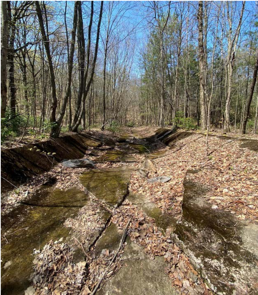
Figure 7. Photo Collage of the Nanticoke Creek Headwaters being lost into the mine workings beneath the deteriorating and abandoned Concrete Flume
