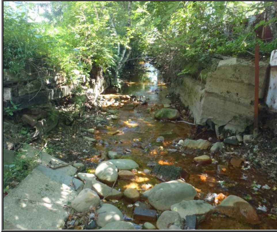
Photo : Constriction point on Sugar Notch Run with concrete retaining walls, railroad ties, and other home-made bank stabilization methods by residents entering Carey's Patch; AMD and filamentous algae present and predominant in the channel with no aquatic life
