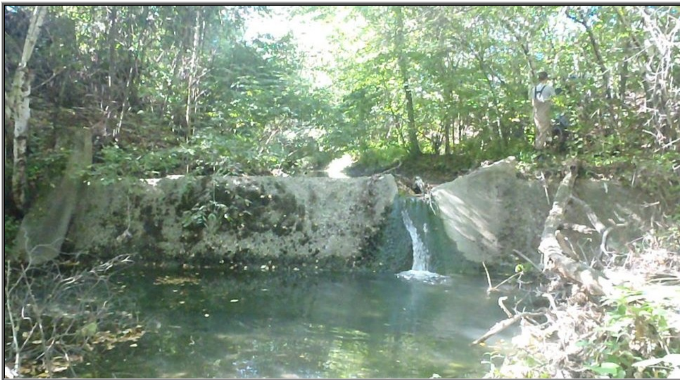
Photo : Looking upstream into Sugar Notch Run at the crack in the concrete dam; 12' in height; 4' pool below the dam; Justyna Sacharzewska, EPCAMR Watershed Outreach and Education Intern working her way around the dam
