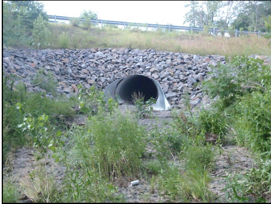
Photo : The upstream side of the squash pipe where Sugar Notch Run is more confined to a stormwater basin as opposed to a stream channel; The guard rail above and road takes you to the WAL-MART Trailer Storage Drop Lot
