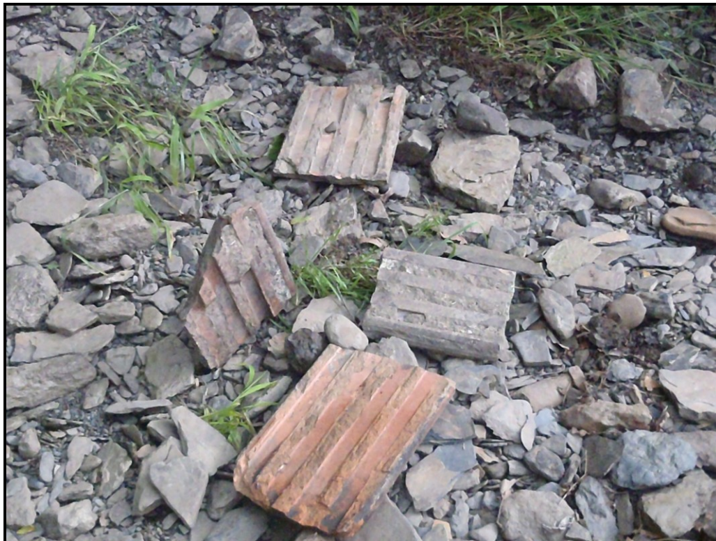
Photo : Terra cotta drain tiles in Sugar Notch Run that have come loose from the floor of the concrete drainage system that is constructed to carry Sugar Notch Run beneath State Route 29
