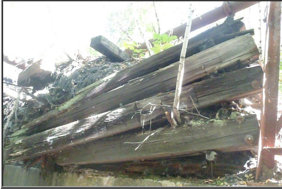
Photo : Railroad siding on the verge of a collapse into Sugar Notch Run adjacent to the abandoned Huber Breaker Colliery Pump House; This area is in need of stabilization as a stream improvement project before the rails fall into Sugar Notch Run and block the railroad tunnel up
