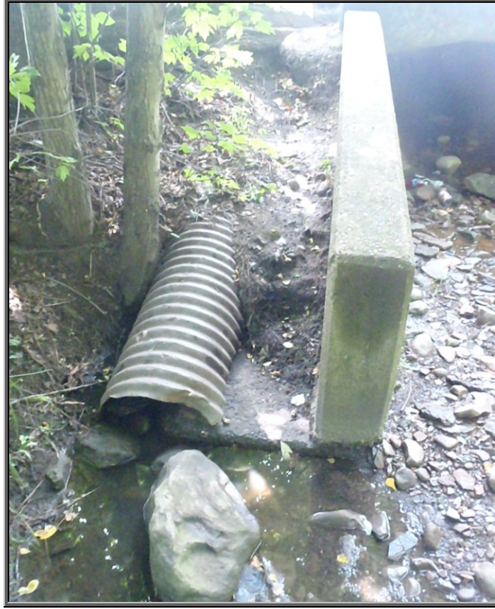
Photo : Sugar Notch Run flowing below Carey's Patch looking upstream towards Sively Street alongside the double-wide culvert where an 18" corrugated stormwater pipe enters the tributary bringing in additional flows during rain events
