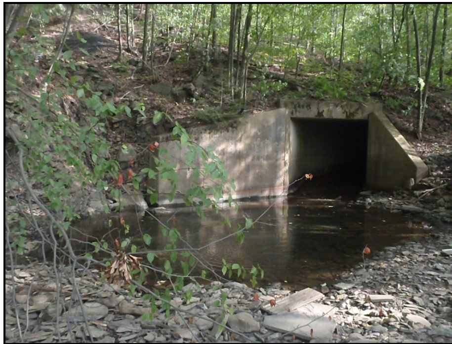
Photo : Sugar Notch Run is pooled at this point upstream in a 3' pool at the outlet of the State Route 29 underpass, however it doesn't flow downstream in the channel at this point and is more than likely lost to the local mine pool in this vicinity
