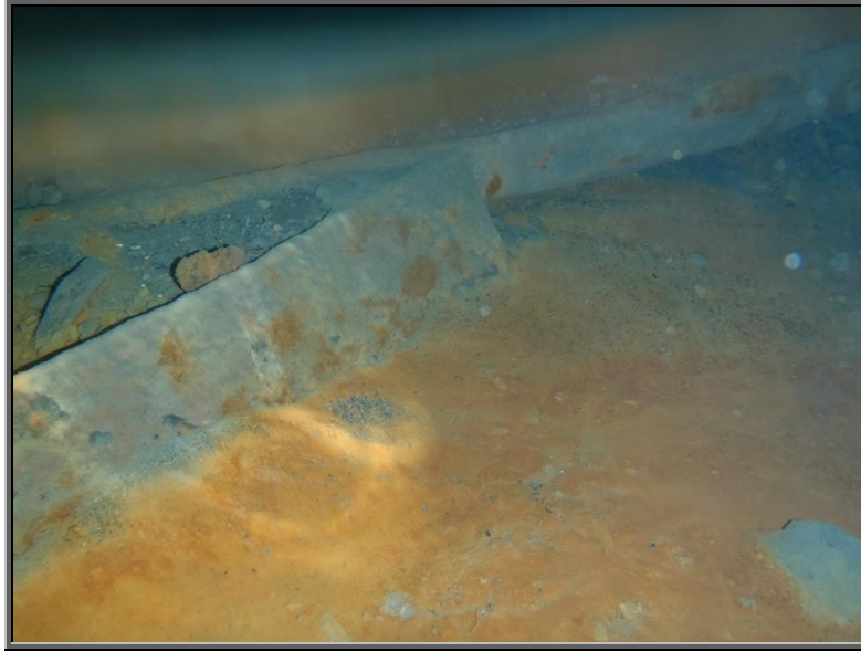
(R) Photo : Rusted rails at the bottom of a 4' deep pool with some iron precipitation on Sugar Notch Run just outside of the railroad tunnel
