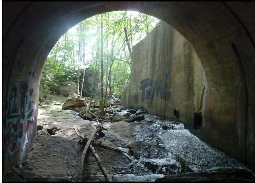
Photo: Looking upstream of Sugar Notch Run as EPCAMR exits from beneath the railroad underpass
