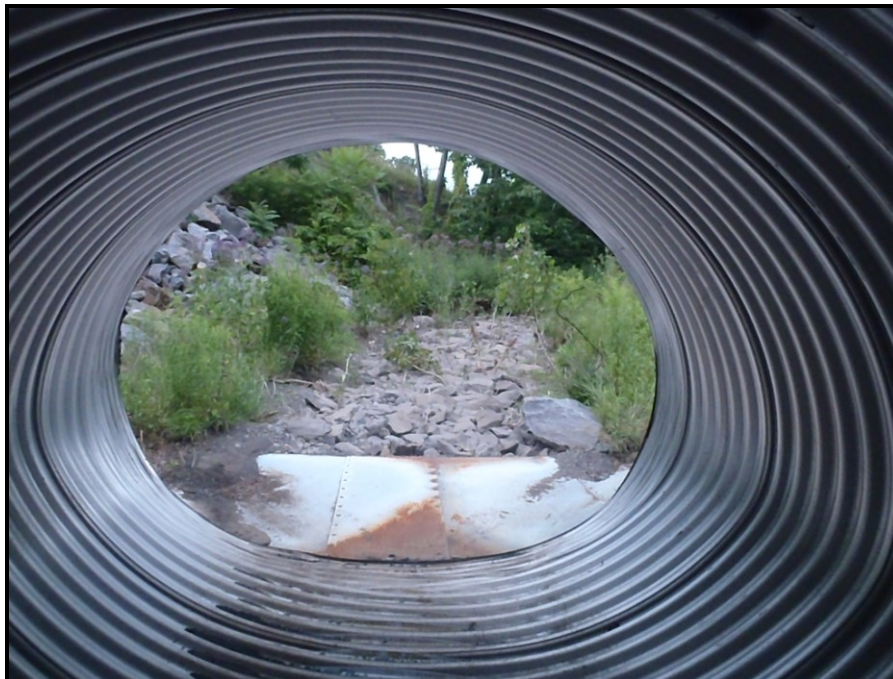
Photo : Looking downstream from inside of a corrugated squash pipe drainage culvert into Sugar Notch Run; WAL-MART stormwater enters from the left side of the bank looking downstream
