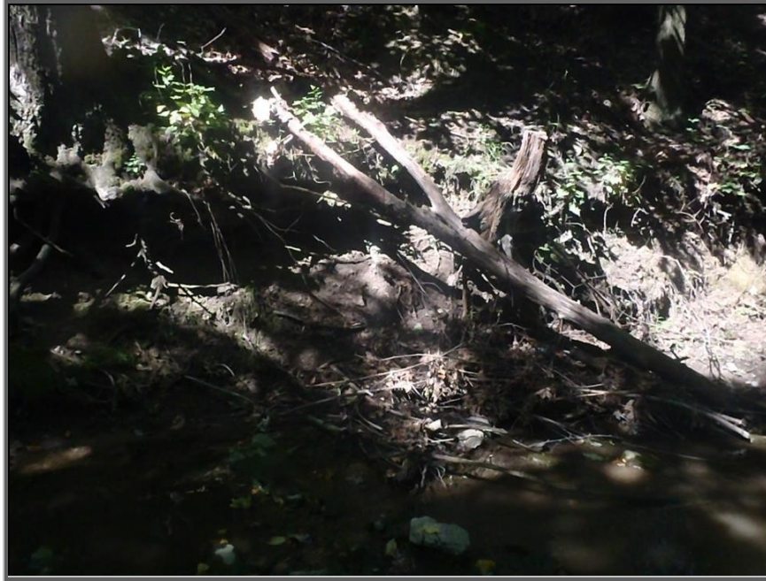
Photo : Minor undercutting of the left bank of Sugar Notch Run probably due to flashy floods on Sugar Notch Run as stormwater scours the area downstream of the railroad tunnel
