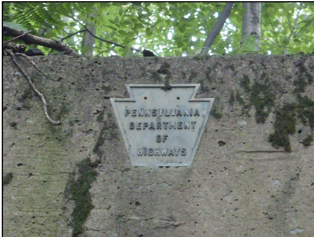
Photo: A closeup of one of the brass PA Department of Highways Keystone plates cemented into the underpass; Seems as if the year of construction name plate might have been stolen from above the plate
