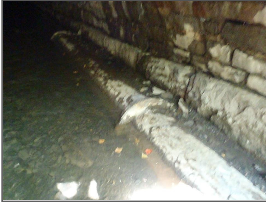
Photo: Partially submerged sanitary sewer line running underneath the railroad tunnel inside the Sugar Notch Run streambed
