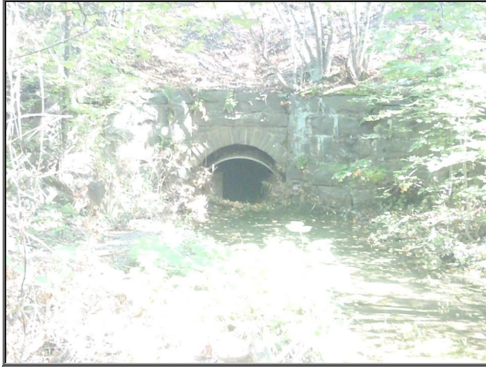
Photo : Old stone arch and corrugated steel culvert at the lower end of the concrete dam creating a ponding area along the wingwalls in Sugar Notch Run; Heavily sediment-laden and full of debris; This potential flooding concern could be easily removed during a stream improvement and habitat restoration improvement project
