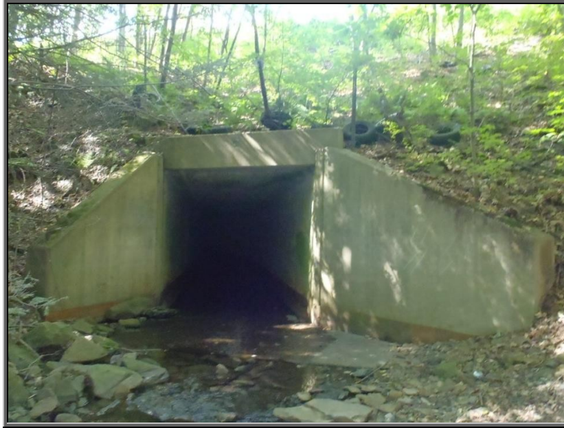
Photo: Looking downstream on Sugar Notch Run at the entrance to the State Route 29 underpass tunnel with a tire pile above header of the structure
