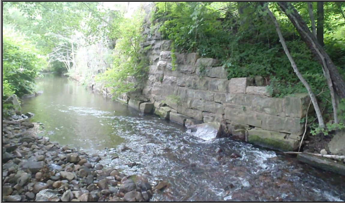
Photo : Looking downstream 200' below the confluence of Sugar Notch Run with the Solomon Creek Main Stem at one of the abandoned railroad bridges that was constructed in 1902.
