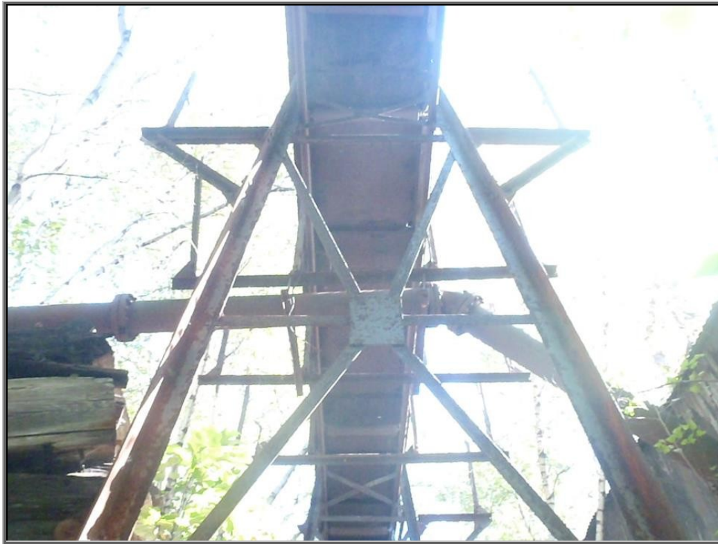
Photo : Iron works plumbing, conveyor scaffold support, and pump pipe main running from the Huber Breaker Colliery Pump House on the right over to a lateral that carried water to the Dorr Thickener and the Menzies Cones where the coal was "floated" and separated
