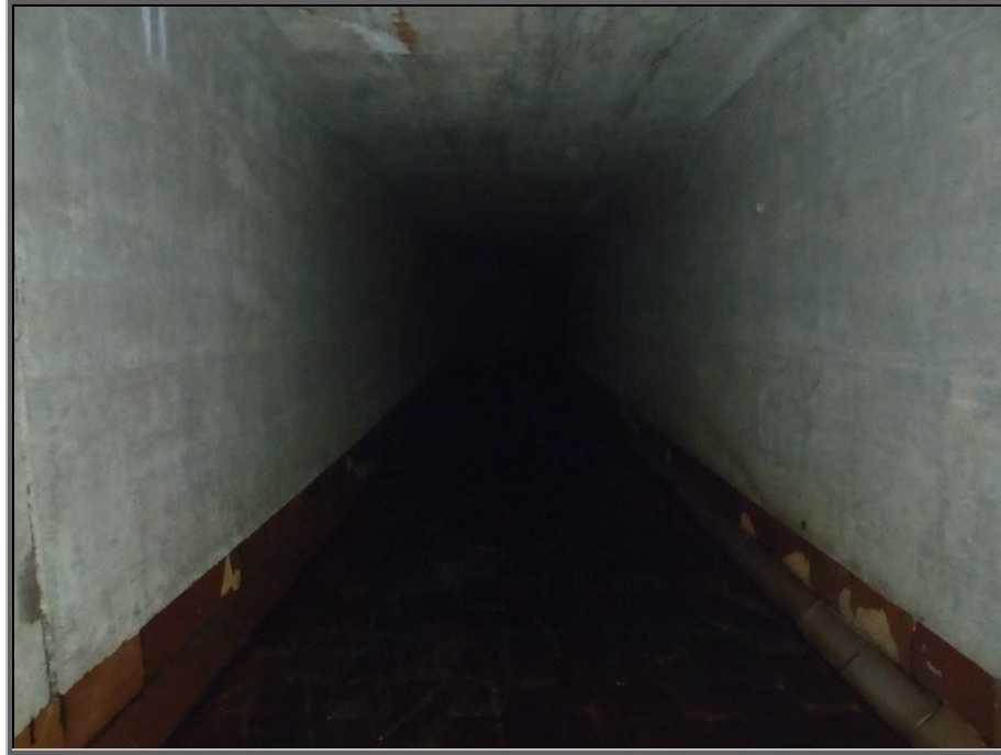
Photo: Entering the terra cotta lined State Route 29 Underpass tunnel that carries Sugar Notch Run looking upstream into the several hundred foot tunnel
