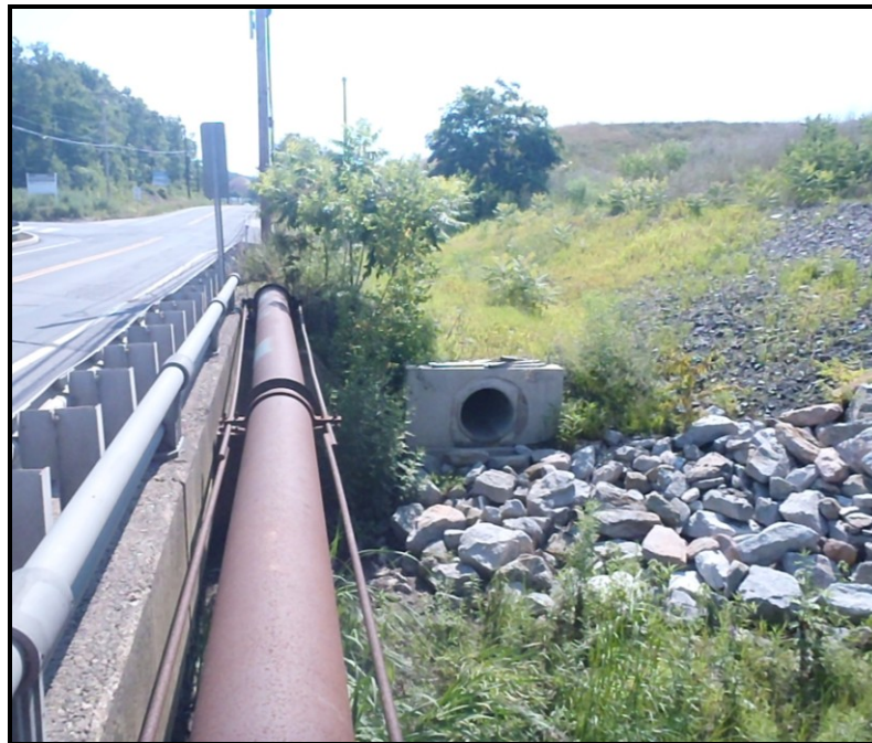
Photo : Storm water drainage outlet with rock apron into Sugar Notch Run along S. Main Street looking south
