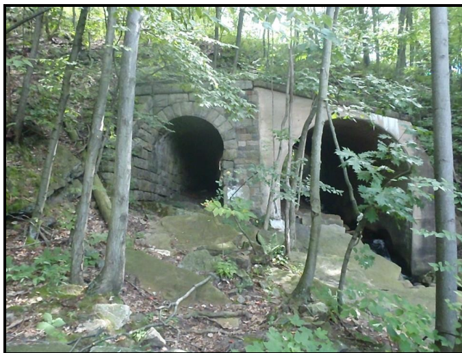
Photo: Old and new railroad underpasses with Sugar Notch Run flowing through the right hand tunnel; built right into the bedrock
