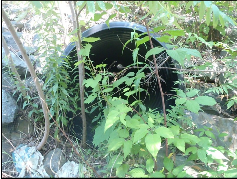
Photo: A stormwater pipe entering the left bank of Sugar Notch Run just upstream of the culvert drainage system beneath Preston Road
