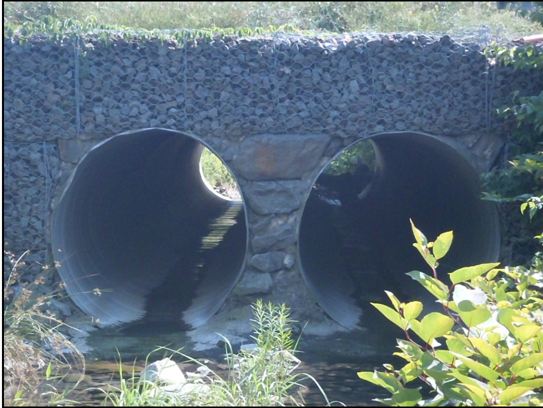
Photo : A tree that is nearly 20' long with its rootwad in lodged in the culvert on the right hand side of the split flow on Sugar Notch Run
