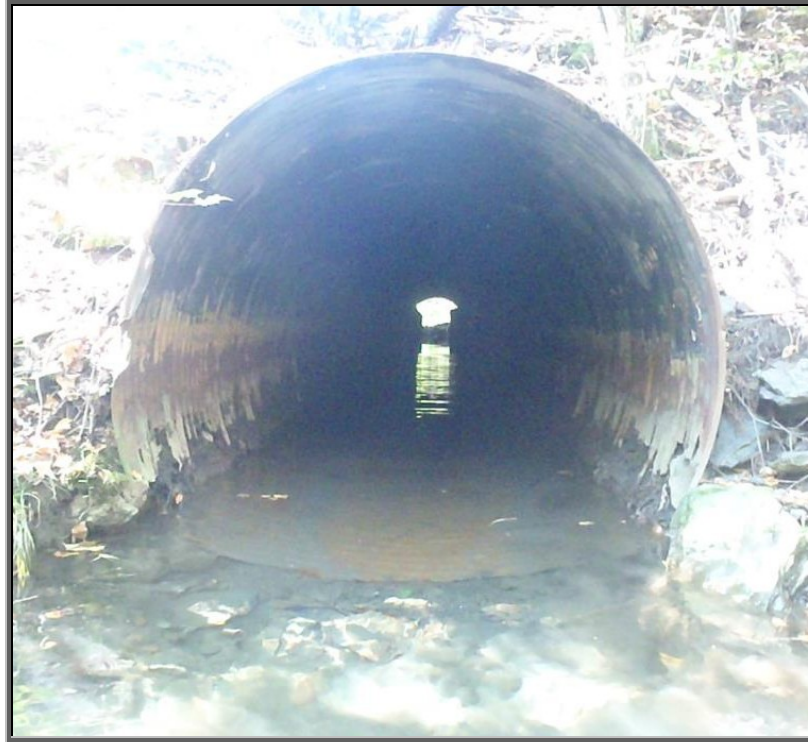
Photo : Looking upstream into 5' corrugated pipe carrying Sugar Notch Run under an abandoned haul road behind the Preston section of Ashley Borough
