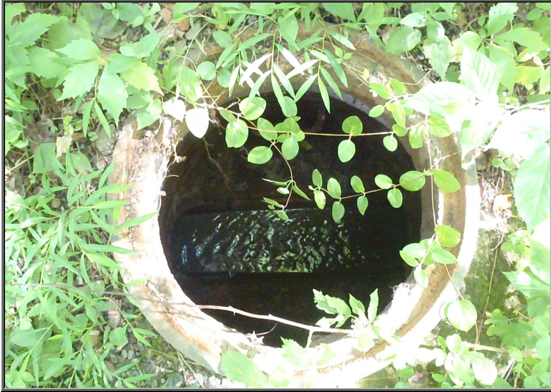
Photo : A sanitary sewer line manhole that is completely missing from this main line just beyond railroad tunnel; EPCAMR will recommend that a new lid be placed on it by either Ashley Borough or the WVSA
