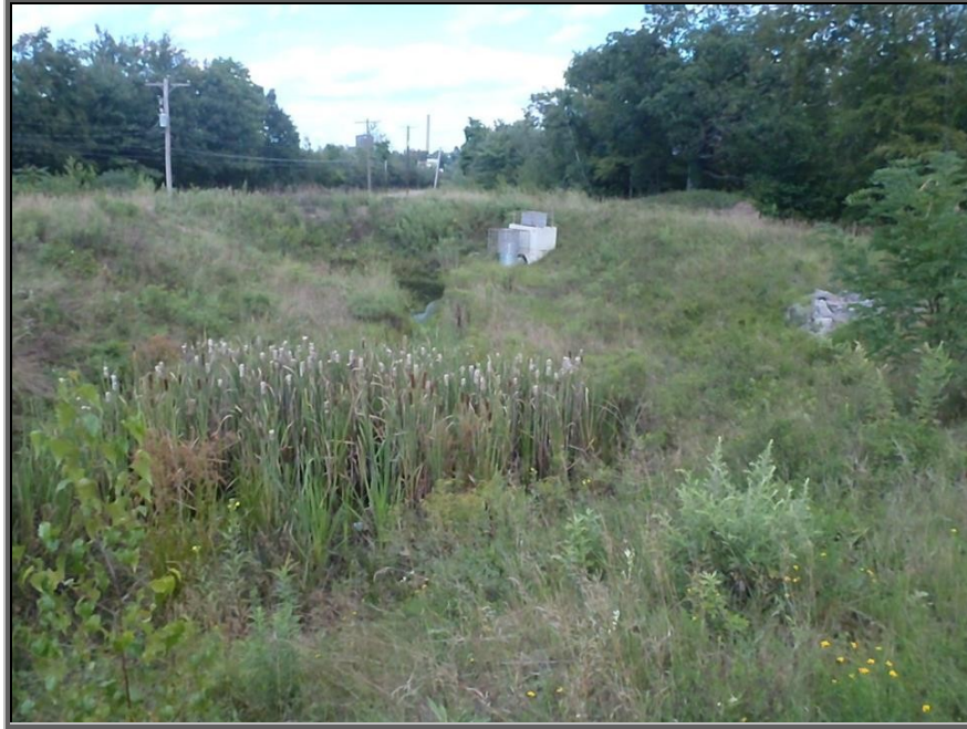
Photo: WALMART Lot Stormwater Detention/Wetlands Basin with a drop inlet structure that empties into Sugar Notch Run to the east of the riser pipe
