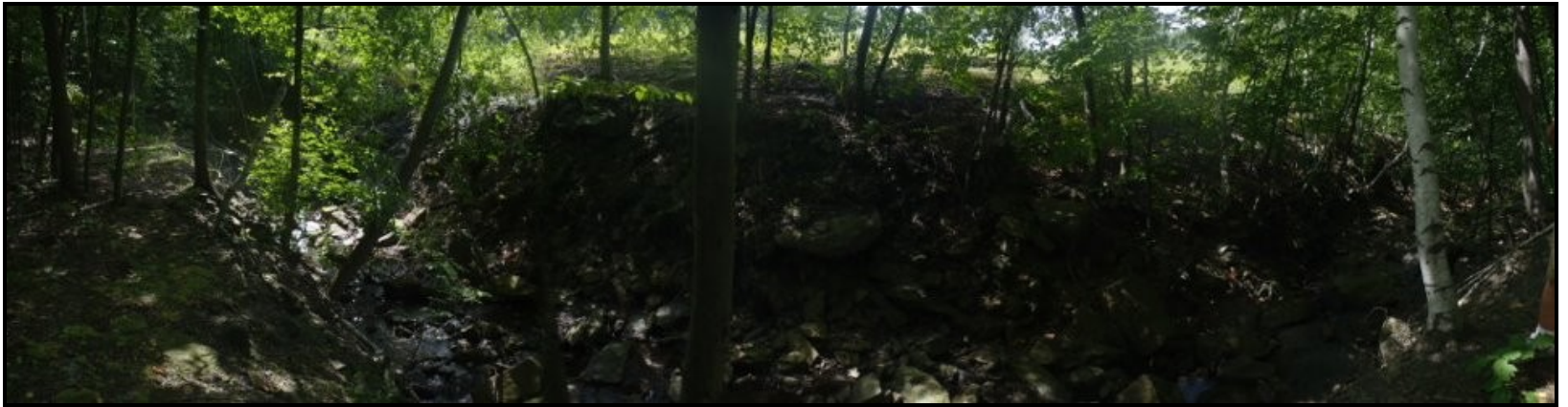
Photo: Extremely undercut and incised channel below the railroad underpasses into Sugar Notch Run
