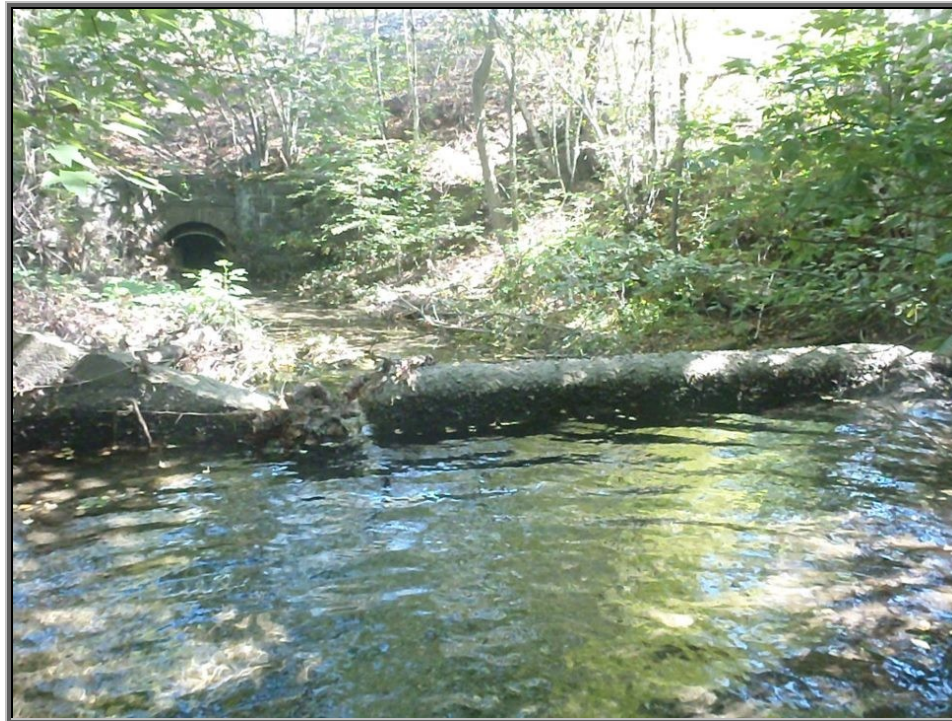
Photo : Old concrete dam possibly connected to the Huber Colliery Operations on Sugar Notch Run with an old railroad stream culvert and stone arch tunnel in the background; Crack in concrete near leaf blockage near the middle of the dam
