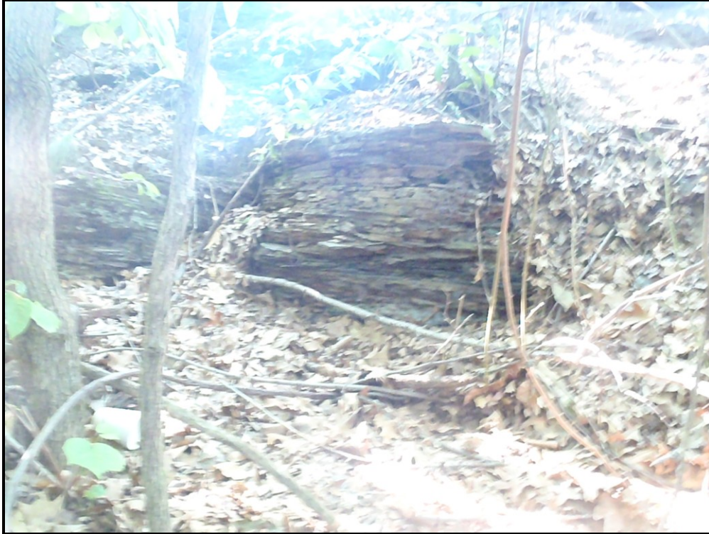
Photo: A shaley outcrop along the right bank looking upstream on Sugar Notch Run that has eroded to the point where stormwater from South Main Street has entered this section and cut down into the fracture shale and caused it to break up into the channel
