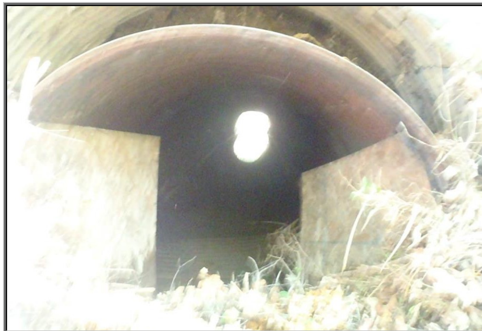
Photo : Culvert blocked by woody debris, leaf packs, and two large pieces of plywood that could lead to future flooding problems if not removed; Sugar Notch Run flowing through the culvert downstream towards Carey's Patch; This potential flooding concern could be easily removed during a stream improvement project
