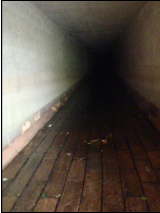
Photo: Entering the terra cotta lined State Route 29 underpass tunnel that carries Sugar Notch Run looking upstream into the several hundred foot tunnel; Sugar Notch Run was flowing through the underpass across the entire length of the terra cotta floor to a depth of 1”
