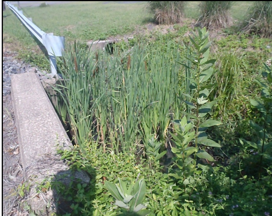
Photo : Drainage culvert along S. Main Street in Ashley that carries storm water across the street to Sugar Notch Run
