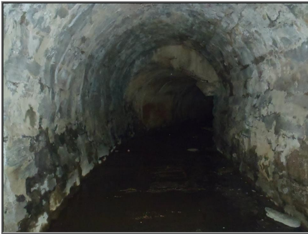
Photo: Old masonry meets new masonry work at the bend in the tunnel; Sugar Notch Run flows over wooden timbers on the left hand-side of the channel within the tunnel
