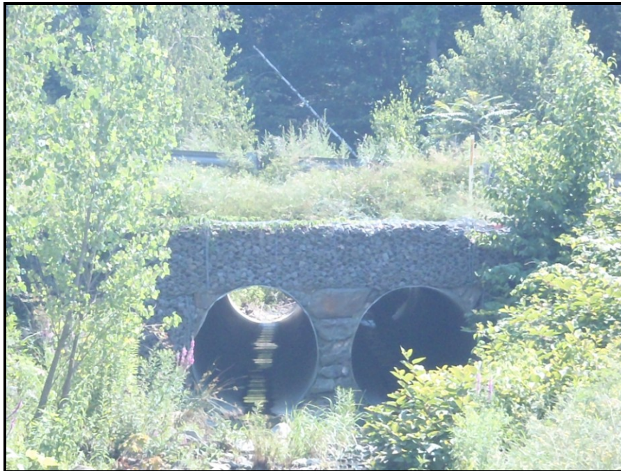
Photo : Double corrugated drainage pipes under Preston Road looking upstream on Sugar Notch Run just off S. Main Street
