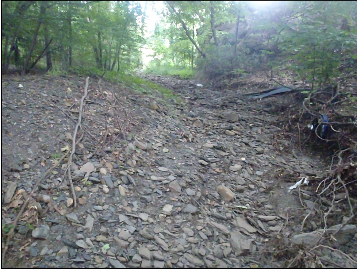
Photo : Looking upstream on Sugar Notch Run which is entirely dry and loaded with sediment, gravel bars, coal silt, and culm material
