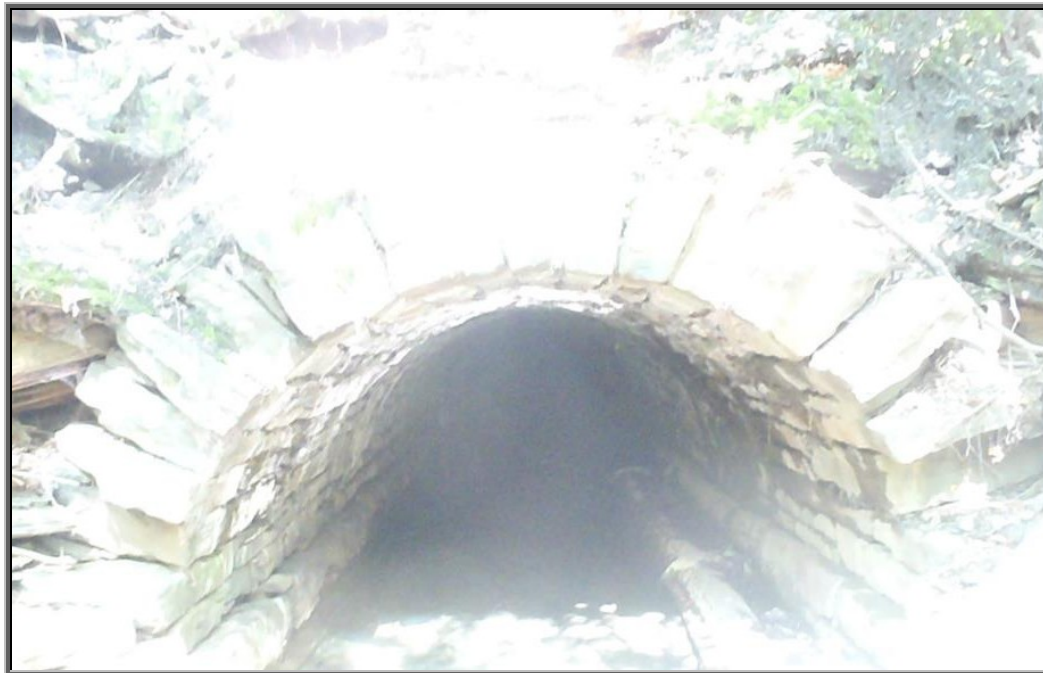
Photo: Looking into the stone arch railroad tunnel crossing and one of the submerged Ashley sanitary sewer mains or WVSA main along with Sugar Notch Run flowing downstream behind the Preston section of Ashley Borough
