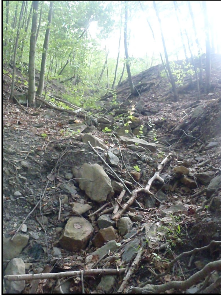
Photo : A stormwater overflow channel that is very steep that drains runoff from the off ramp of State Route 29 onto S. Main Street at the light; The PA DOT Maintenance Facility Shed is located upstream and adjacent to this draw to the right of this area
