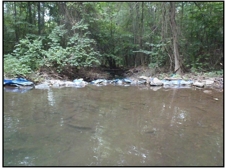
(R) Photo: Looking downstream into the pool and man-made dam on Sugar Notch Run; This dam could easily be removed to prevent a potential flooding hazard downstream as a stream channel improvement project
