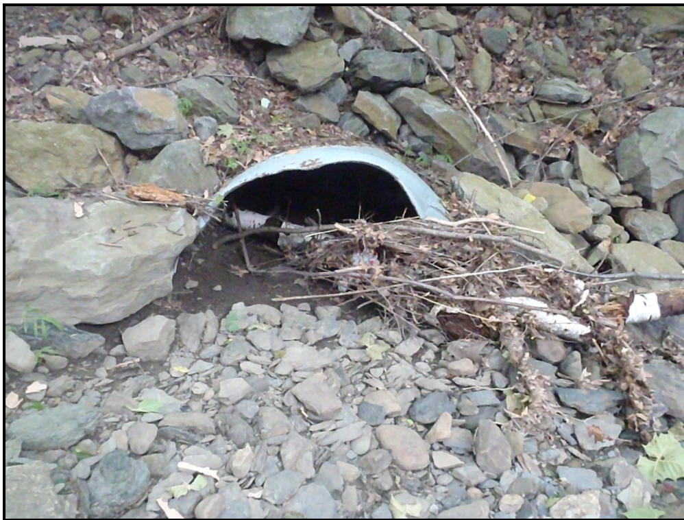
Photo : The left drainage pipe is entirely blocked on the upstream side of Sugar Notch Run which is dry and has already experienced high water and storm events that have deposited all of the smaller rock material in a gravel bar deposition just above both pipes
