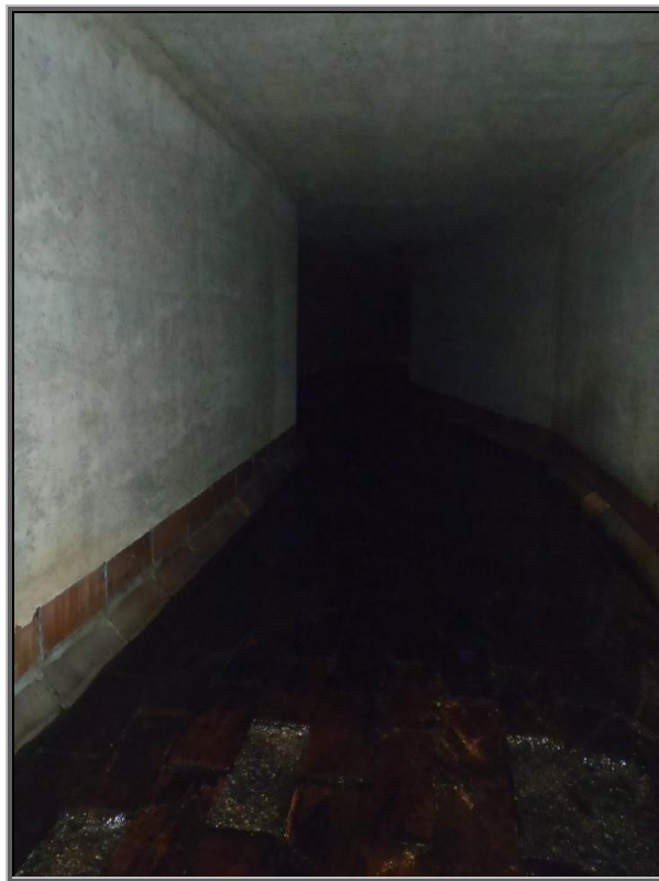
Photo: A few missing tiles here are probably the ones that were found below the pool downstream in Sugar Notch Run
