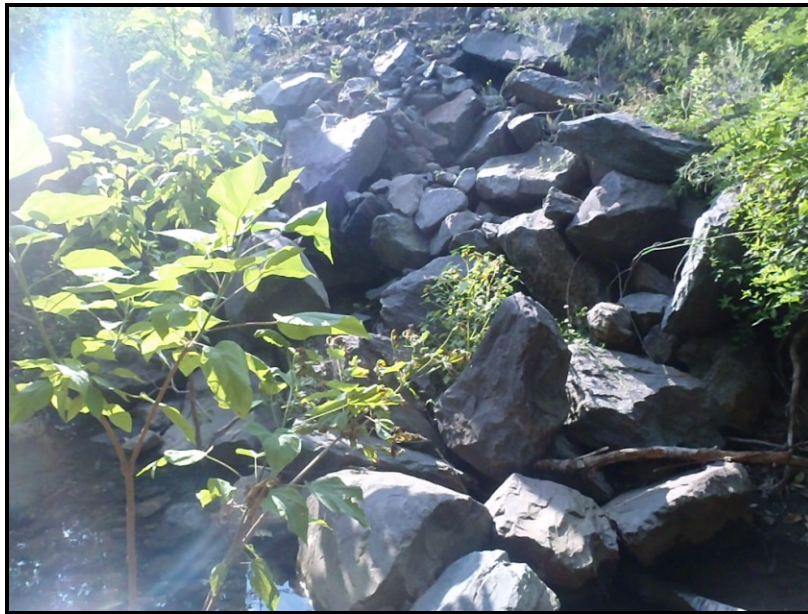
Photo: A rock-filled stormwater drainage area backfilled at some point to prevent further erosion of the channel along the right bank of Sugar Notch Run
