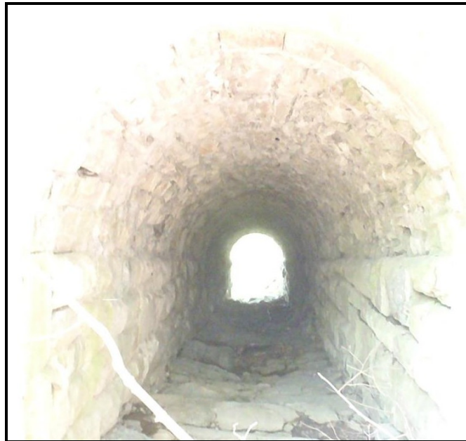
(R) Photo: A shot of the older constructed masonry cut stone underpass looking down the other side of the railroad tunnel
