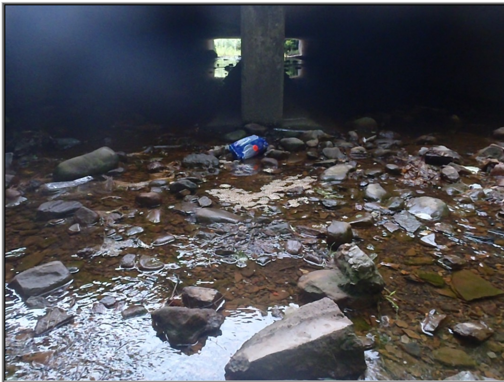
Photo : Sugar Notch Run flowing below Carey's Patch looking upstream towards Sively Street into the double-wide culvert full of debris that could easily be cleaned out as a part of a restoration project
