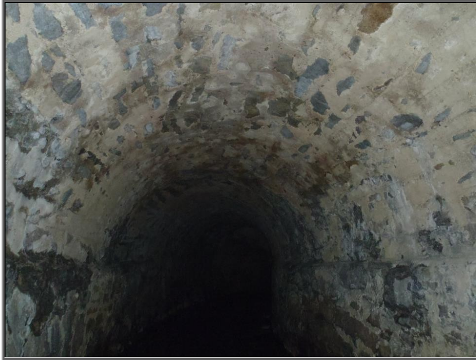
Photo: Grout work touch ups at a bend in the railroad tunnel; Walking into the darkness
