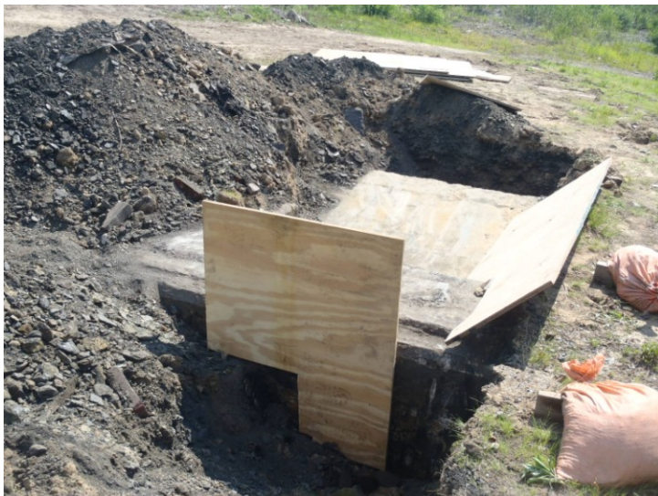
Forming up the sides of the footer for the Huber Breaker Miner's Memorial on top of the former abandoned Engine House Foundation in Ashley
