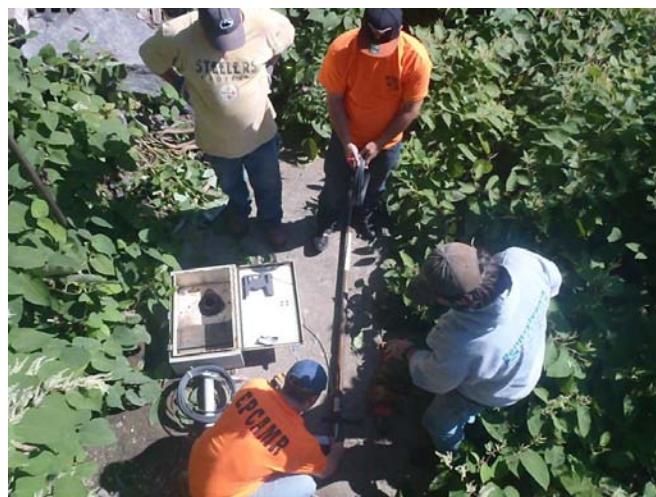
Zip tying & duct taping pressure transducer cables to the pipes before placing down the Old Forge Borehole
