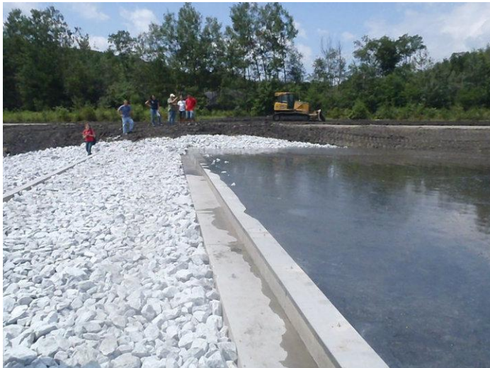
Partners watch as the Silver Creek AMD Treatment System fills up for the first time.
