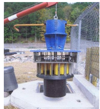
Micro-hydro turbines installed at the Audenreid Treatment System
