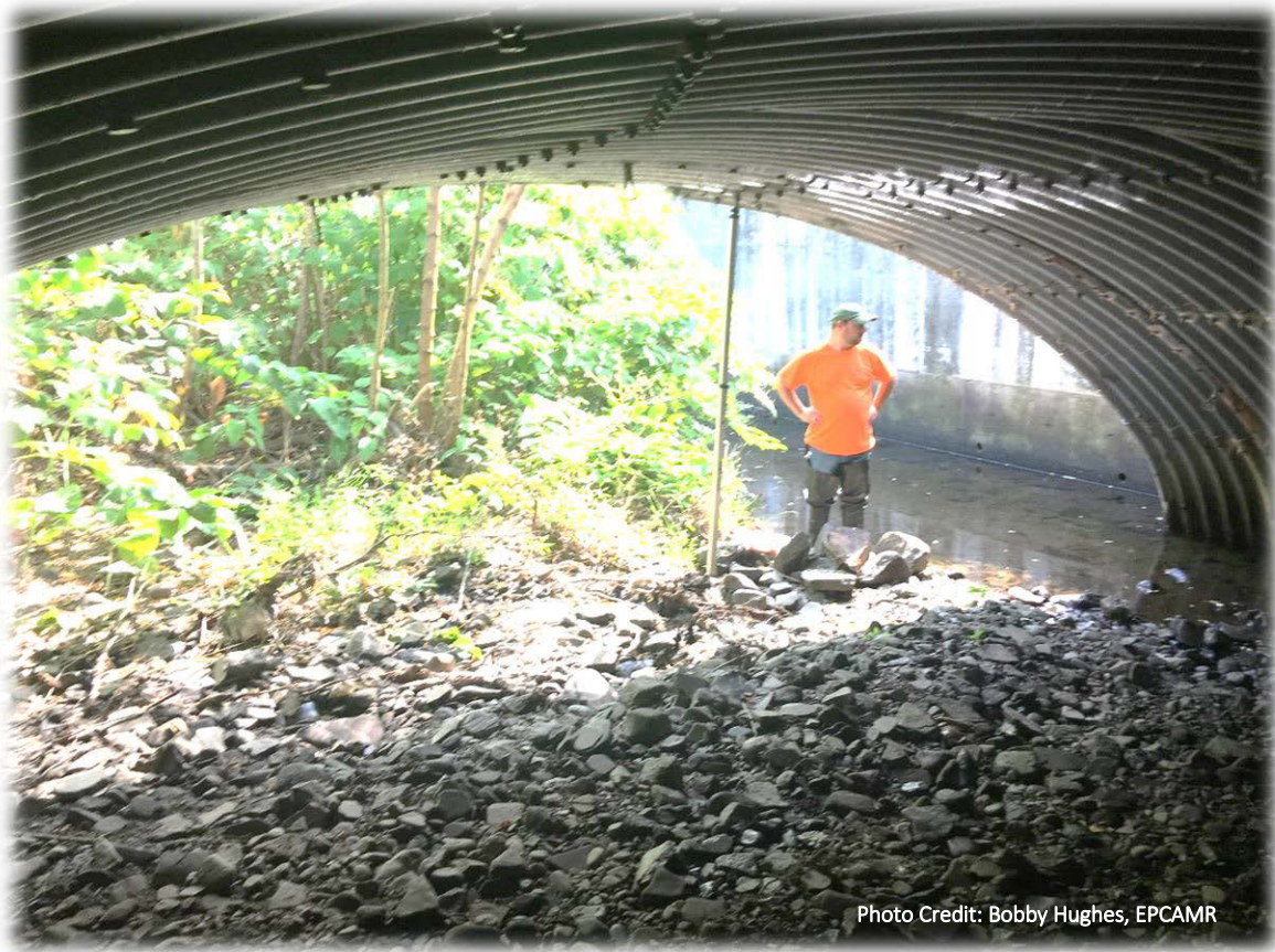
Figure 7. Tom Mayka, DAMA Stormwater Coordinator surveying the conditions of Toby Creek at outlet of the large corrugated metal culvert east of Dunkin Donuts on the Dallas Memorial Highway before conducting the AOP Assessment.
