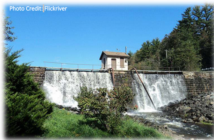
Figure 13. Overflow from the Huntsville Dam in the Huntsville Creek subwatershed of larger Toby Creek Watershed 36
