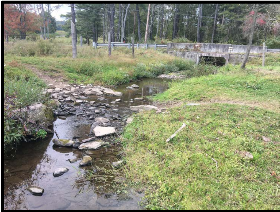
Figure 26. A stream crossing on the unnamed headwater tributary to the Huntsville Reservoir looking upstream toward the concrete bridge culvert on Park Road (T-597) in Dallas Township, PA
