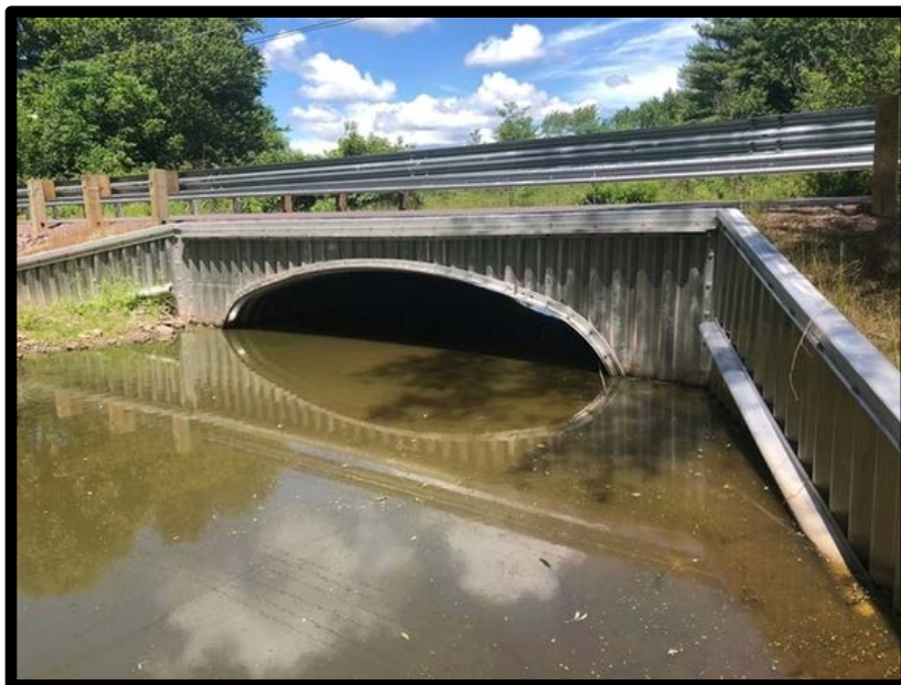
Figure 4. Newly installed bridge culvert near Yalick Farms where the headwaters of Huntsville Creek flows beneath Reservoir Road before heading towards the Luzerne County Fairgrounds
