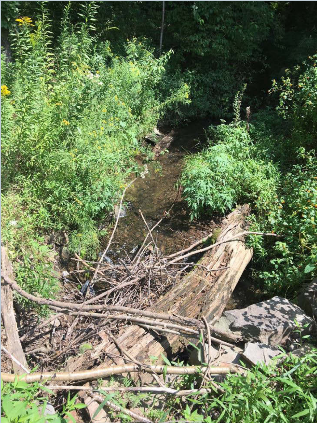
Figure 178. A shot taken looking upstream on the UNT to the northeast of Dug Road, where large woody debris is found blocking the culvert from a previous high-water event. The debris pile can easily be removed by hand to make the UNT passable through the pipe culvert.
