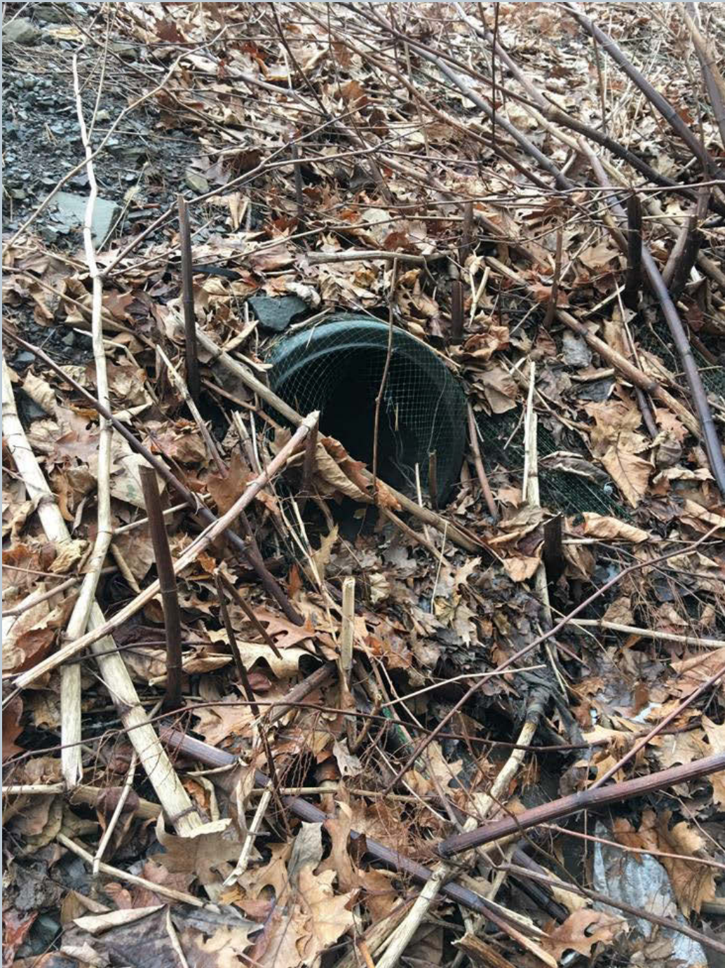
Figure 138. A 24-inch black HDPE stormwater outfall pipe (dry) structure that is not aligned with Toby Creek.
