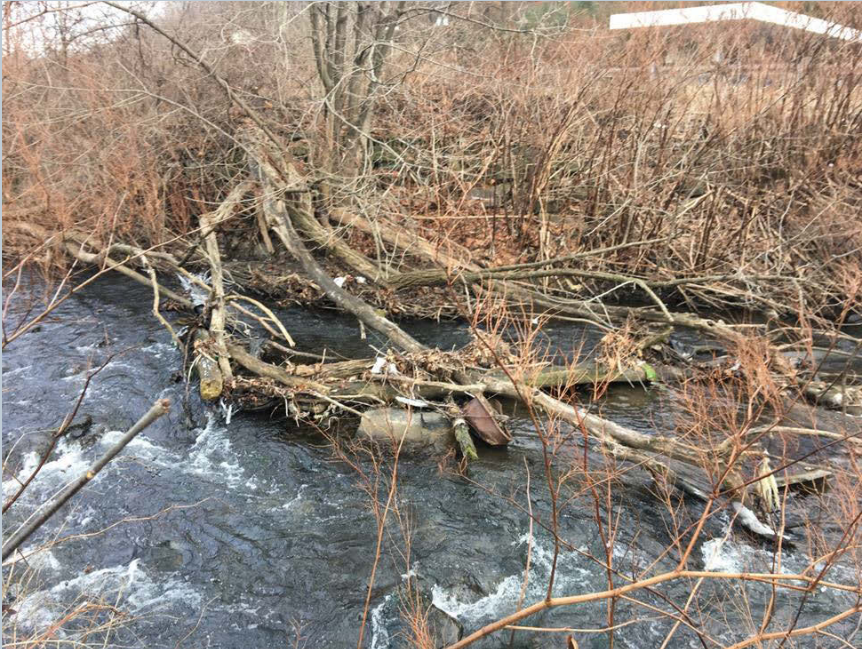
Figure 106. A very large fallen tree and some woody debris that has landed in Toby Creek, redirecting flow to one of the boxes in the bridge. This has created a gravel bar deposition behind the tree, just upstream of the bridge over State Route 309, along S. Main Street.
