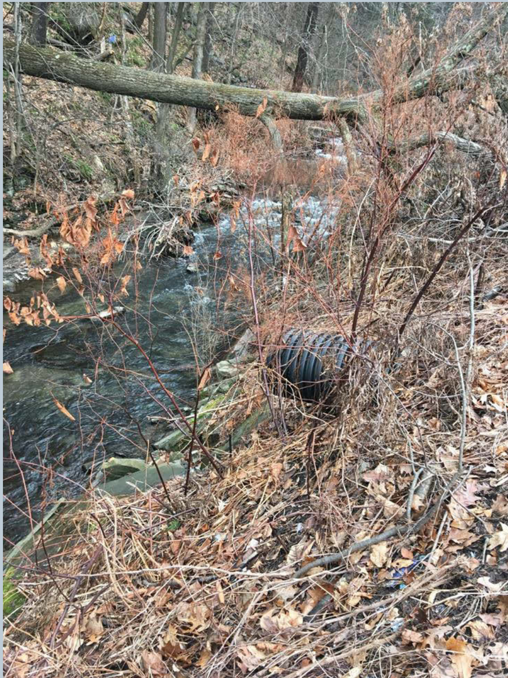
Figure 137. A 24-inch black HDPE stormwater outfall pipe (dry) structure that lies perpendicular to, and is not aligned with, Toby Creek.
