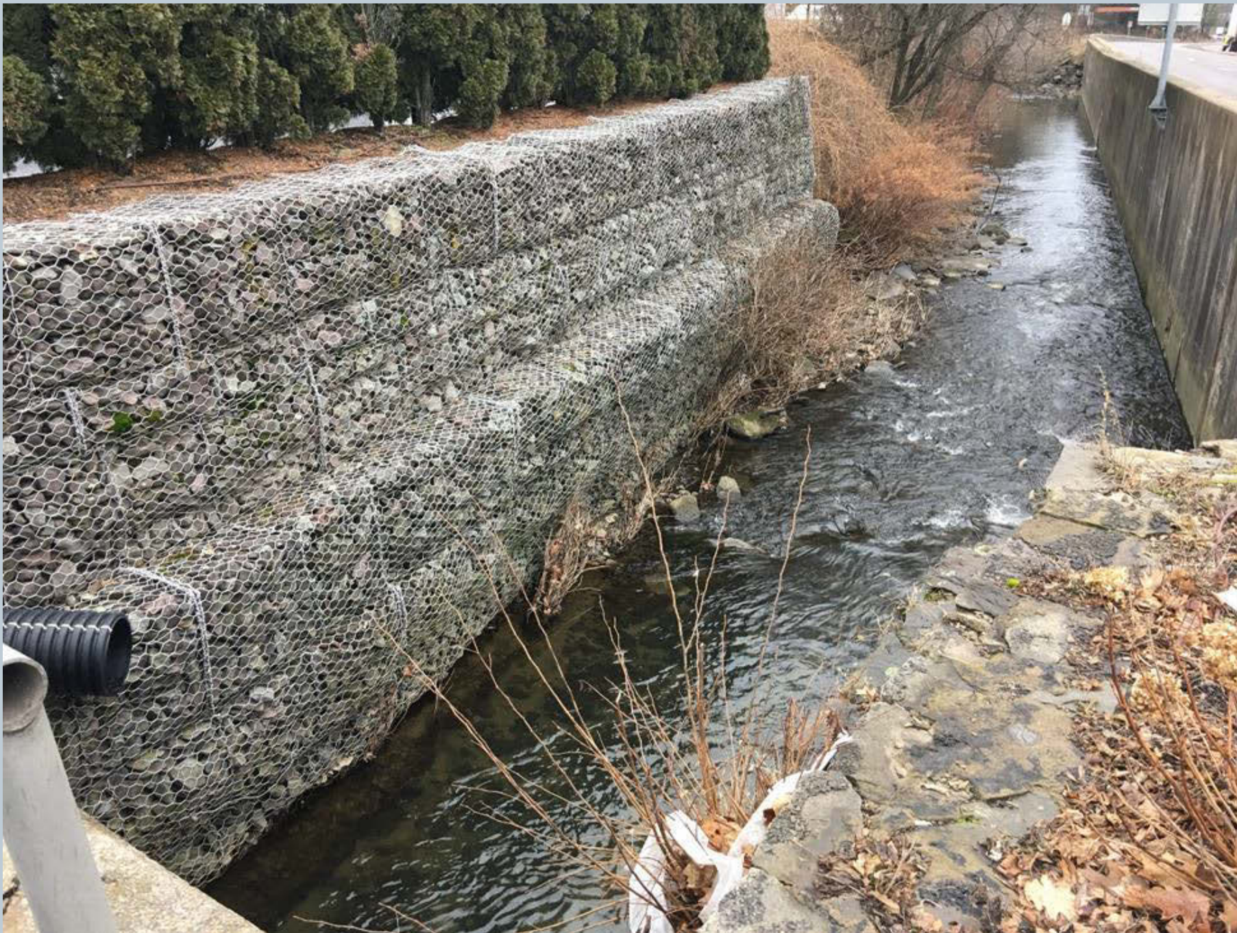
Figure 144. Looking downstream on Toby Creek from the Age of Innocence Parking Lot, gabion rock-filled baskets are in place as a stabilization project along the left wall for nearly 200-feet. There is a 12-inch black corrugated HDPE pipe is floating 9-foot above the Toby Creek draining parking lot.
