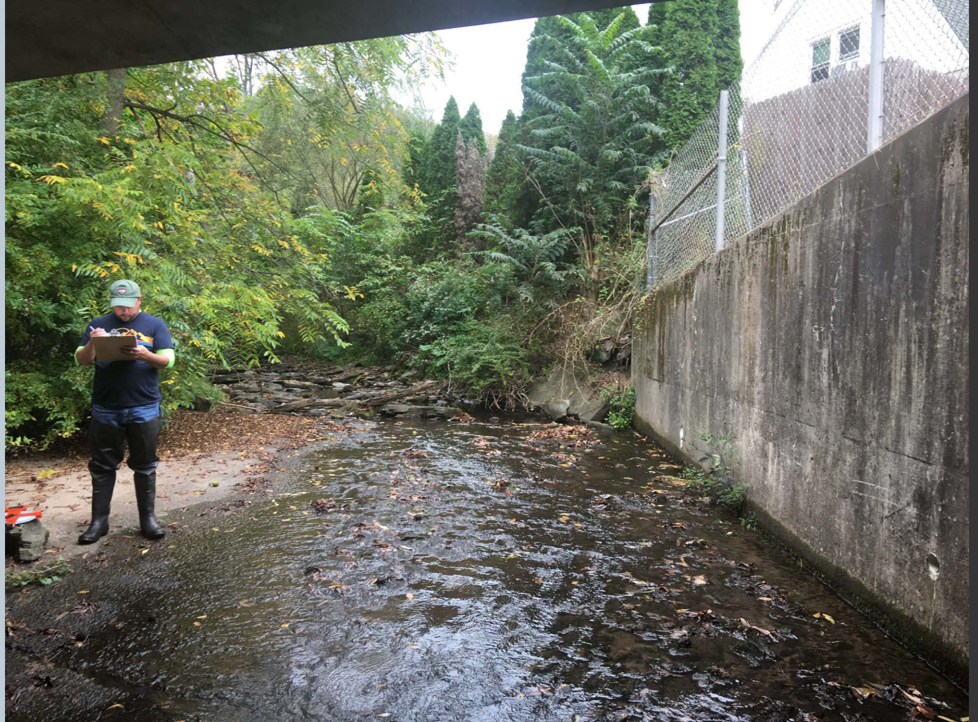
Figure 301. Bridge culvert over Carverton Road looking upstream on the unnamed tributary with Tom Mayka, DAMA Stormwater Coordinator where the concrete footer meets the unnamed tributary.
