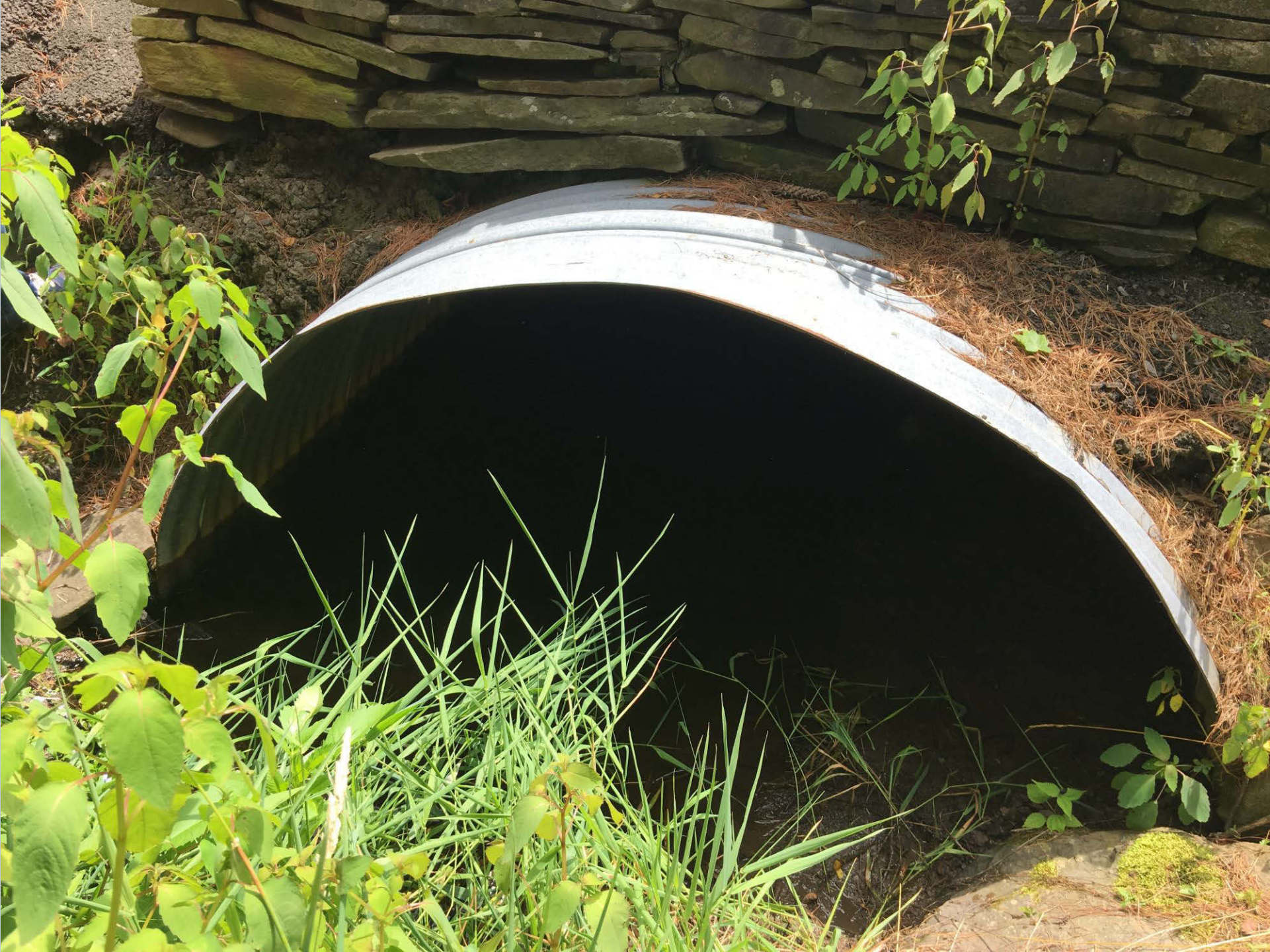
Figure 211. An unnamed tributary to Toby Creek at an inlet of corrugated metal pipe on Glenn Riddle Lane with a moderate constriction.
