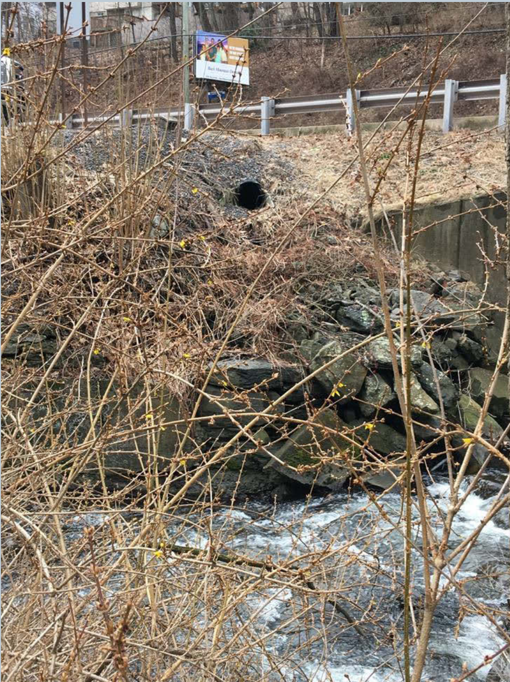
Figure 134. A 24-inch black HDPE stormwater pipe (dry) not aligned on State Route 309. This location is just before the bridge that is north of the Car Mix lot.
