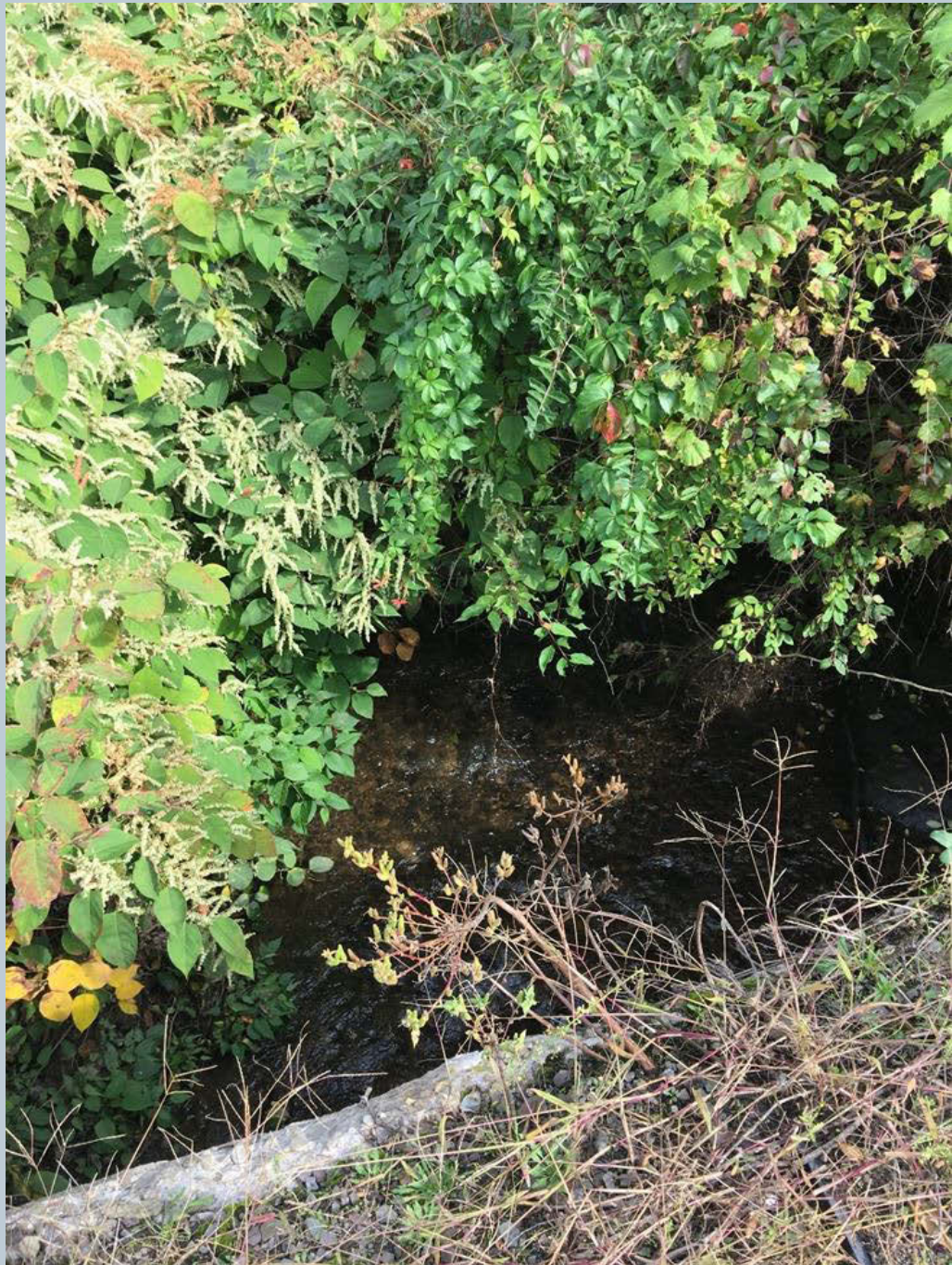
Figure 57. A shot of an unnamed tributary that flows through a box culvert before entering Toby Creek just above Amelia's Diner.
