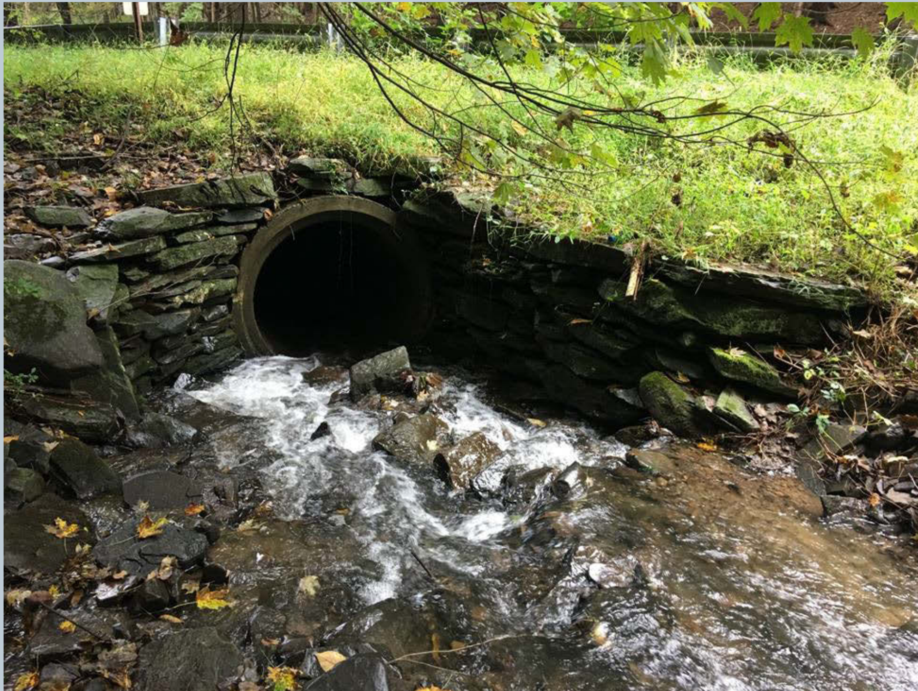
Figure 29. The Green Pond unnamed tributary looking downstream along E. Center Street. This is a shot of a 36-inch concrete pipe culvert with a masonry headwall. The left wall is failing, and the headwall can easily be reconstructed by hand.
