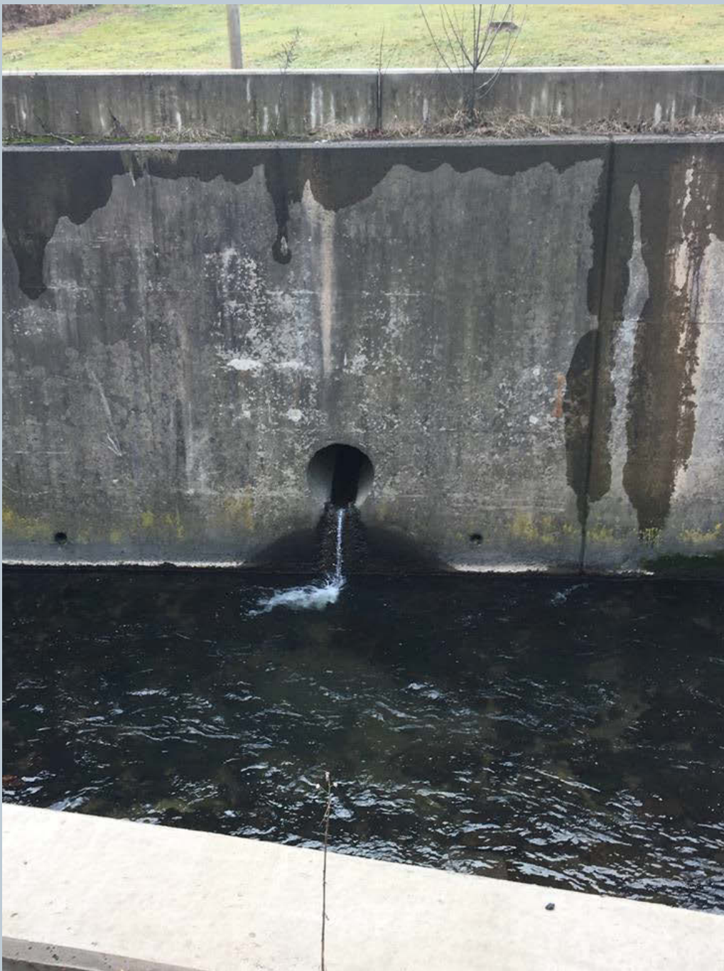
Figure 116. Flowing through the lower portion of the retaining wall, an UNT from Mt. Greenwood Cemetery flows into Toby Creek.
