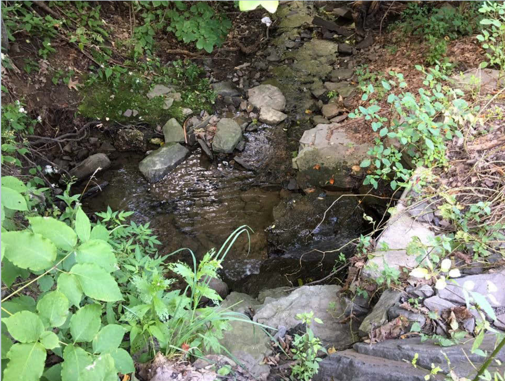
Figure 186. A shot of another UNT flowing downstream through an 18-inch or 24-inch black HDPE culvert pipe along Manor Road. The downstream outlet from the pipe culvert has a small scour pool and highly eroded streambank opposite the pipe that could use some rock reinforcement along the streambank or willow staking to reinforce the streambank and stabilize it.
