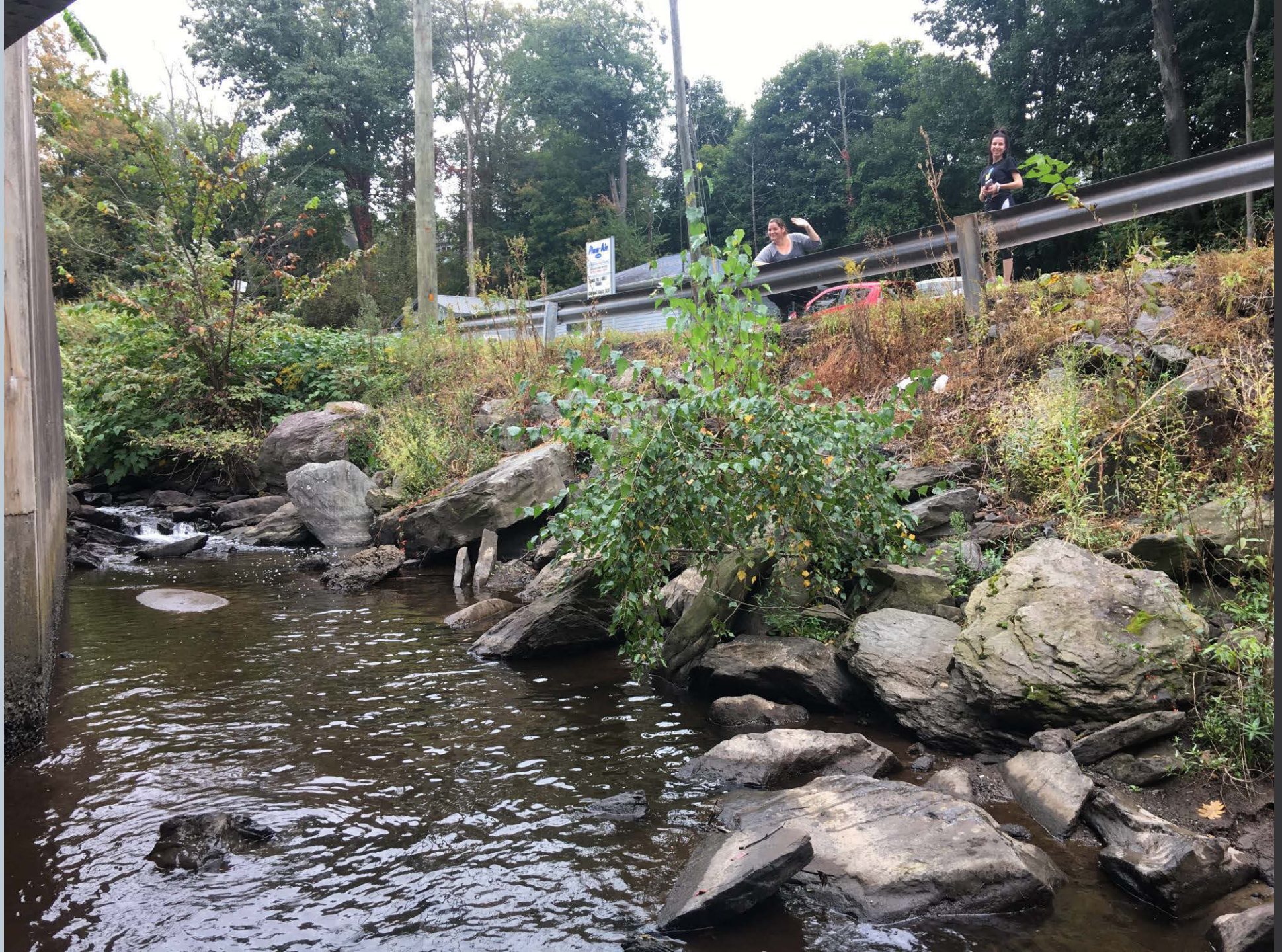
Figure 278. Looking upstream on Toby Creek standing in front of the inlet side of the bridge culvert over the Dallas Memorial Highway. Large rip rap rock has been placed along the streambank along N. Main Street to prevent further erosion. DHL/EPCAMR Volunteer is taking notes.
