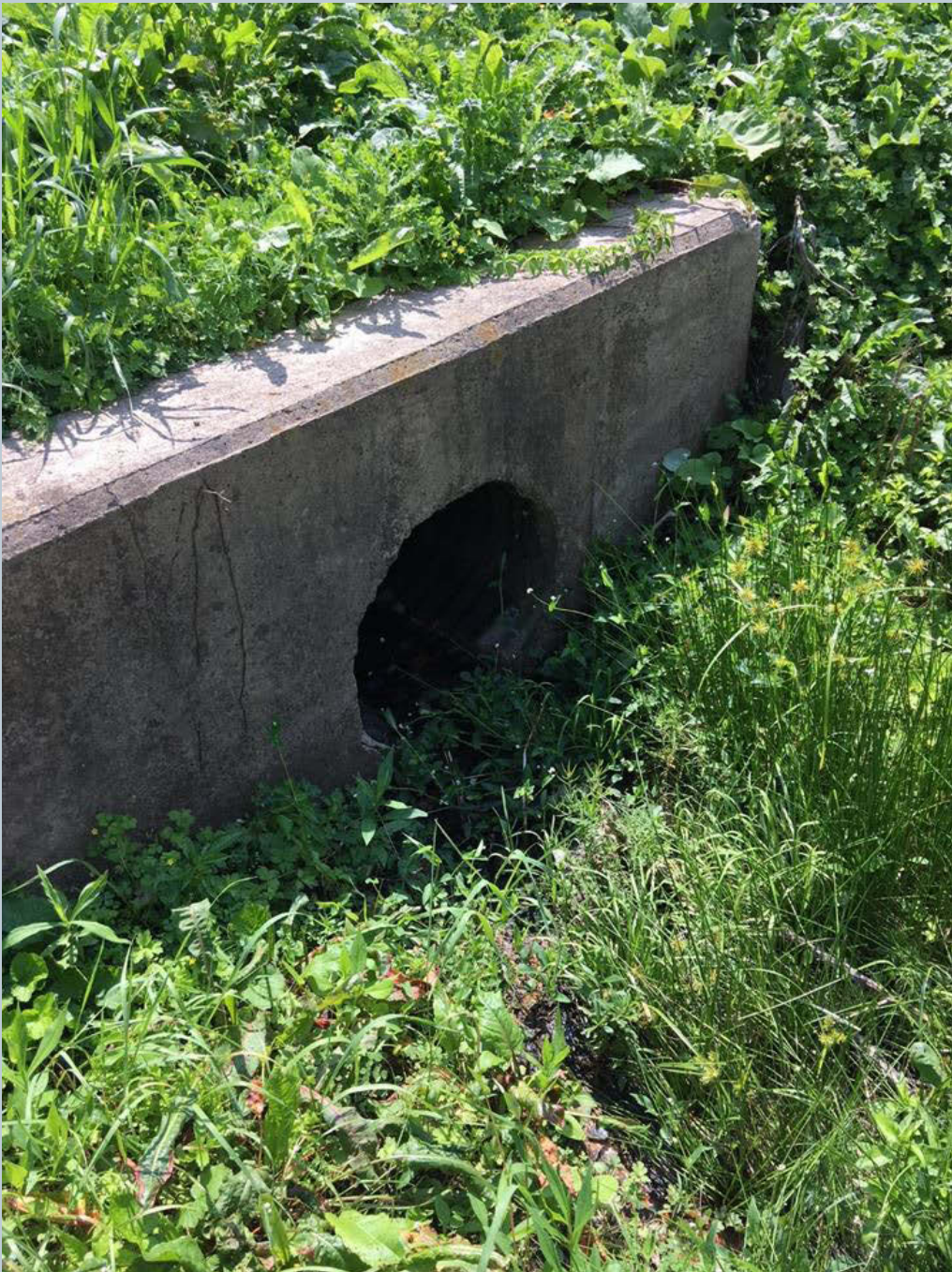
Figure 174. A shot of an 18-inch or 24-inch corrugated pipe and headwall to the larger wetlands complex, located downstream of Dug Road. This pipe is located between Terrace Road and Carverton Road.
