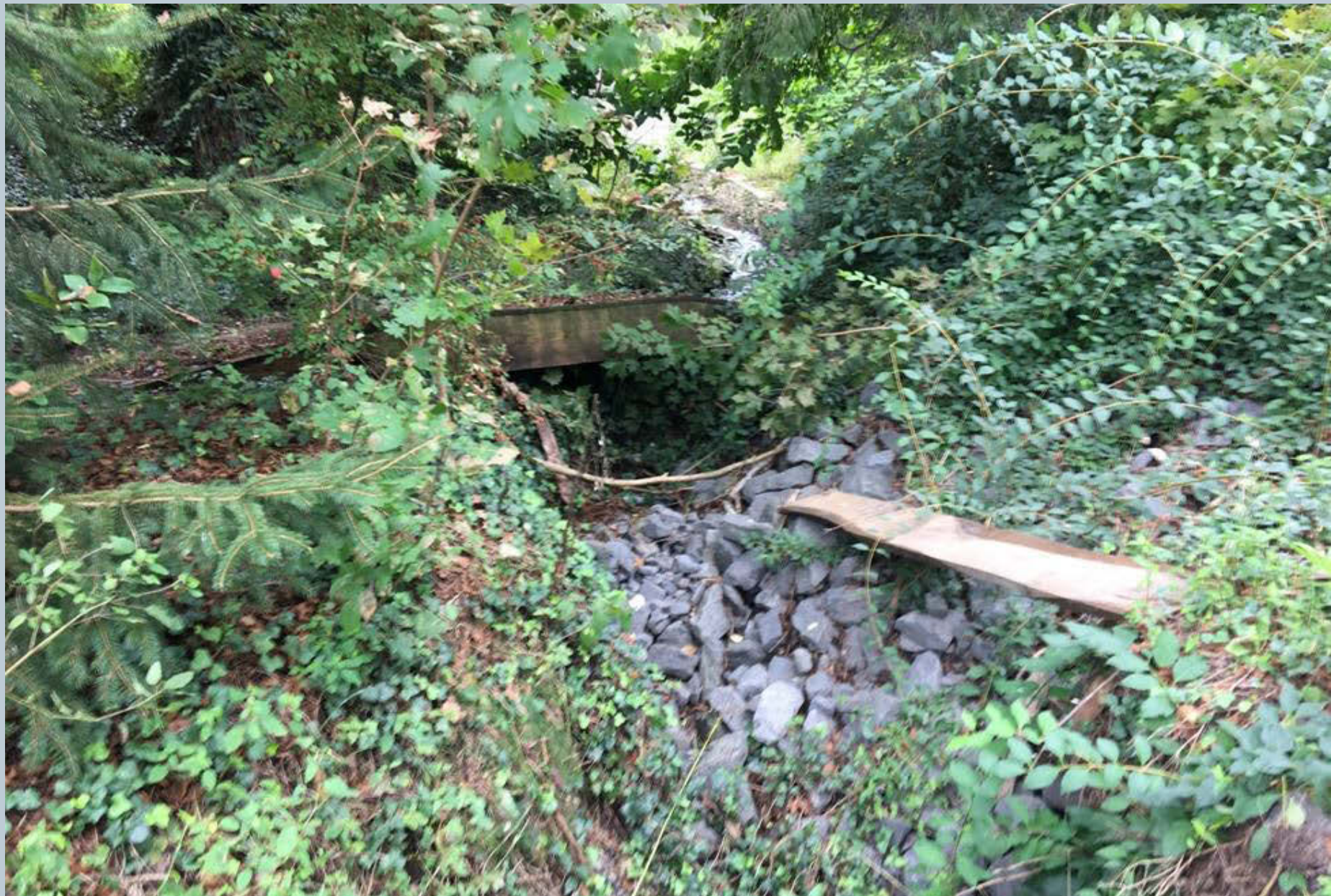
Figure 63. A collapsed area on the upstream end of another unnamed tributary to Toby Creek off Pioneer Avenue and Overbrook Road.
