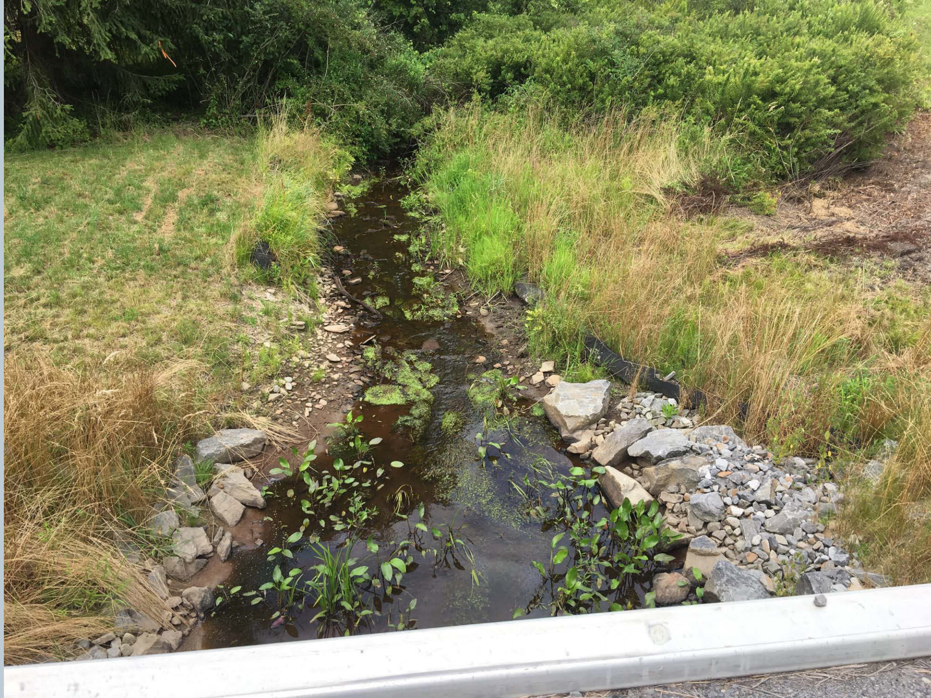
Figure 224. An unnamed tributary to Toby Creek looking upstream of the bridge on Hildebrandt Road with some rock armoring along the wingwalls and native riparian plants along the banks of the tributary and some remnant erosion control filter socks.
