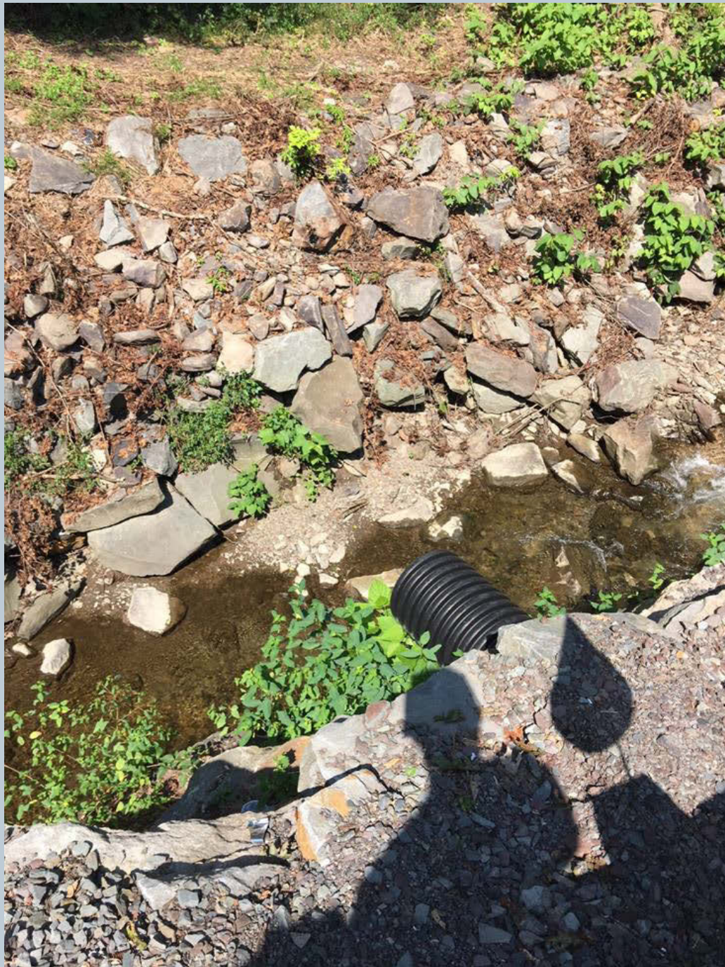
Figure 160. A shot of a black HDPE pipe sticking out from the retaining wall that drains a stormwater from the parking lot.
