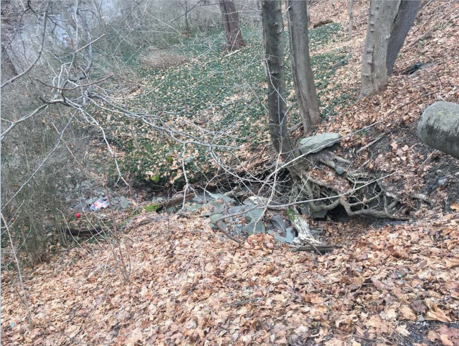
Figure 86. A shot of the severe drop from the storm drain outlet pipe. This has created a massive undercutting of the bank and stormwater channel all the way down to Toby Creek. A rip rap or large boulder step-pool reinforcement channel conveyance down to Toby Creek is needed to redirect stormwater downstream into Toby Creek rather than upstream.
