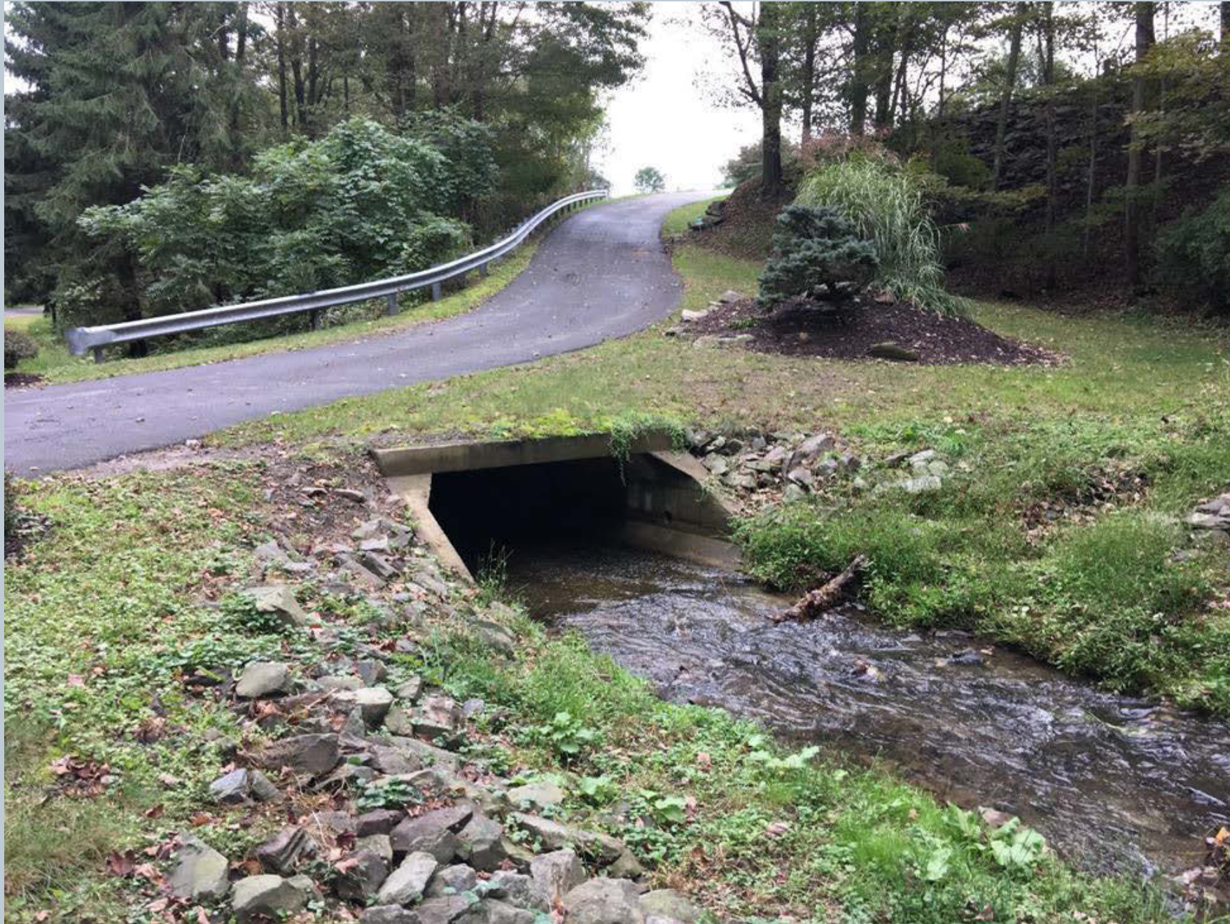
Figure 32. Looking downstream at the box culvert on the Green Pond unnamed tributary, located under the private driveway at 230 E. Center Street.
