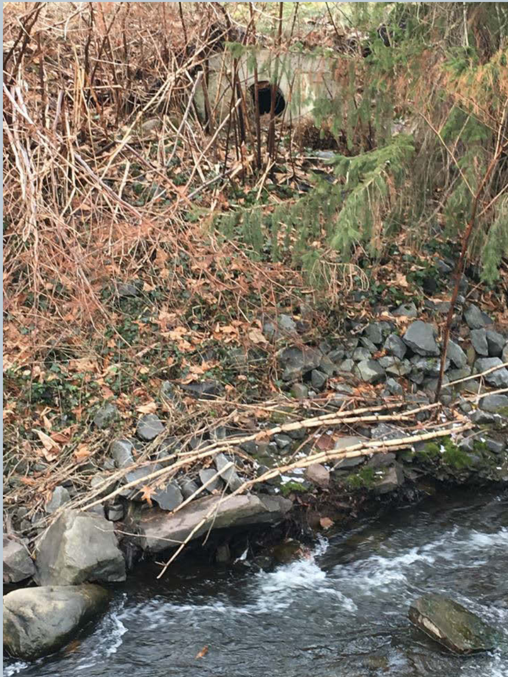
Figure 130. A 12-foot culvert from Kost Tire aligned along the left bank, looking upstream.
