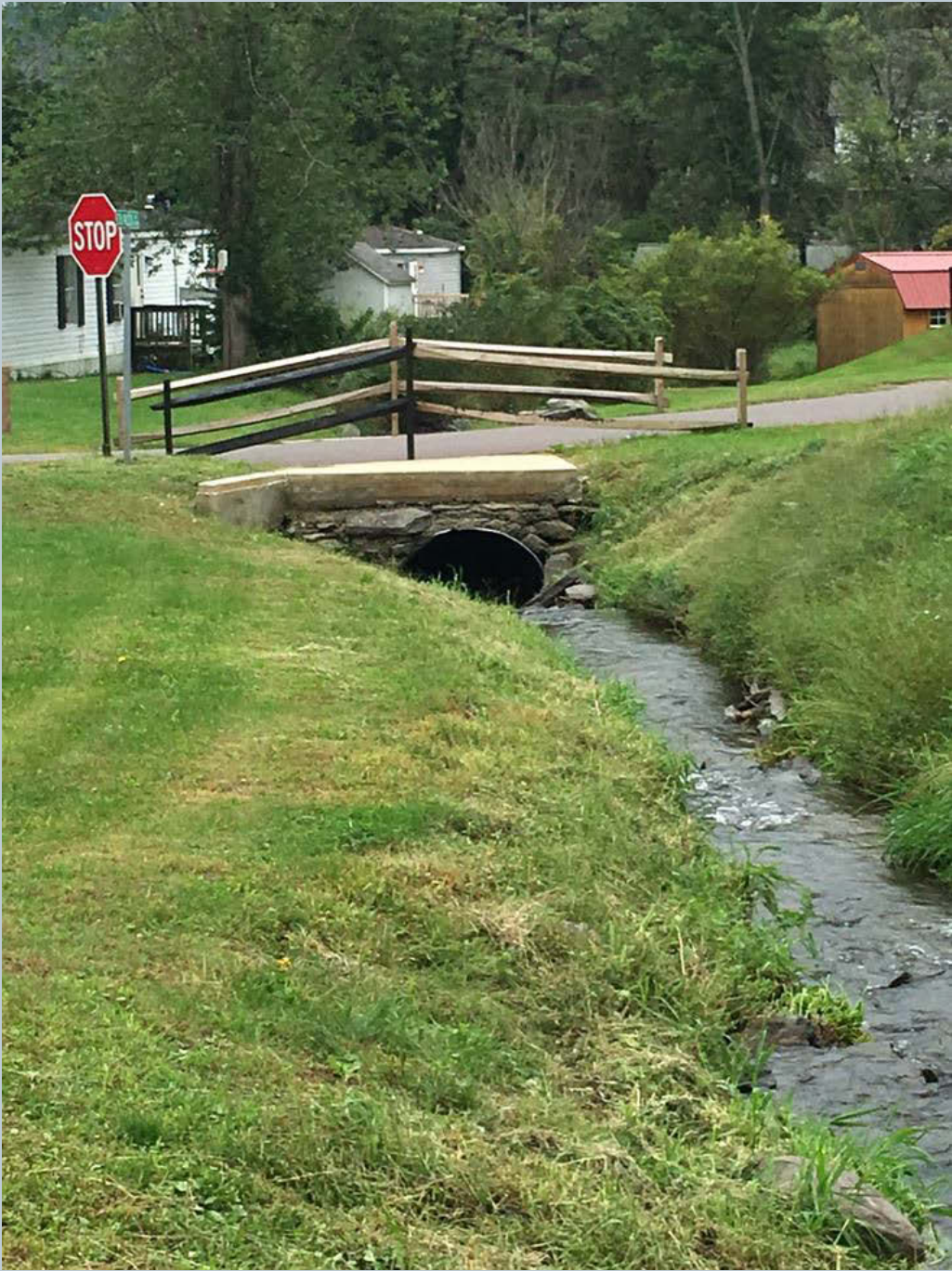
Figure 42. A shot looking downstream at a corrugated squash culvert pipe along Echo Valley Drive. This culvert is grouted and cemented with rock and rusted out completely at the bottom of the corrugated metal culvert pipe.
