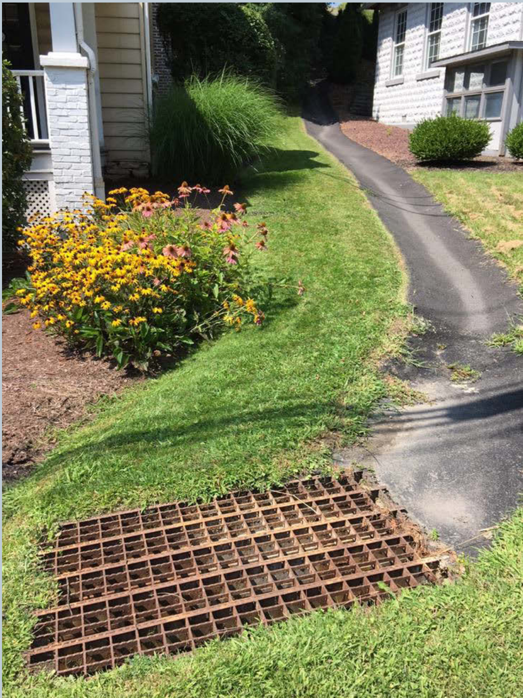
Figure 170. A shot of a macadam sluceway diversion taken from an upper parking lot area which is located between Berkshire Hathaway (Ted Poggi, Realtor) and the Church along Carverton Road, which enters a storm drain on the property before crossing Caverton Road.
