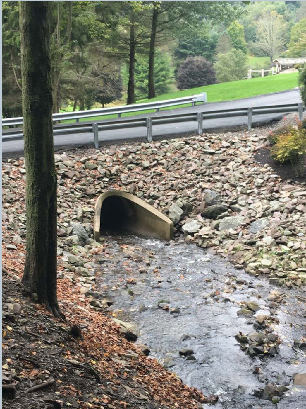
Figure 23. A shot of a concrete culvert under a private driveway that has a wide floodplain and a gravel bar deposit upstream. The driveway causes a rip-rap swale coming into the unnamed tributary.
