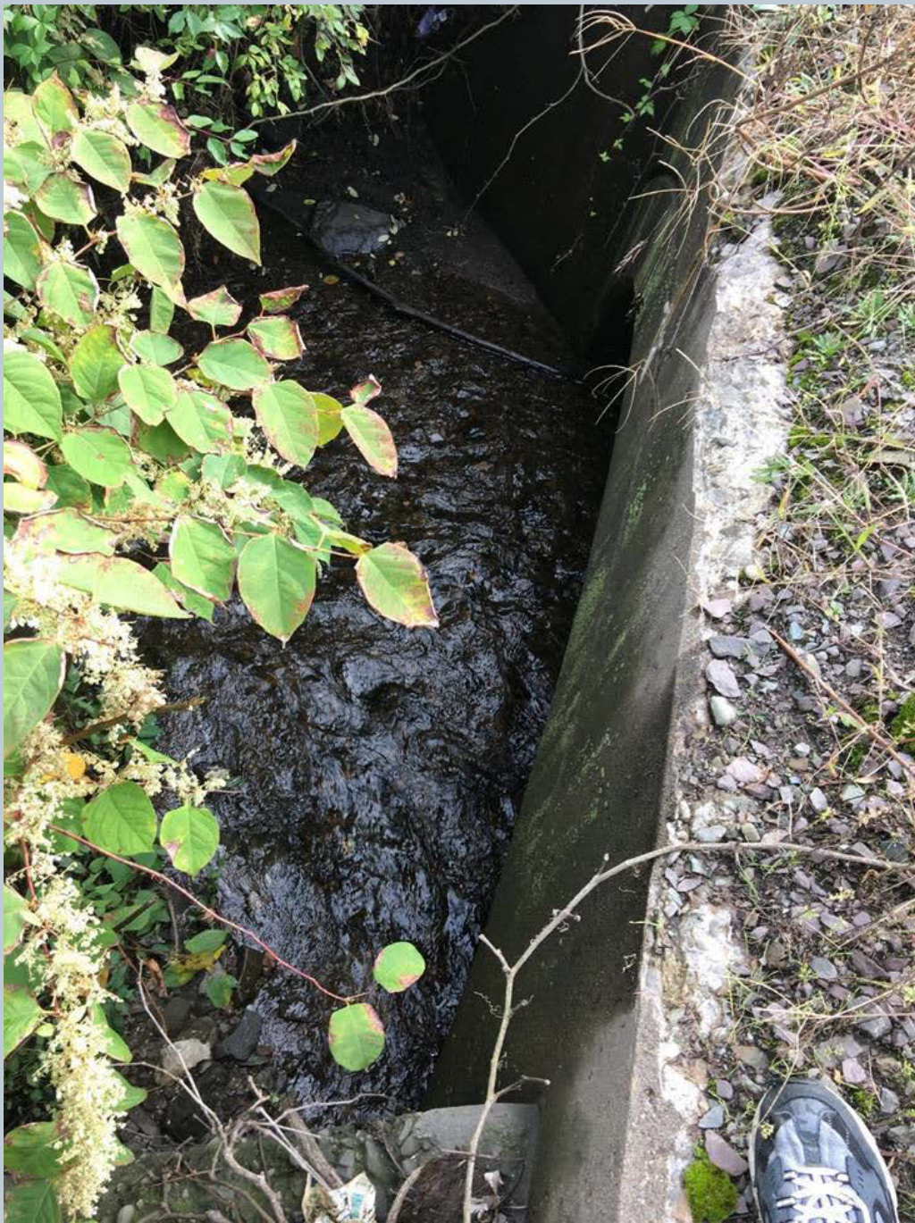
Figure 56. An unnamed tributary to Toby Creek behind Amelia's Diner. The unnamed tributary flows out of a much wider box culvert before reaching Toby Creek. This location is sediment-laden and has a presence of Japanese knotweed.
