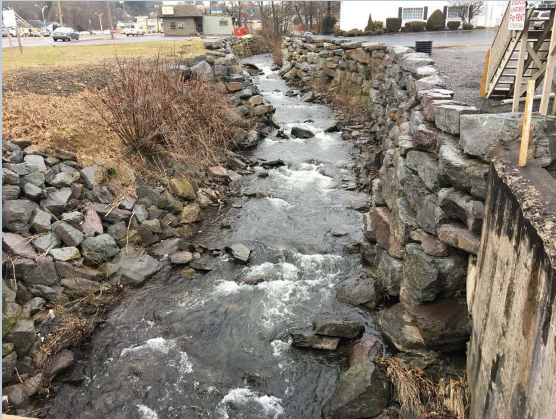
Figure 145. Looking upstream on Toby Creek from the W. Center Street bridge towards the Snowdon Funeral Home, this section of Toby Creek has a large historic streambank stabilization project that follows along both sides of the creek.
