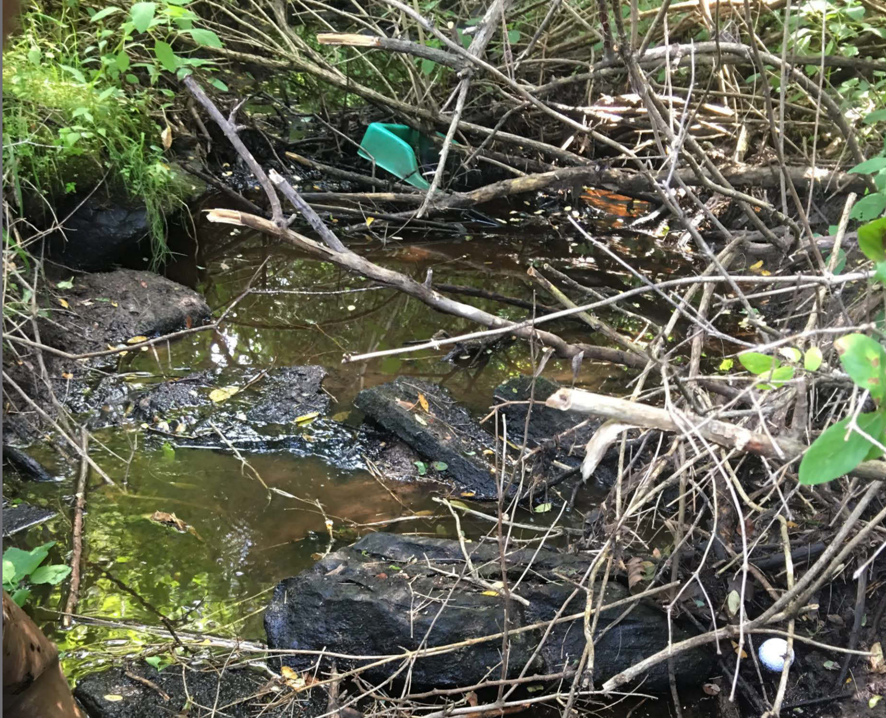
Figure 202. Looking upstream of culvert on unnamed tributary above Hole 4 on the Irem Golf Course. Litter is present and a small cleanup is recommended.
