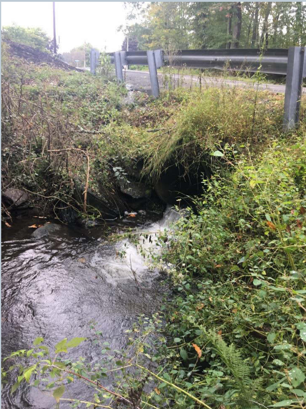
Figure 15. The concrete culvert has a 3-4-inch drop to the unnamed tributary, cascading into the downstream channel. A rock apron is recommended for aquatic connectivity and to prevent further scour from developing.
