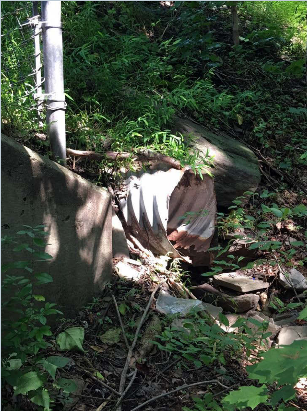
Figure 166. A rusted 18-inch corrugated pipe facing upstream. The pipe is not aligned when entering the UNT, creating a scour pool next to a large root wad from a tree along the streambank.
