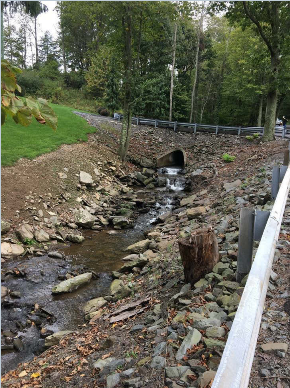
Figure 25. A log vane deflector or rip-rap are recommended, along with the removal of the rock check dam, to prevent further downcutting of the Green Pond unnamed tributary.
