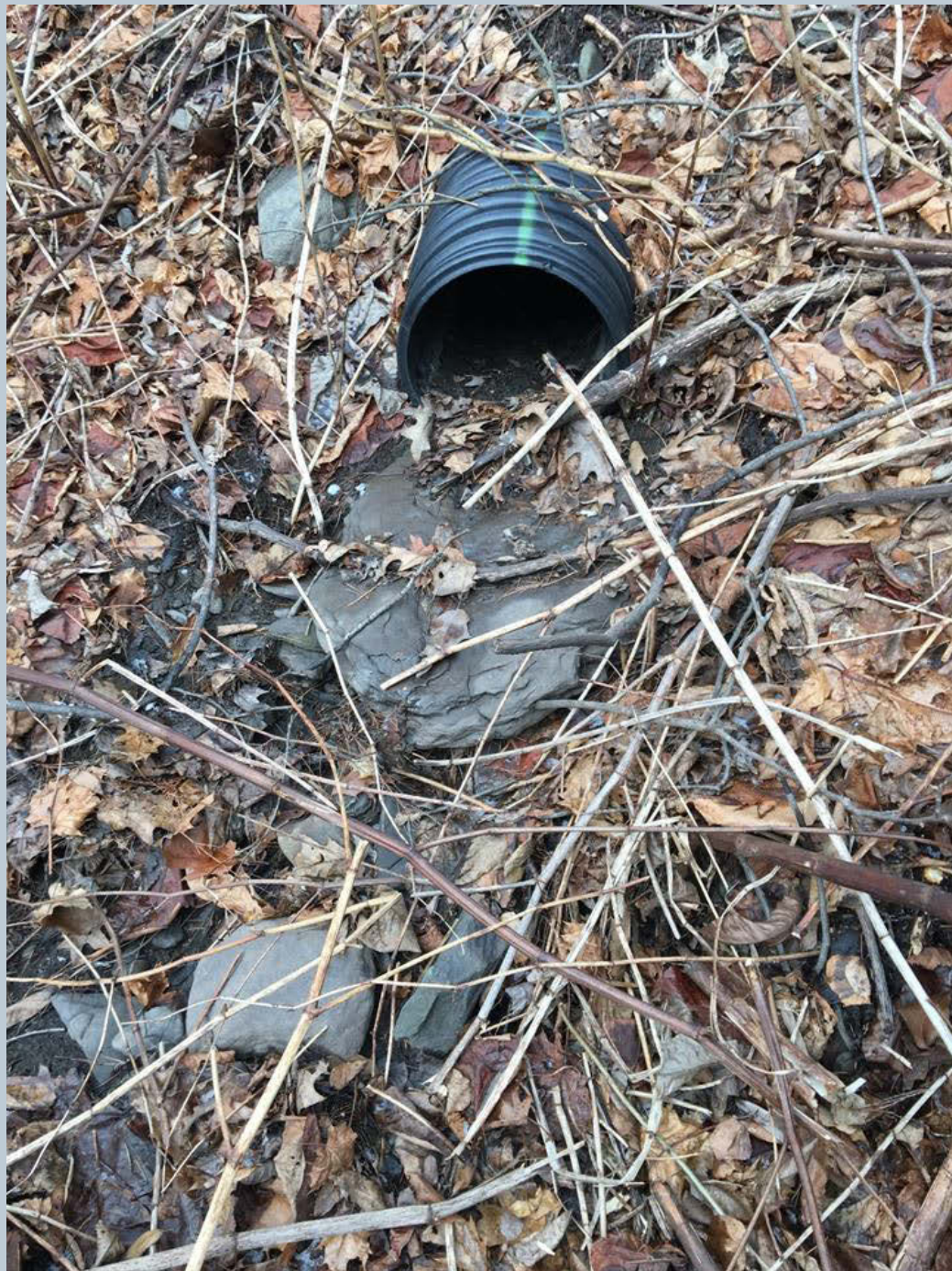
Figure 133. A 12-inch black HDPE stormwater pipe (dry) aligned with Toby Creek.
