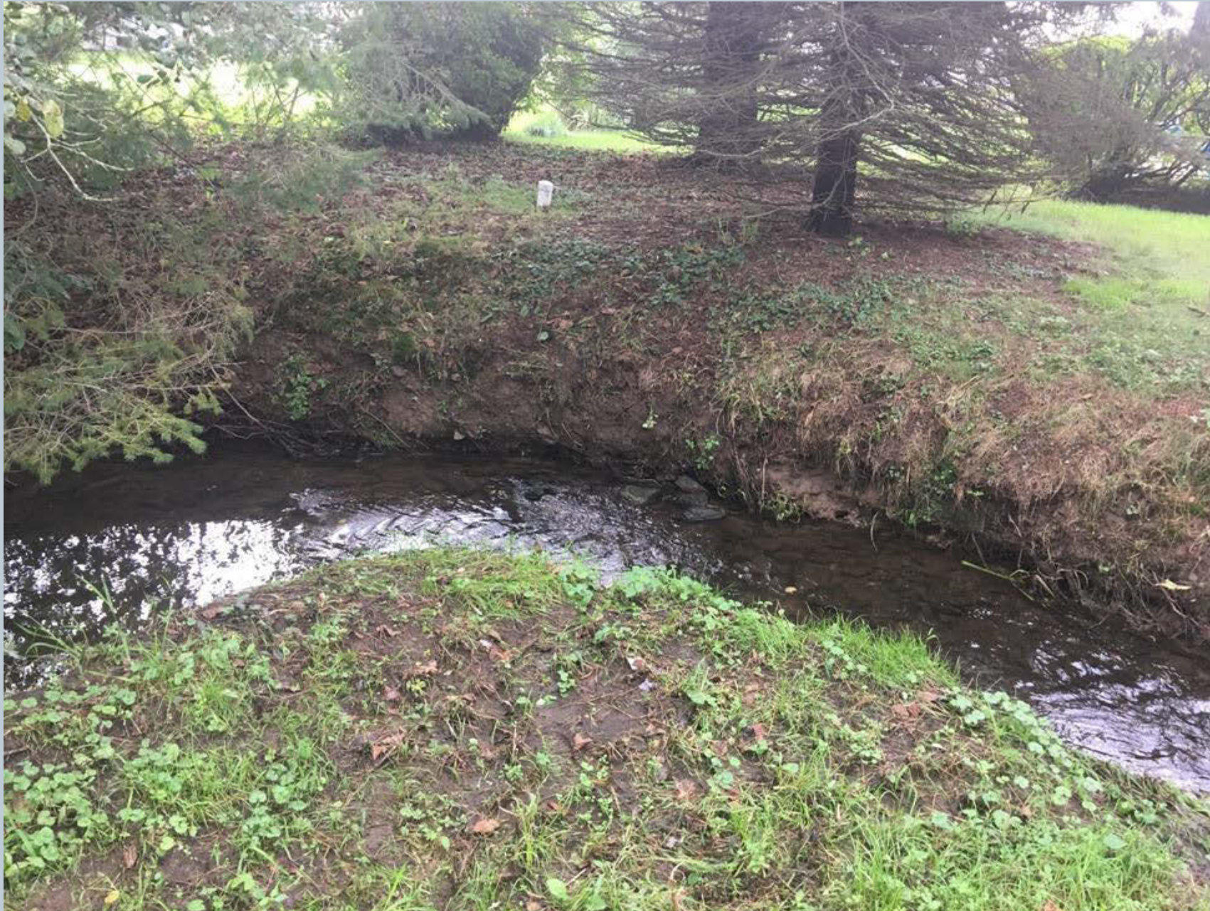
Figure 9. This photo shows 35 feet of potential streambank restoration planting behind 375 Woodbine Drive. White plastic pipes extended above the grade are suspected to be lateral cleanouts from the sewer or defunct water lines. Riparian restoration will require a utility mark out to be mindful of trees not impacting sewage flows from homes.
