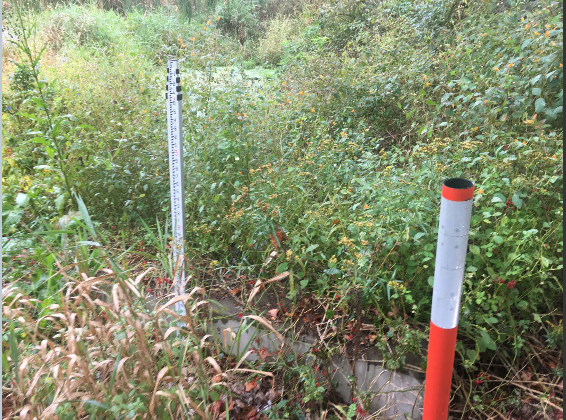
Figure 307. Looking upstream on stormwater forebay at the entrance to Windsor Farms development on an unnamed tributary to Toby Creek along Manor Drive.
