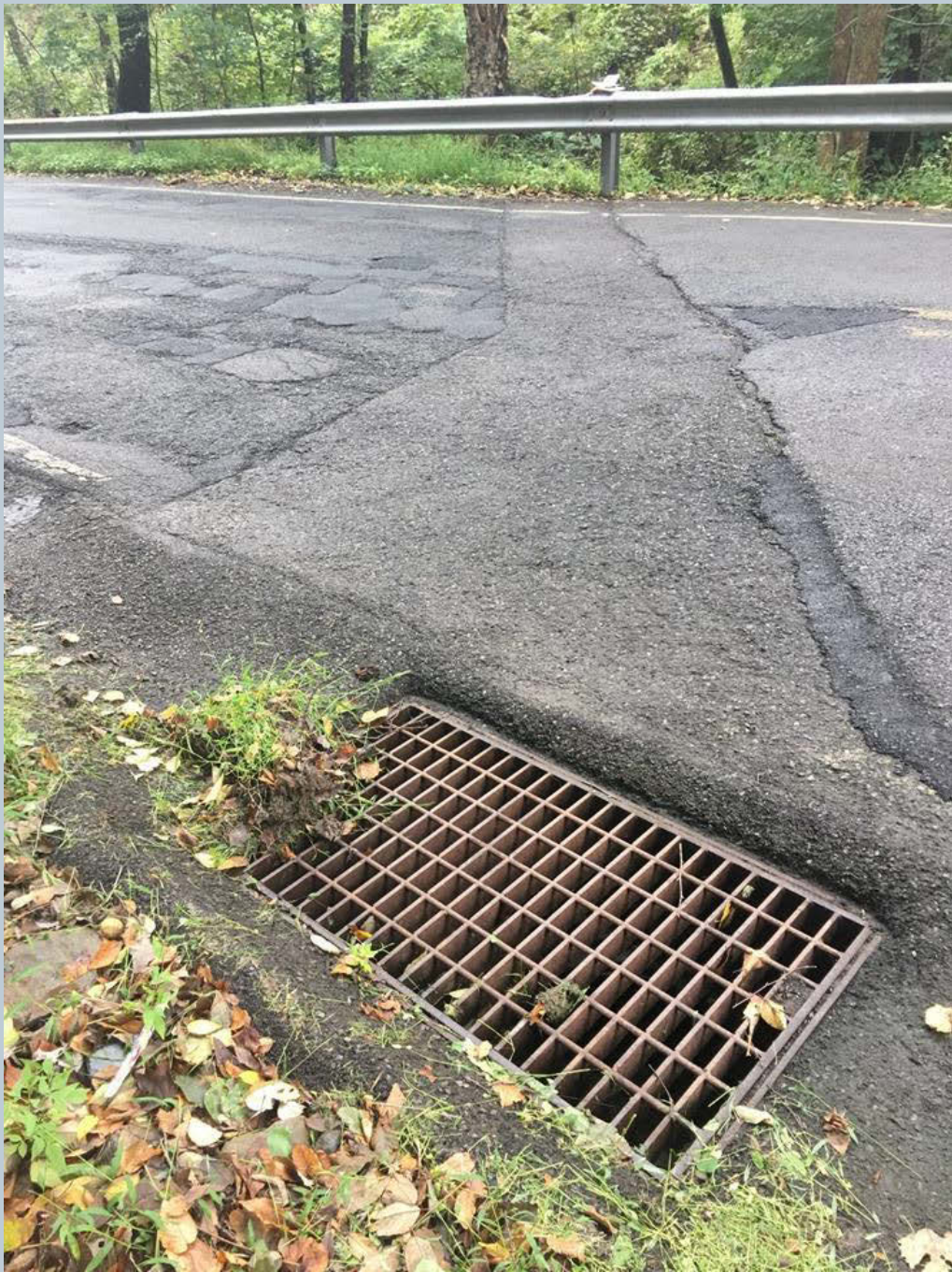
Figure 17. A storm drain on the opposite side of Harris Hill Road which drains to the Green Pond unnamed tributary.
