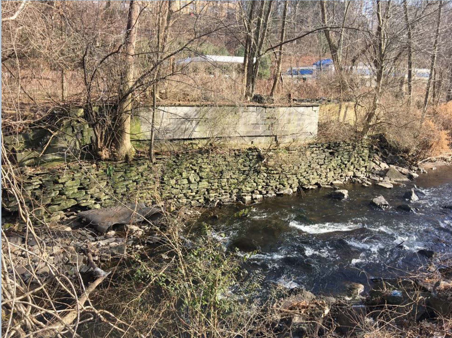
Figure 105. An old stone-stacked wall with a concrete block foundation is located above the floodplain bench and streambank. Upstream, where the wall has failed, there are gravel bar deposits. Near this location, just under a dozen tires have been illegally dumped. A small cleanup along this stretch of Toby Creek, along S. Main Street, would easily remove the tires.
