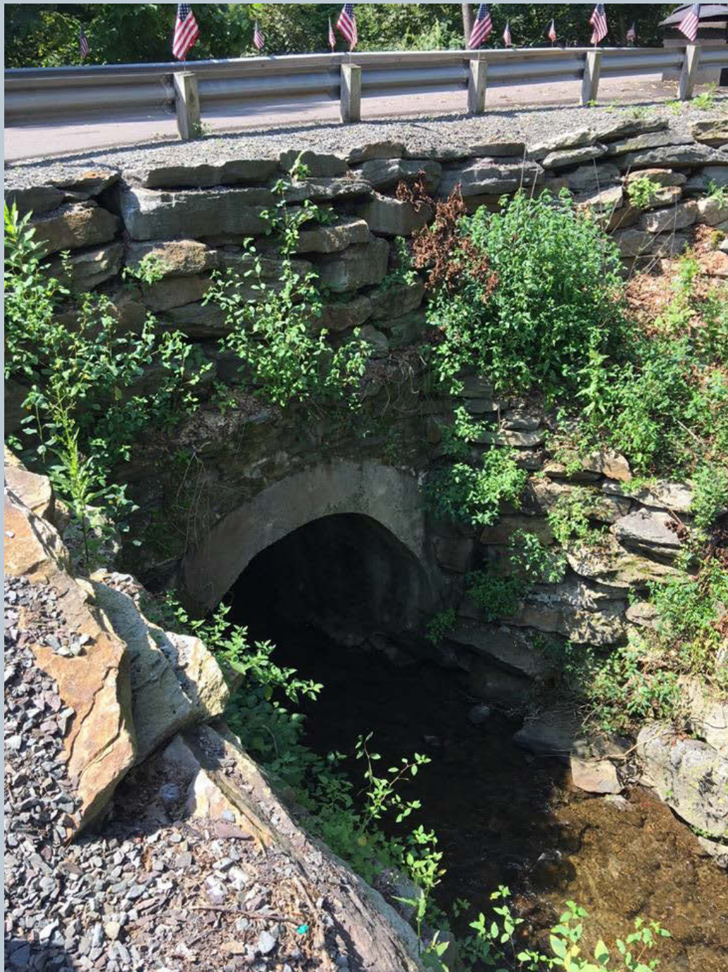
Figure 159. This photo is looking downstream at a stone arch that is over a concrete culvert. The culvert is on another UNT that flows along Carverton Road behind Pizza Perfect, in Trucksville. A hard armoring and rip-rap with a shot-crete and a quarry-cut retaining wall is found alongside of the northeastern side of the streambank, behind Pizza Perfect, and along the opposite bank from the meander to the stone arch culvert.
