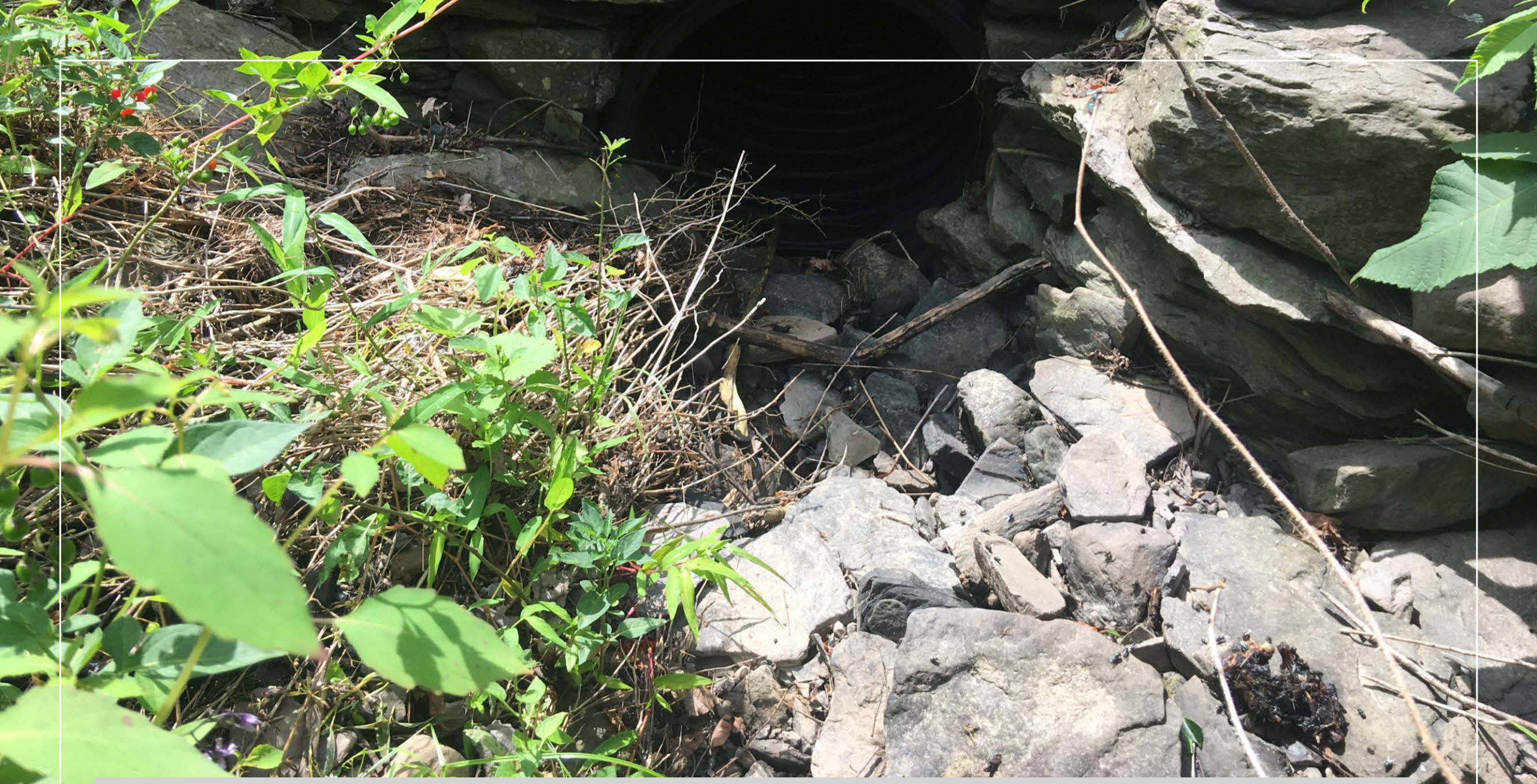
Figure 198. Ephemeral stream channel along the intersection of Country Club Road and Ridgeway Drive where the headwall is failing causing a cascading feature leading into the inlet of the culvert.
