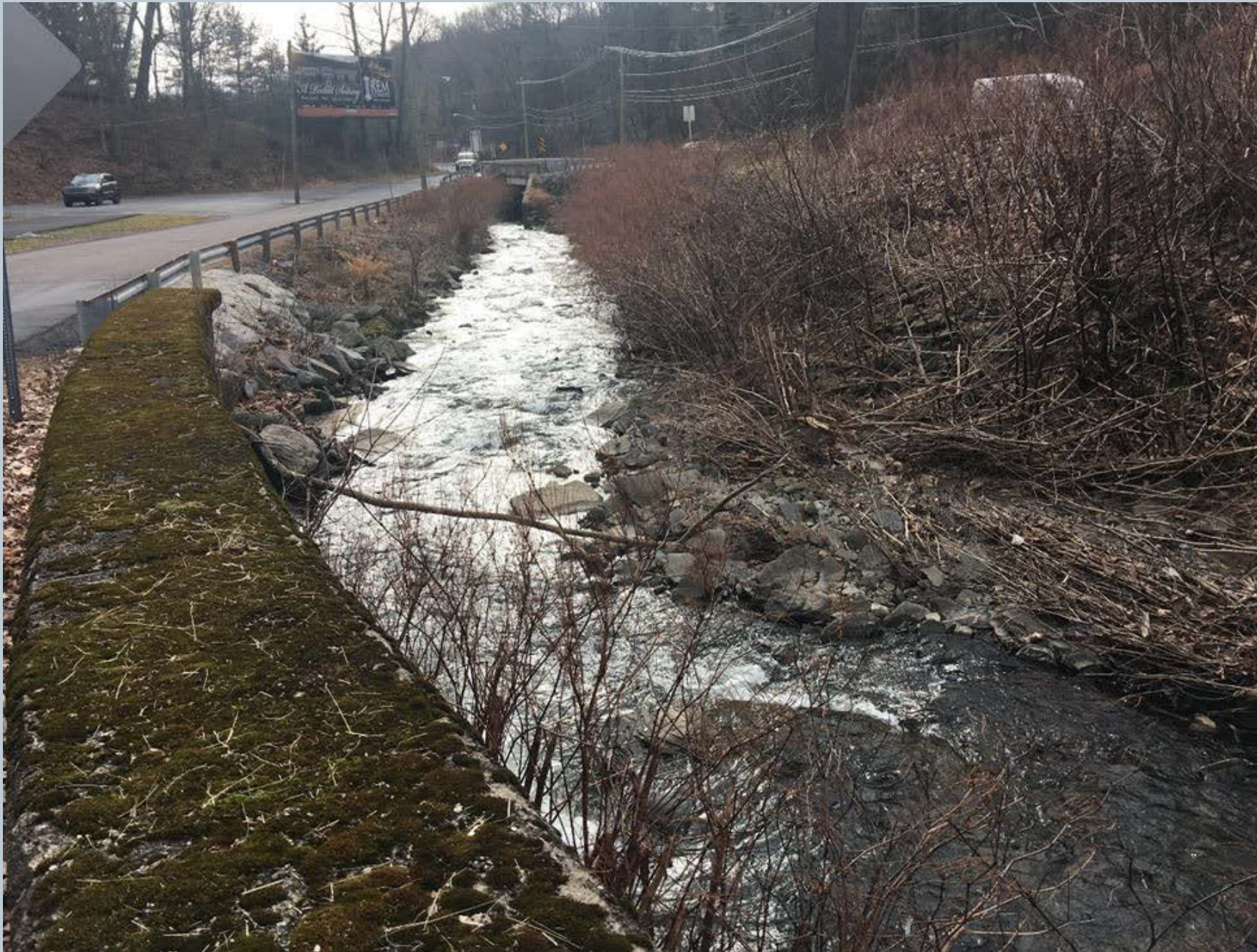
Figure 90. Looking downstream on Toby Creek from a curved concrete retaining wall along N. Main Street towards Plum Ave. This location has shotcrete rip rap along N. Main Street which is used to stabilize the streambank and protect the road from a historic undercutting that occurs just below the curved retaining wall on the left side of the bank.
