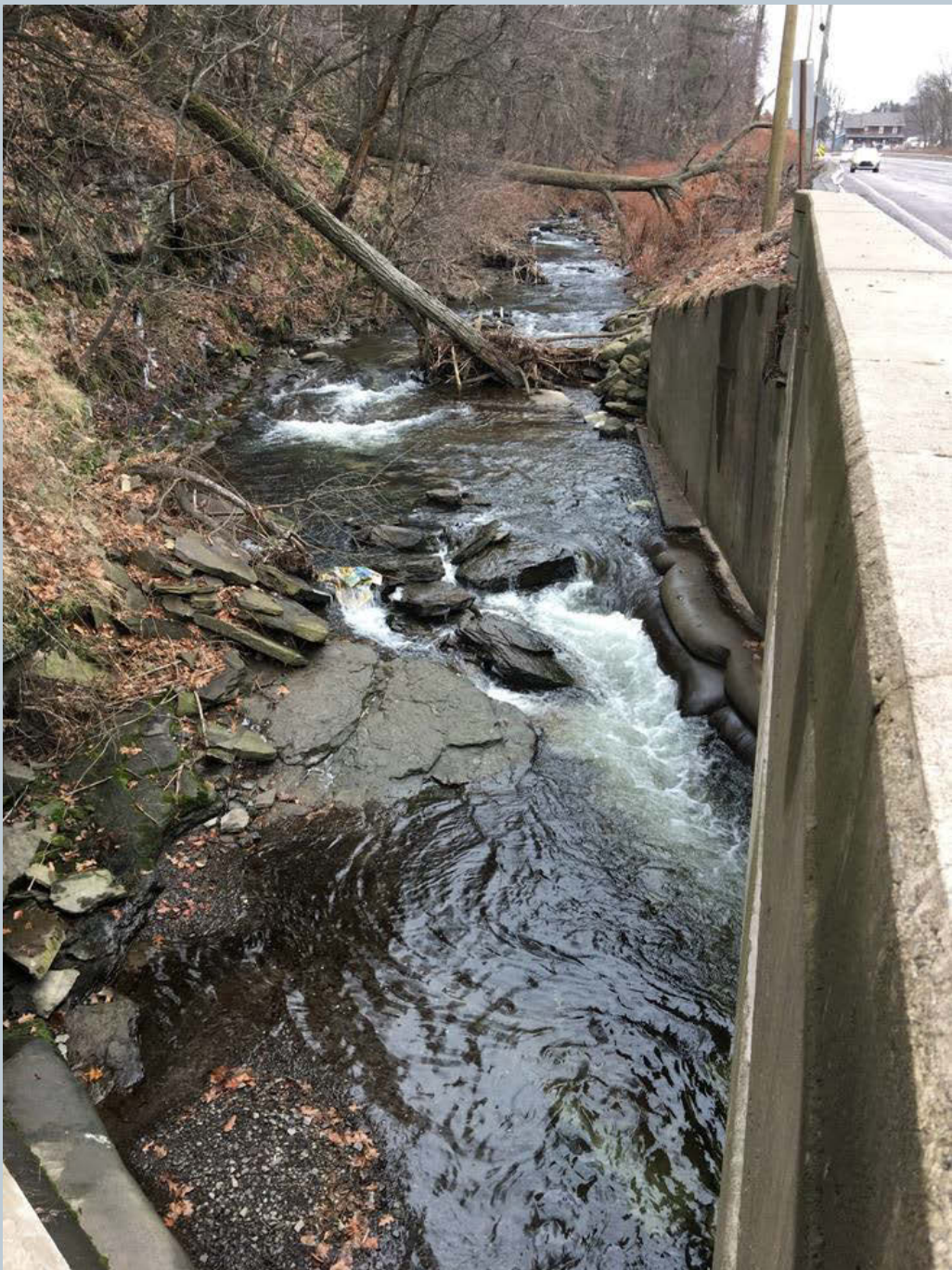
Figure 136. Looking upstream on Toby Creek, just north of the bridge over State Route 309, near the end of N. Main Street. This shot captures a large fallen tree that is angled into Toby Creek above the bridge, which raises future concerns. There has also been severe undercutting of the bedrock along the left wingwall abutment.
