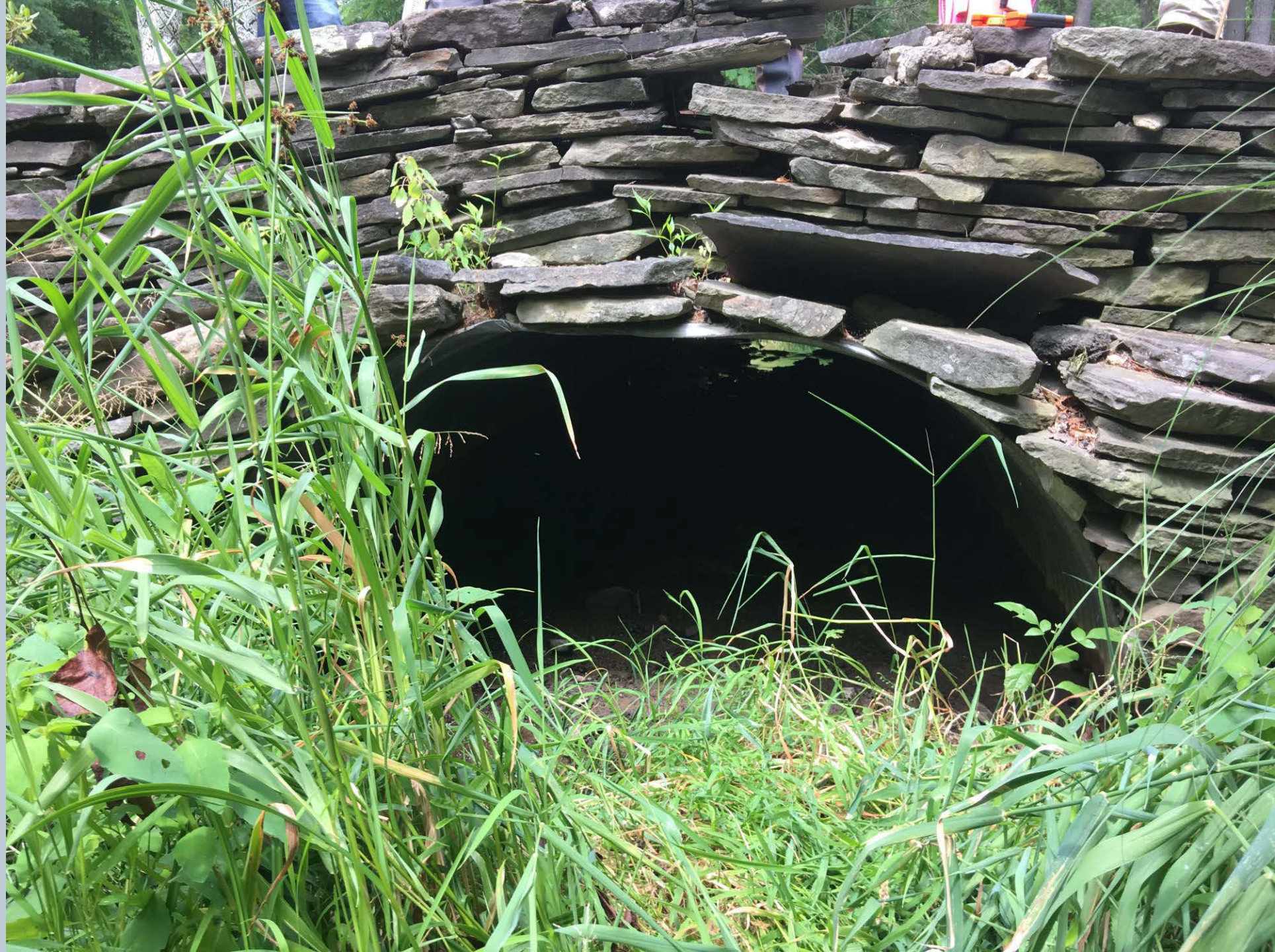
Figure 214. An unnamed tributary to Toby Creek looking upstream of the outlet corrugated metal pipe on Glenn Riddle Lane with an excellent landscaped riparian area.
