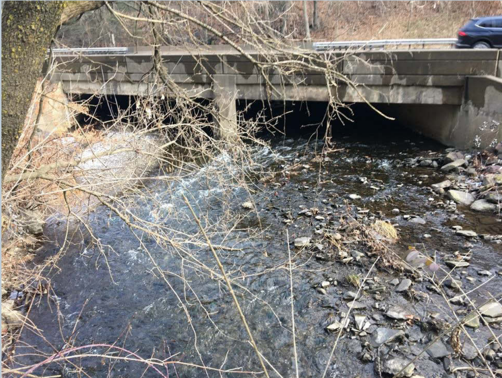
Figure 99. Taken looking upstream from S. Main Street along an old concrete retaining wall at a bend in Toby Creek. From just 50 feet below the double box culvert bridge running over State Route 309 (pictured), gravel and cobble deposition is seen in the left box, which carries about 30% of the flow. The right box carries the remaining 70% of the flow.
