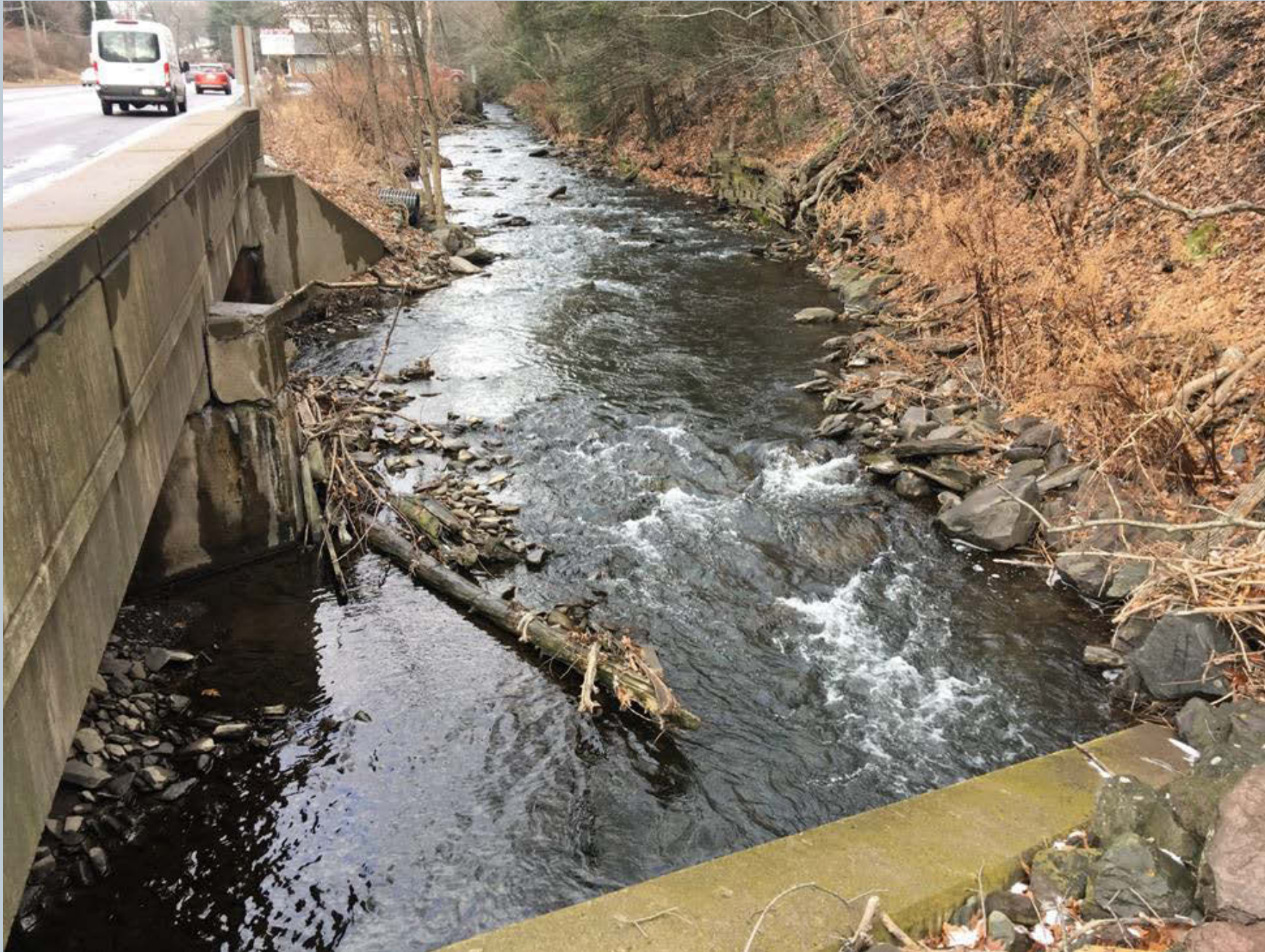
Figure 107. Looking upstream on Toby Creek from the double box culvert bridge over State Route 309, debris can be seen piled up against the middle abutment. 70% of the creek flows through the left box on the upstream side of the bridge.
