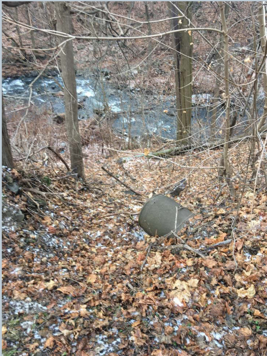
Figure 91. A dry 18-inch concrete stormwater outfall pipe structure located under Heller's Grove Road, sticking out over the steep bank that is aligned downstream with Toby Creek.
