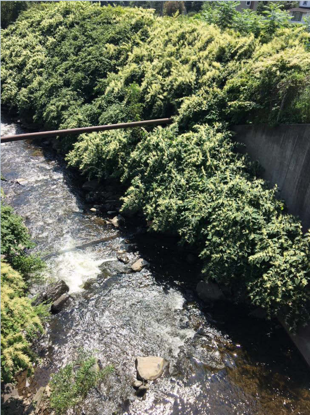
Figure 163. A shot of Toby Creek, looking downstream from a bridge at Carverton Road and State Route 309. A water or sewer line is secured overhead and above Toby Creek at approximately 20 feet. This line comes out of a retaining wall from the Trucksville Volunteer Fire and Rescue Company.
