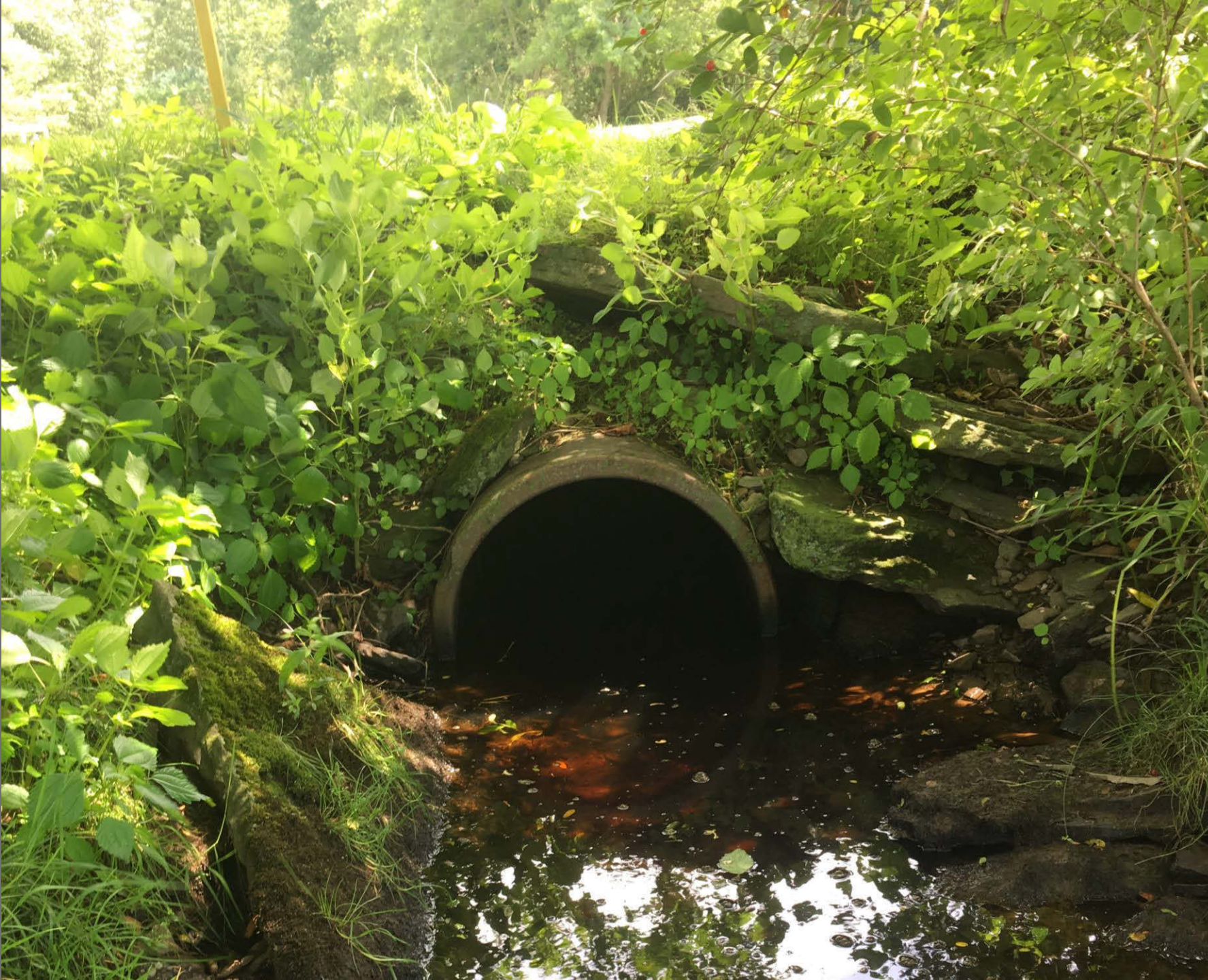
Figure 204. Outlet of concrete pipe on an unnamed tributary that extends across Hole 4 and is piped once beneath the fairway on the Irem Golf Course.
