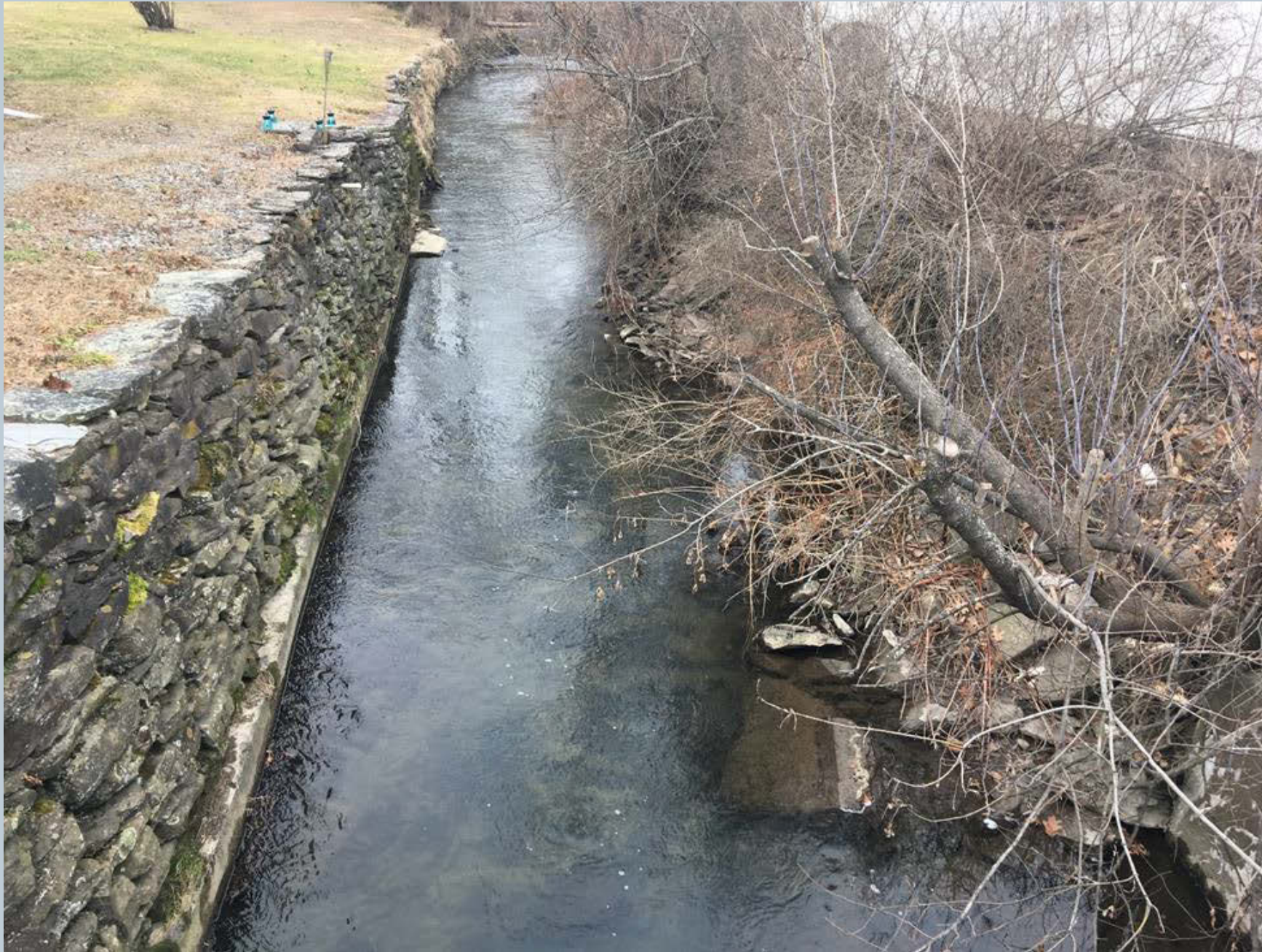
Figure 76. This location is looking upstream on Toby Creek, before it flows along N. Main Street and back into Dallas Borough, from the bridge over Lower Demunds Road. A large manmade stone-stacked retaining wall has been historically constructed along the left streambank looking upstream. The retaining wall has created a very straight morphology for the creek for several hundred feet.
