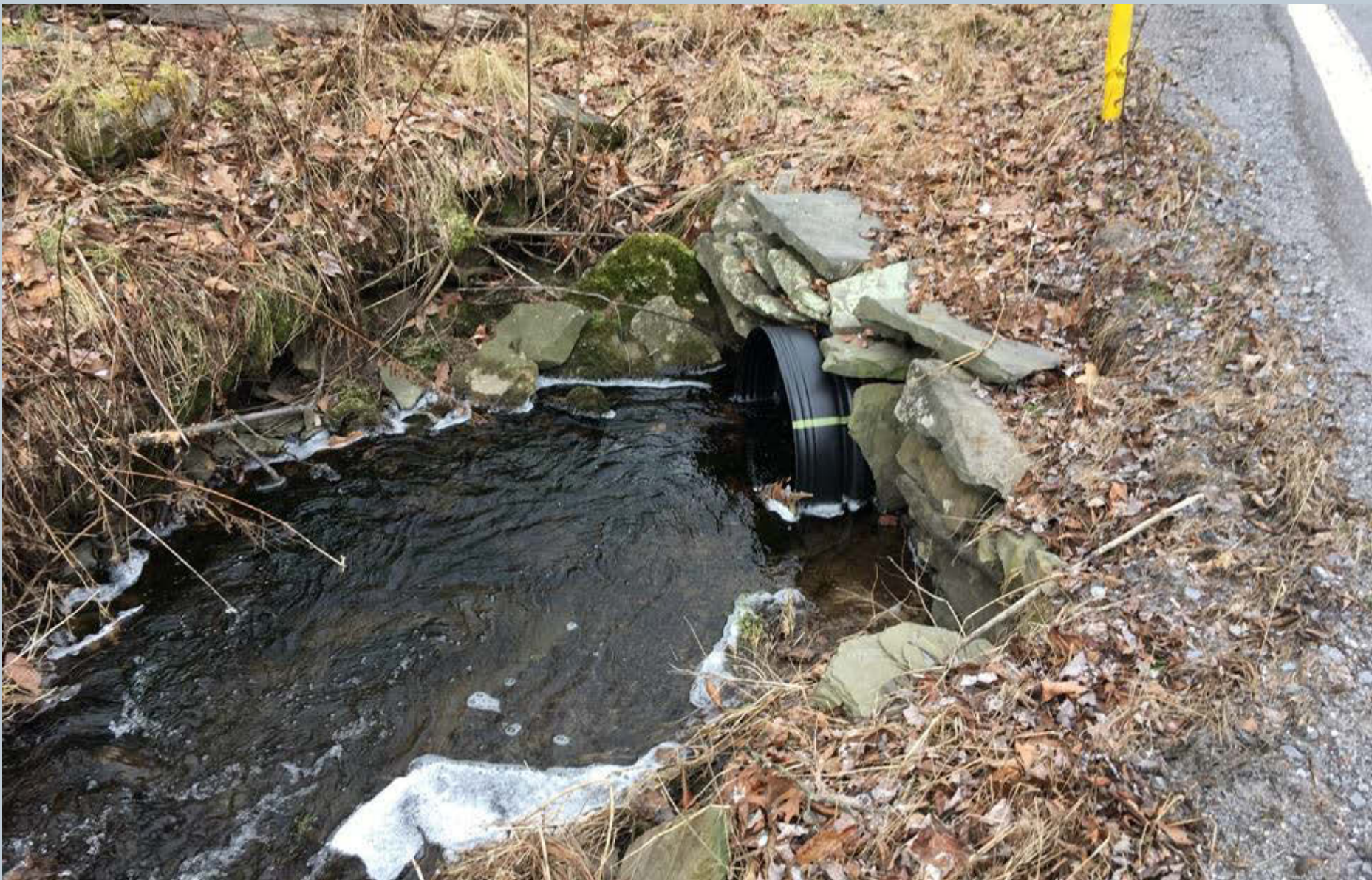
Figure 65. A shot of Trout Brook flowing through the black HDPE pipe culvert into a large forested wetland area that is located on private property. The culvert is not aligned beneath Lower Demunds Road.
