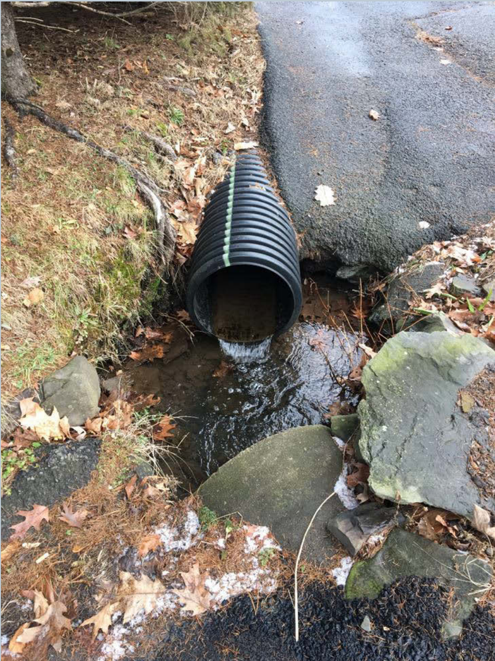
Figure 120. A shot of an 18-inch black HDPE pipe that is disconnected from another 18-inch concrete pipe at the corner of N. Main Street and Division Street, separated by a two-foot gap and drop that allows for roadside runoff. This runoff then enters the 18-inch concrete pipe that carries the stormwater and the UNT to Toby Creek.
