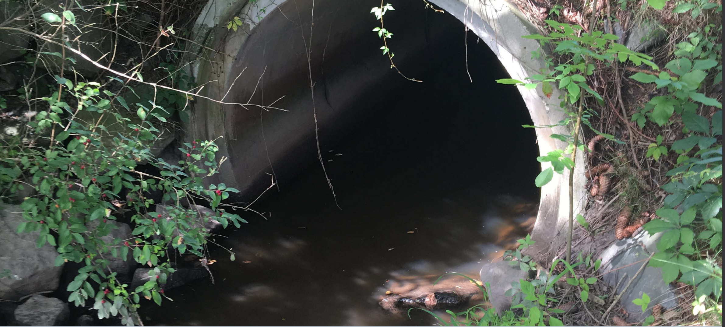
Figure 193. Inlet pipe at the dip in Irem Road at the bottom of the hill. Catfish were present. A severe constriction exists upstream and beneath the road to the other side of the golf course. Pipe is recommended to be replaced to a larger box culvert.
