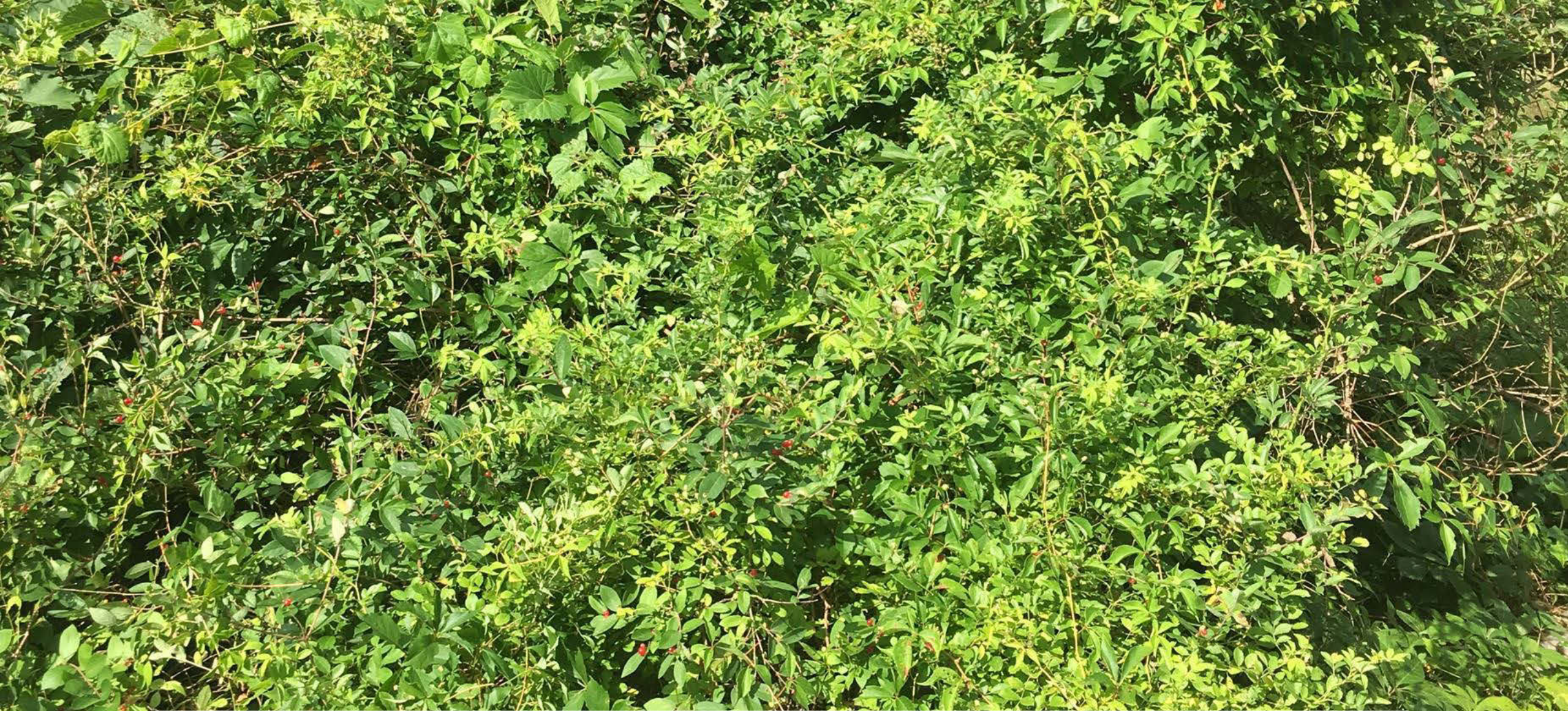
Figure 195. Downstream of culvert at the dip in Irem Road at the bottom of the hill. The herbaceous woody shrubbery has overgrown the outlet to the point it isn't even visible.
