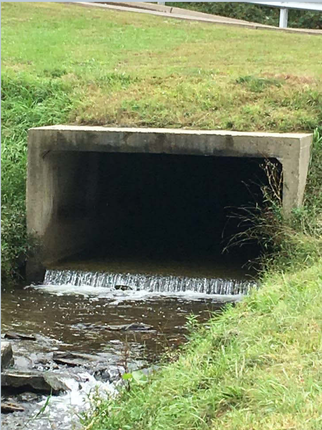
Figure 41. Looking upstream at the box culvert, this location cascades to the Green Pond unnamed tributary (around 3-inches). This location could use a rock apron for aquatic organism passage.
