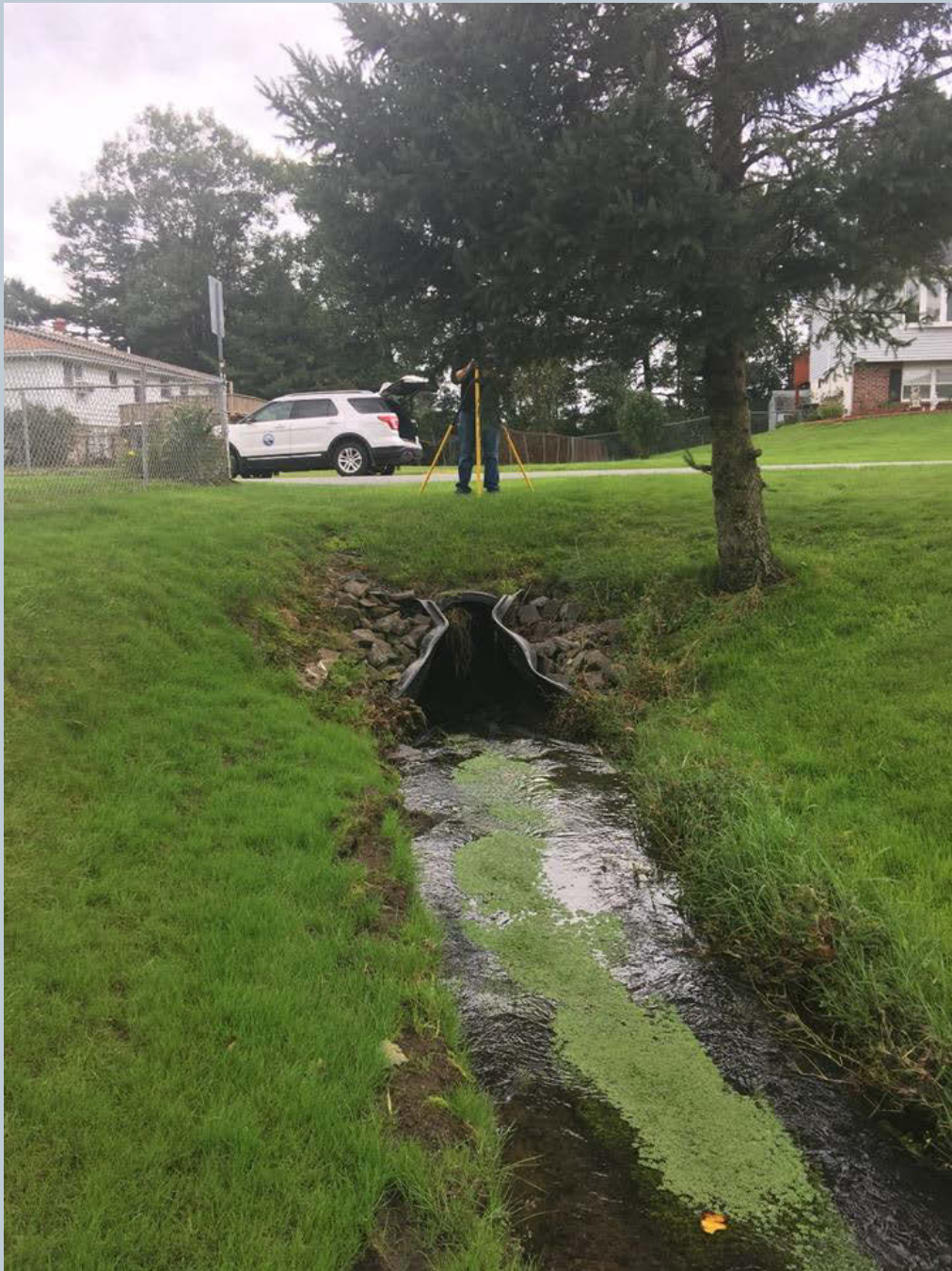
Figure 11a. Looking downstream at the Green Pond unnamed tributary duckweed, sediment, and pipe constriction are present.
