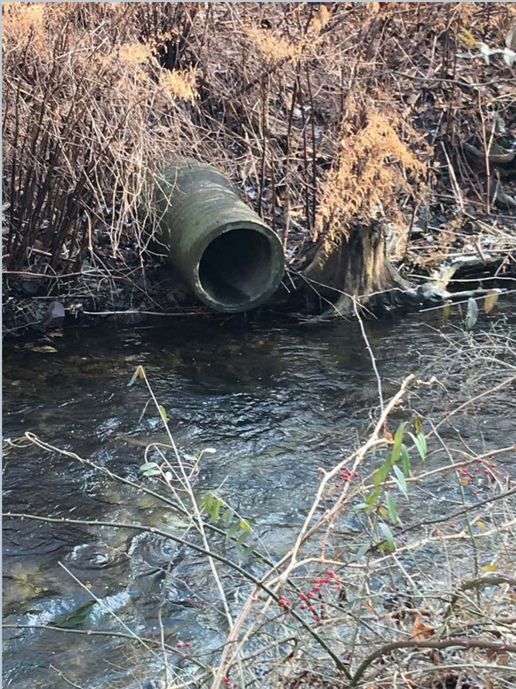
Figure 101. A dry 24-inch concrete stormwater pipe structure. The pipe runs perpendicular to Toby Creek, and is not aligned with the creek.
