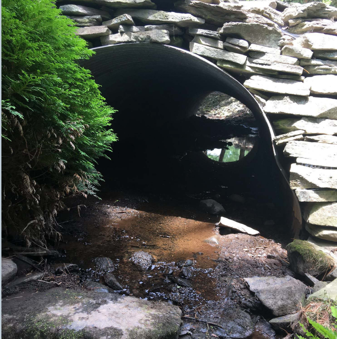
Figure 217. An unnamed tributary to Toby Creek looking upstream of the outlet corrugated metal pipe on Sunny Brook Lane. The pipe is full of sediment and is slightly rusted out.
