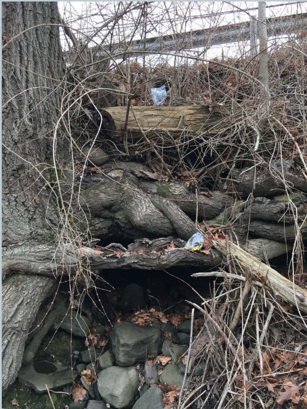
Figure 129. An old 12-foot concrete pipe (dry) for stormwater runoff from Shaver Avenue directed over a steep embankment, down to N. Main Avenue.
