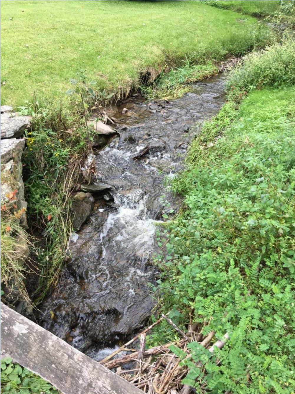
Figure 50. A photo looking upstream on the unnamed tributary to Toby Creek off Ferguson Avenue. Minor streambank erosion and undercutting are present.
