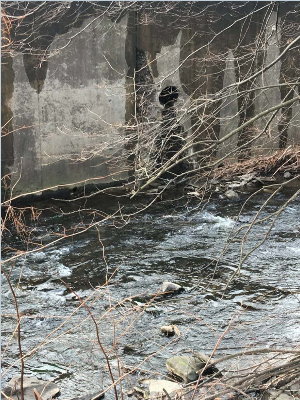
Figure 119. An UNT to Toby Creek flows from the middle of the concrete retaining wall (pictured) along N. Main Street and Division Street.
