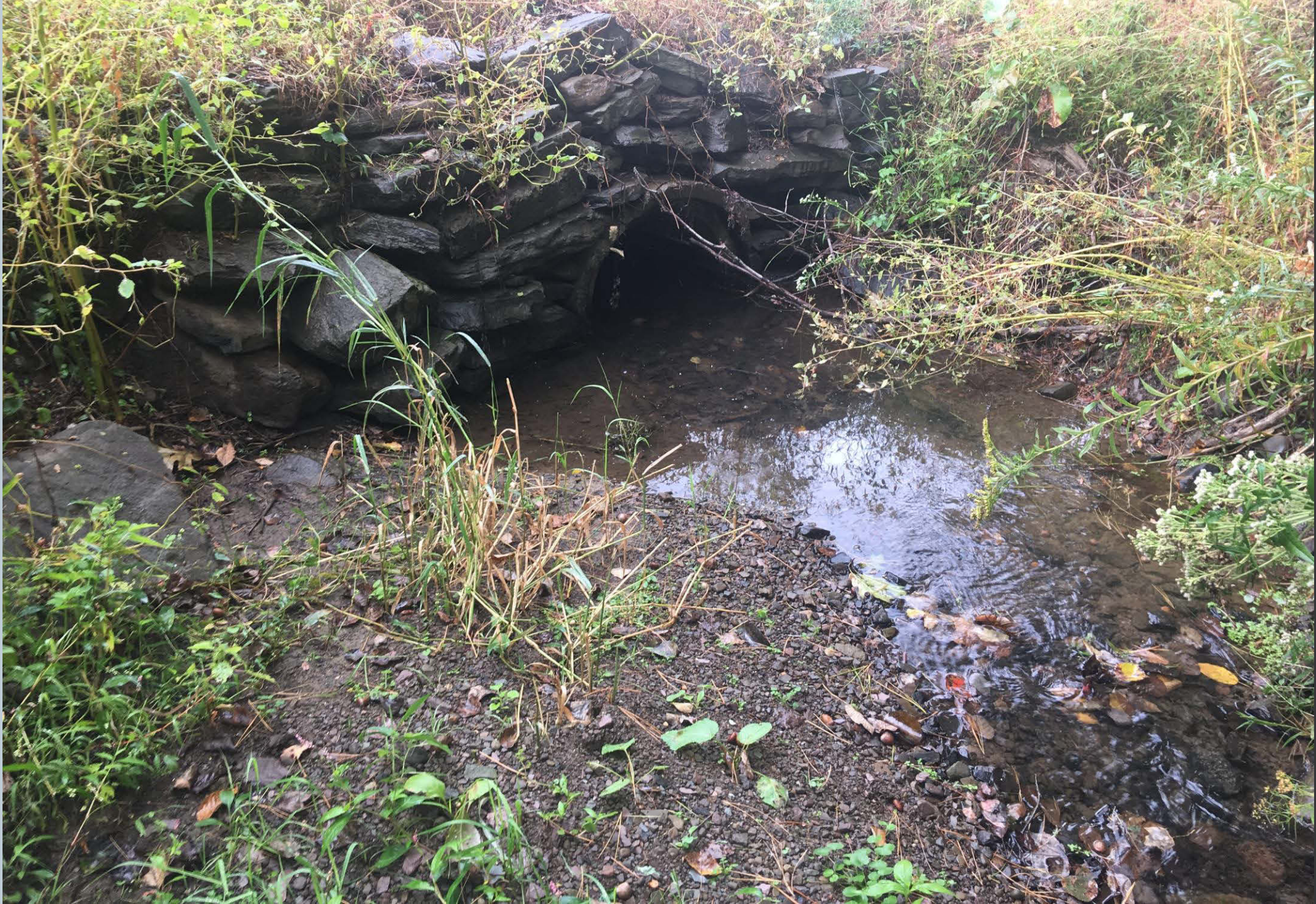
Figure 323. Looking downstream of the culvert inlet along Dug Road where a sediment gravel bar is present and a scour pool created by the two stormwater conveyances that come off of both hillsides along Dug Road in both directions to this low lying area. Fish present.
