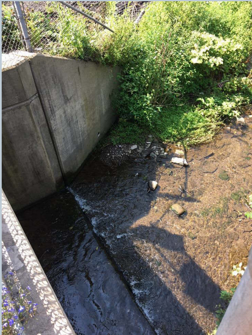
Figure 164. A shot of an UNT looking upstream along Carverton Road from the small bridge near Pizza Perfect.
