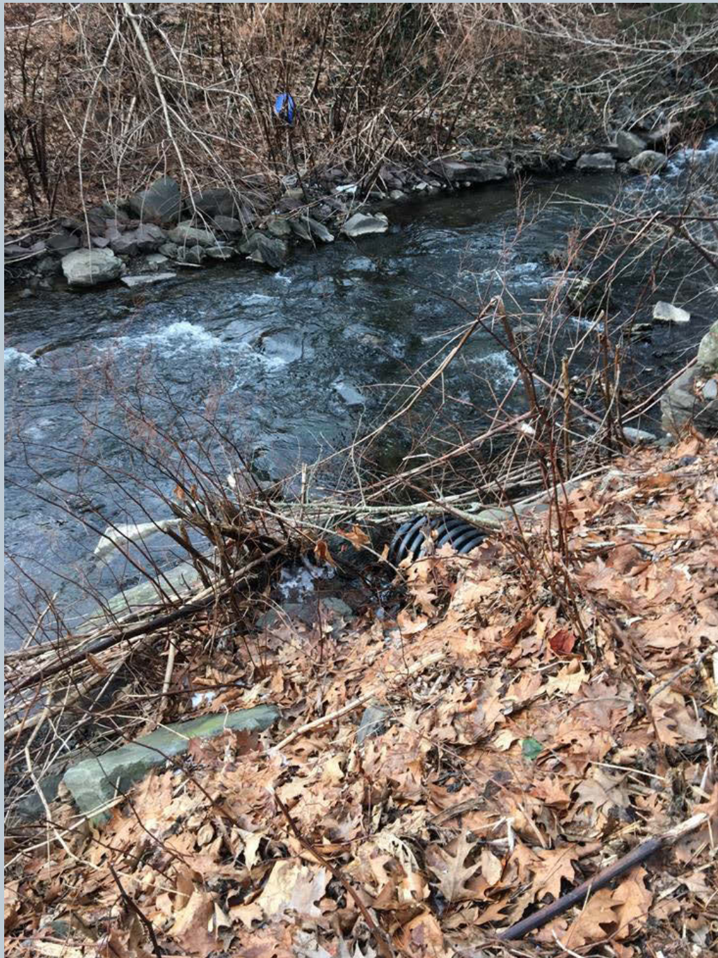
Figure 127. A 24-inch black HDPE pipe (flowing) that is not aligned, carrying an UNT across N. Main Street, perpendicular to Toby Creek.
