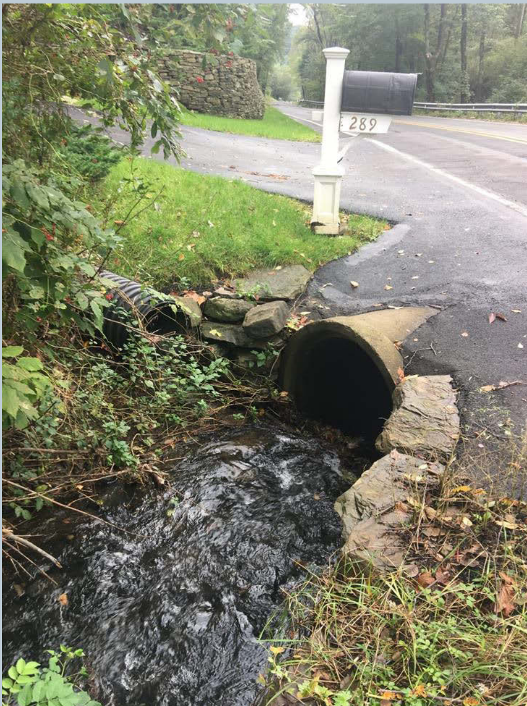
Figure 14. The Green Pond unnamed tributary concrete culvert pipe crosses the road heading downstream at 289 Harris Hill Road. There is an 18-inch black HDPE pipe to the left of the unnamed tributary, adjacent to the driveway.
