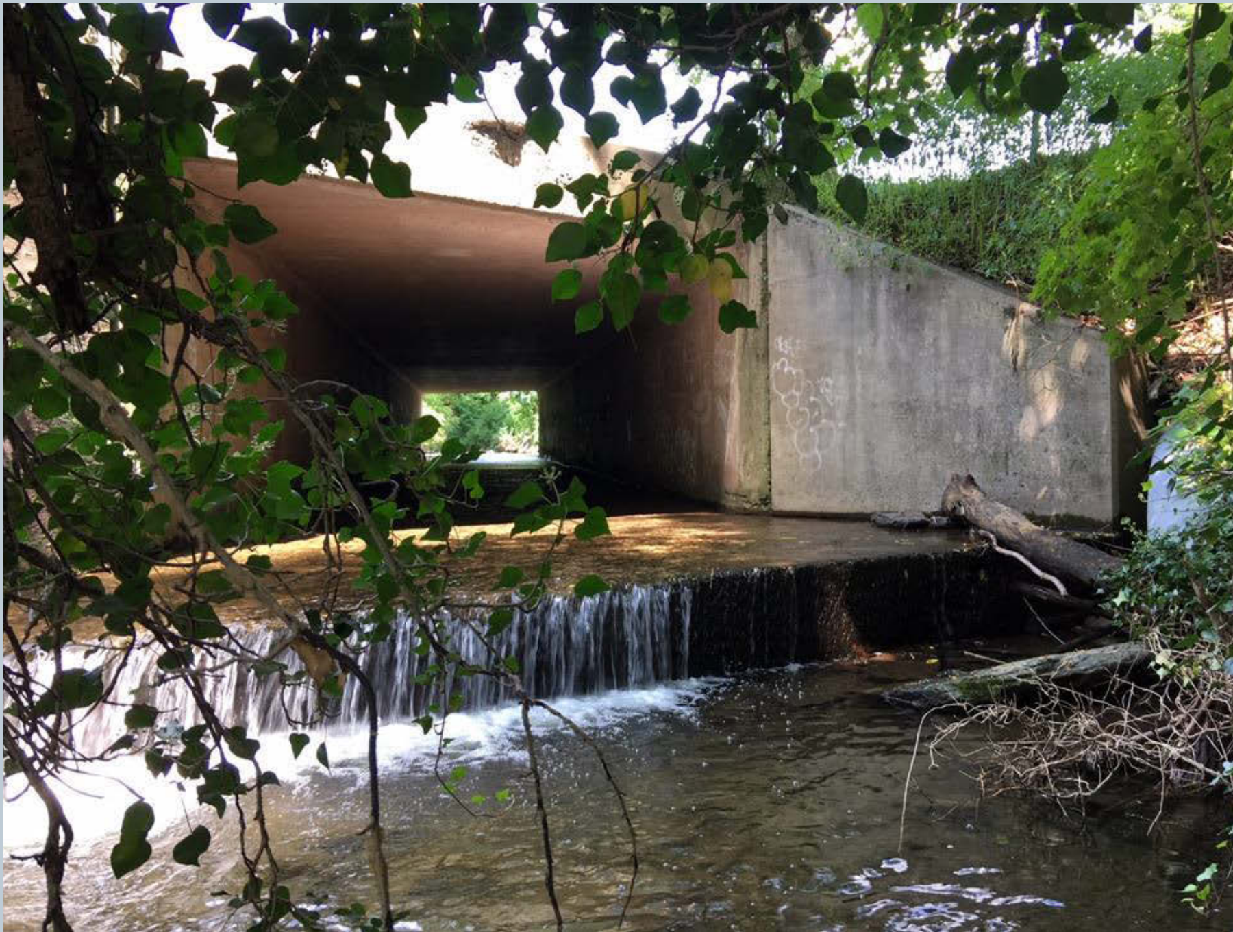
Figure 168. A shot of a two-foot concrete dam located below the bridge that is over the UNT to Toby Creek. An 18-inch corrugated metal pipe that enters the UNT from the northwesterly direction along the right bank, looking upstream. It is currently undetermined if the concrete dam is in an encased sewer line.
