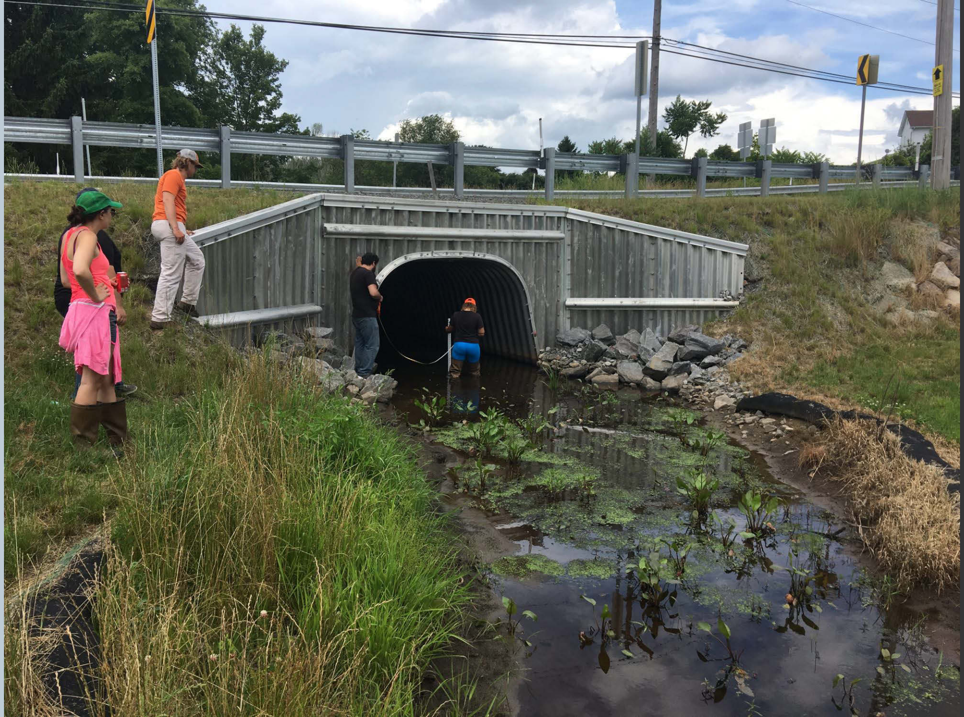
Figure 226. An unnamed tributary to Toby Creek looking upstream towards the bridge on Hildebrandt Road with some rock armoring along the wingwalls and native riparian plants along the banks of the tributary and some remnant erosion control filter socks.
