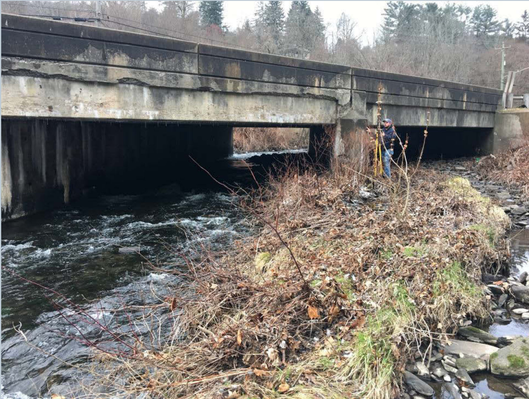
Figure 96. A shot looking upstream on Toby Creek at a double box culvert bridge on State Route 309. 100% of the flow is contained beneath the left box and no flow was present in the right box, 50% of the left box contained cobble, and 100% of the right box contained cobble.
