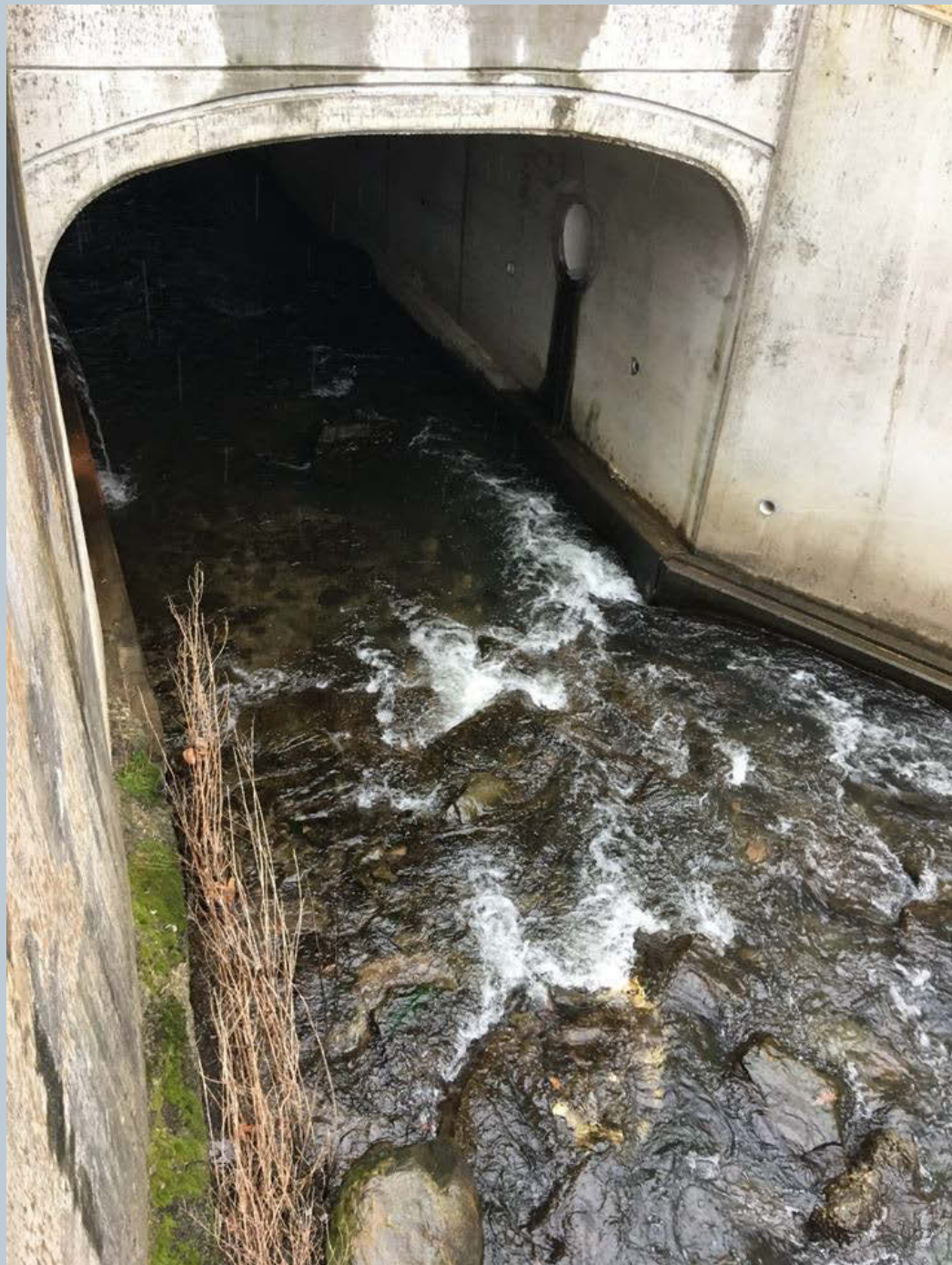
Figure 146. Beneath the W. Center Street Bridge there is an UNT that enters Toby Creek through an outfall pipe structure on the left bank of the retaining wall while looking downstream.
