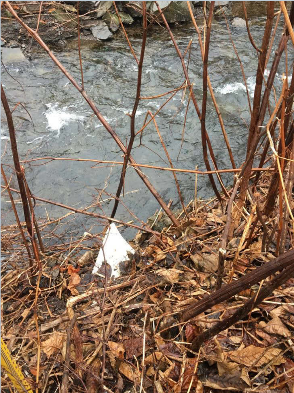
Figure 148. A 12-inch white PVC-like stormwater pipe, aligned with Toby Creek, is located two feet above the water level along an old retaining wall, located behind the clothing recycling bins near Cook's Pharmacy.
