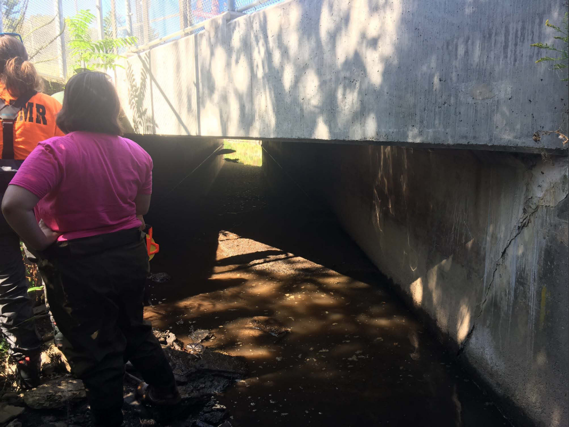
Figure 249. Culvert that directs Toby Creek from beneath Main Street, under the commercial district, until it outlets along Verve Vertu in Dallas. This is an open section before going into another culvert under the commercial district in Dallas.
