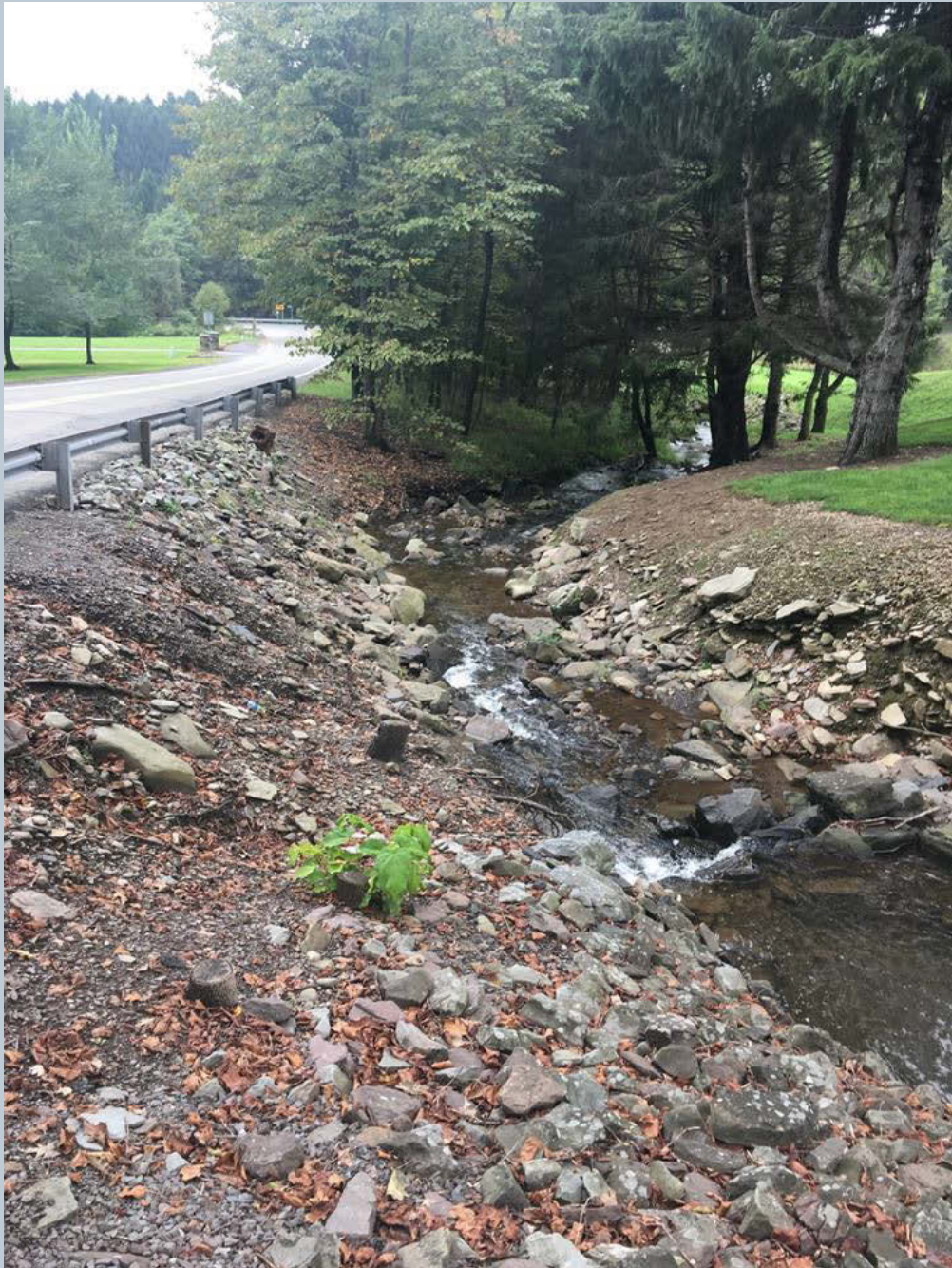
Figure 24a. A shot looking upstream toward the culvert along a private driveway.
