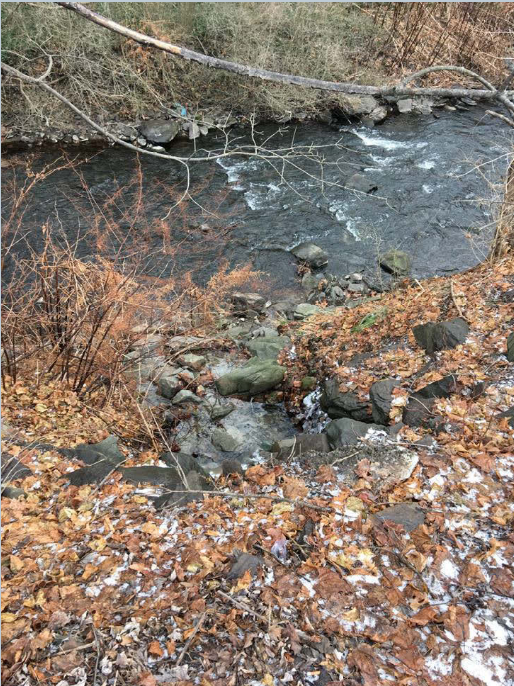
Figure 93. Taken looking downstream on Toby Creek at a scour pool that has resulted from a 24-inch concrete stormwater outfall pipe structure.
