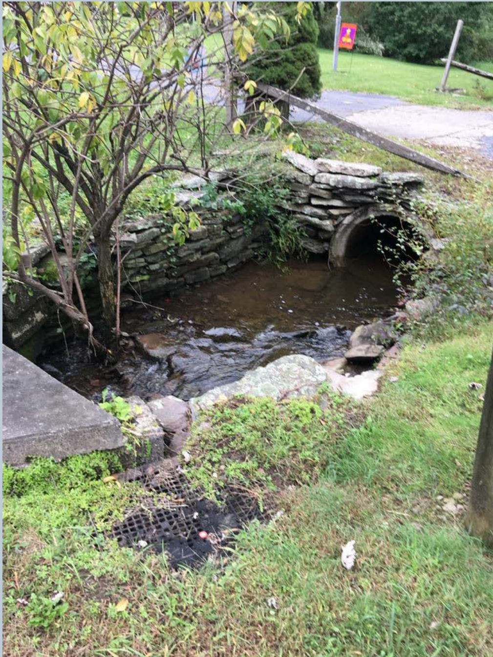
Figure 49. A headwall and concrete culvert pipe along the cul de sac on Ferguson Avenue. This is a shot of a 12-foot section of the unnamed tributary to Toby Creek.
