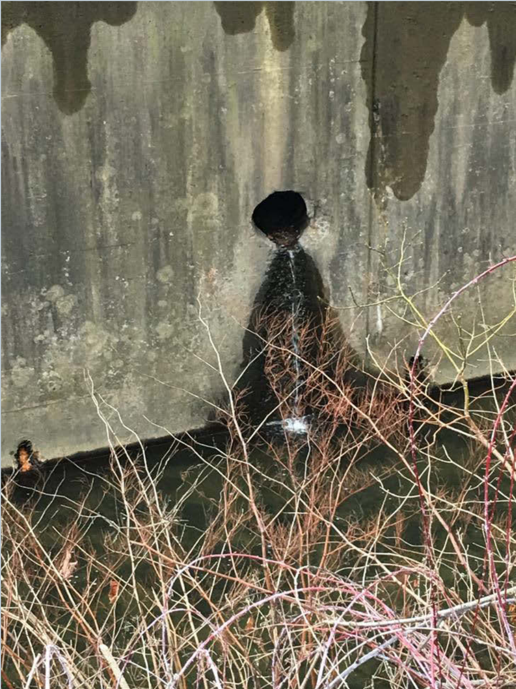
Figure 143. An UNT to Toby Creek outfall from 12-inch opening in retaining wall from State Route 309.
