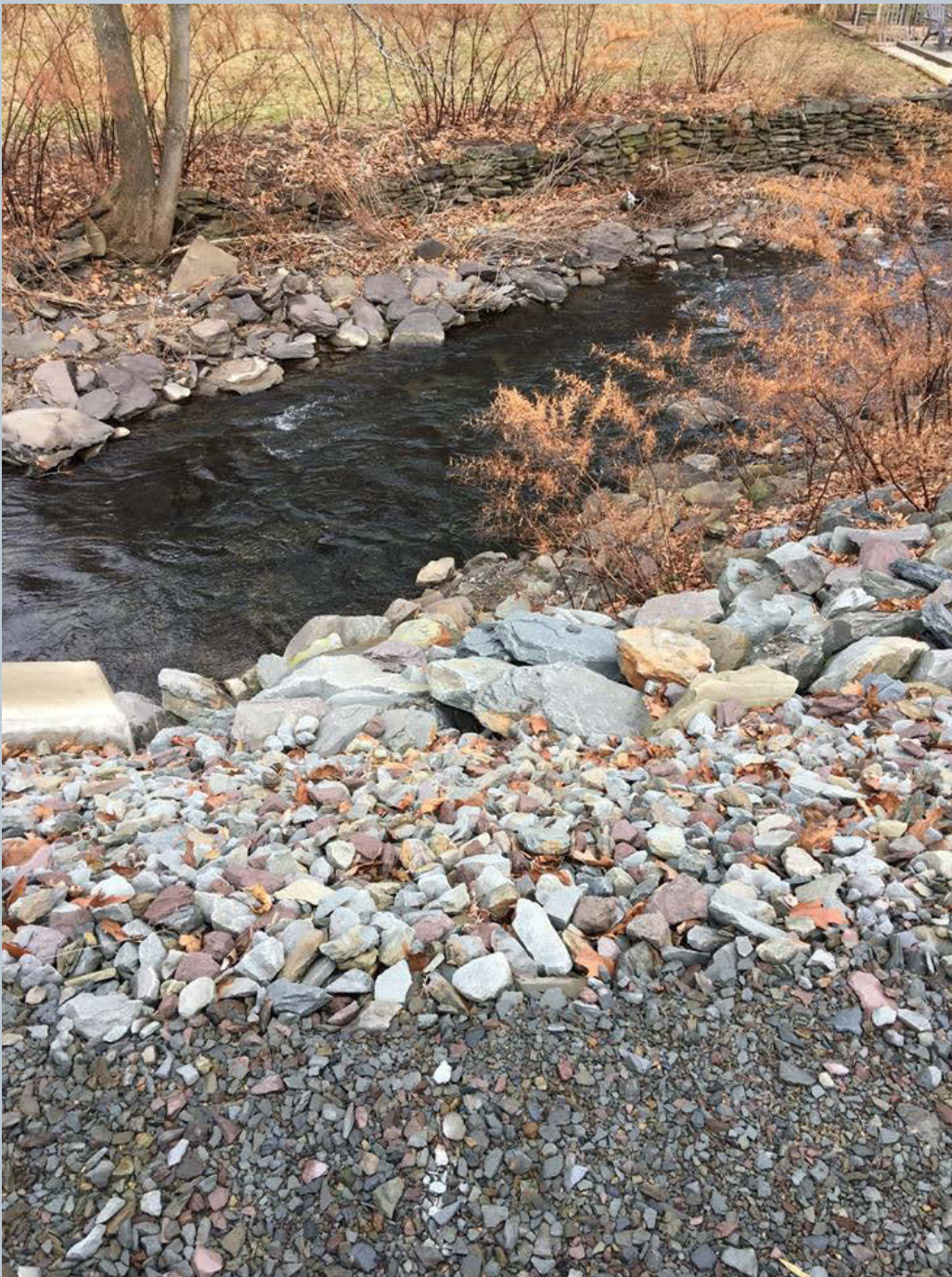
Figure 125. Looking downstream at an 18-inch galvanized stormwater pipe (dry) structure, covered with rip rap for protection. The structure is aligned to Toby Creek from the drop inlet structure on the closed bridge over N. Main Street.
