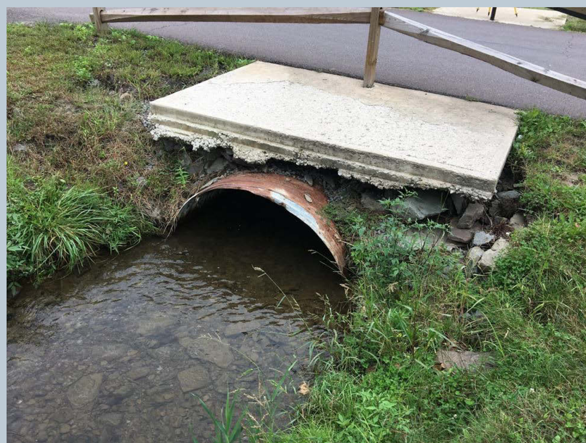
Figure 43. Looking upstream on corrugated squash pipe under Echo Valley Drive. This unnamed tributary is sediment-laden. (There is another unnamed tributary to the Green Pond unnamed tributary on the opposite side of Echo Valley Drive that was inaccessible).
