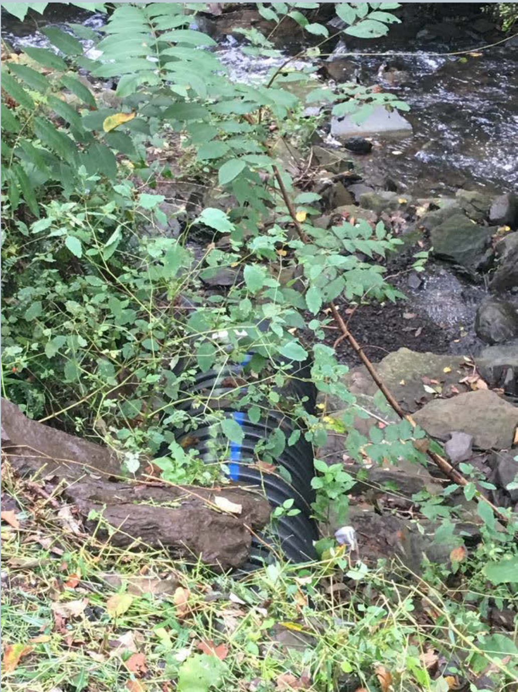
Figure 18. An 18-inch black HDPE stormwater pipe found 6 feet above the Green Pond unnamed tributary. There is no rock apron; it is recommended to either use existing rocks in the channel to construct an apron or cut the length of the pipe back.
