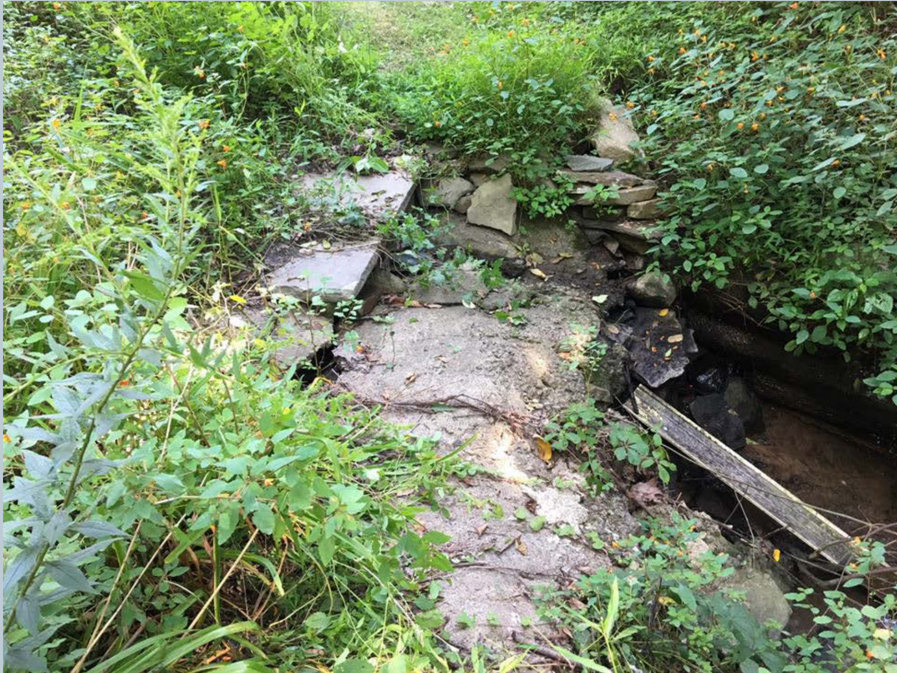
Figure 183. A shot of some rip-rap impediment on the UNT. This impediment could be removed and replaced with a small cross-vane to keep the flow of the UNT in the center of the stream channel to allow the high water flows to pass under the covered bridge. Some engineering may be necessary in this location.
