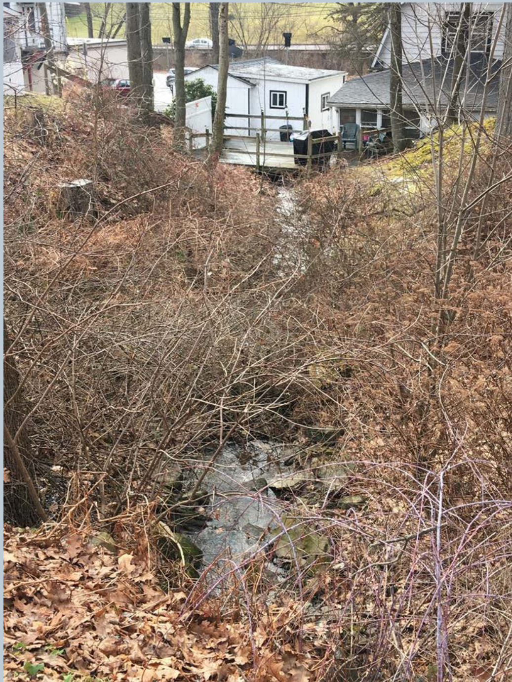
Figure 121. An UNT to Toby Creek that flows through a stone culvert beneath Railroad Street, directly under the deck and shed of a private residence on the corner of N. Main Street and Division Street.
