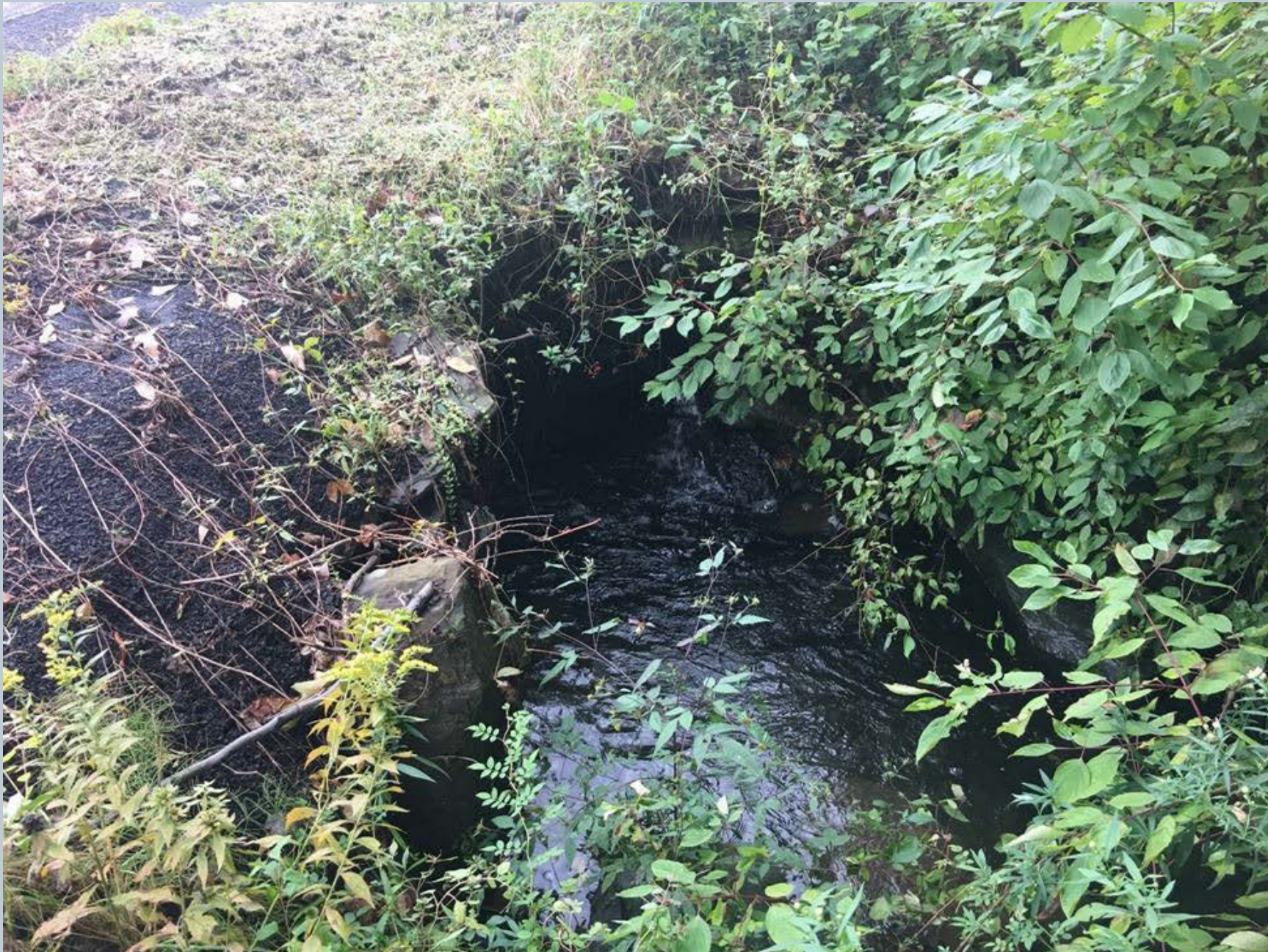
Figure 12. The Green Pond unnamed tributary flows across Harris Hill Road at this location. A 12-inch stormwater pipe in the unnamed tributary flows into a heavily wooded area before heading downstream along Harris Hill Road.
