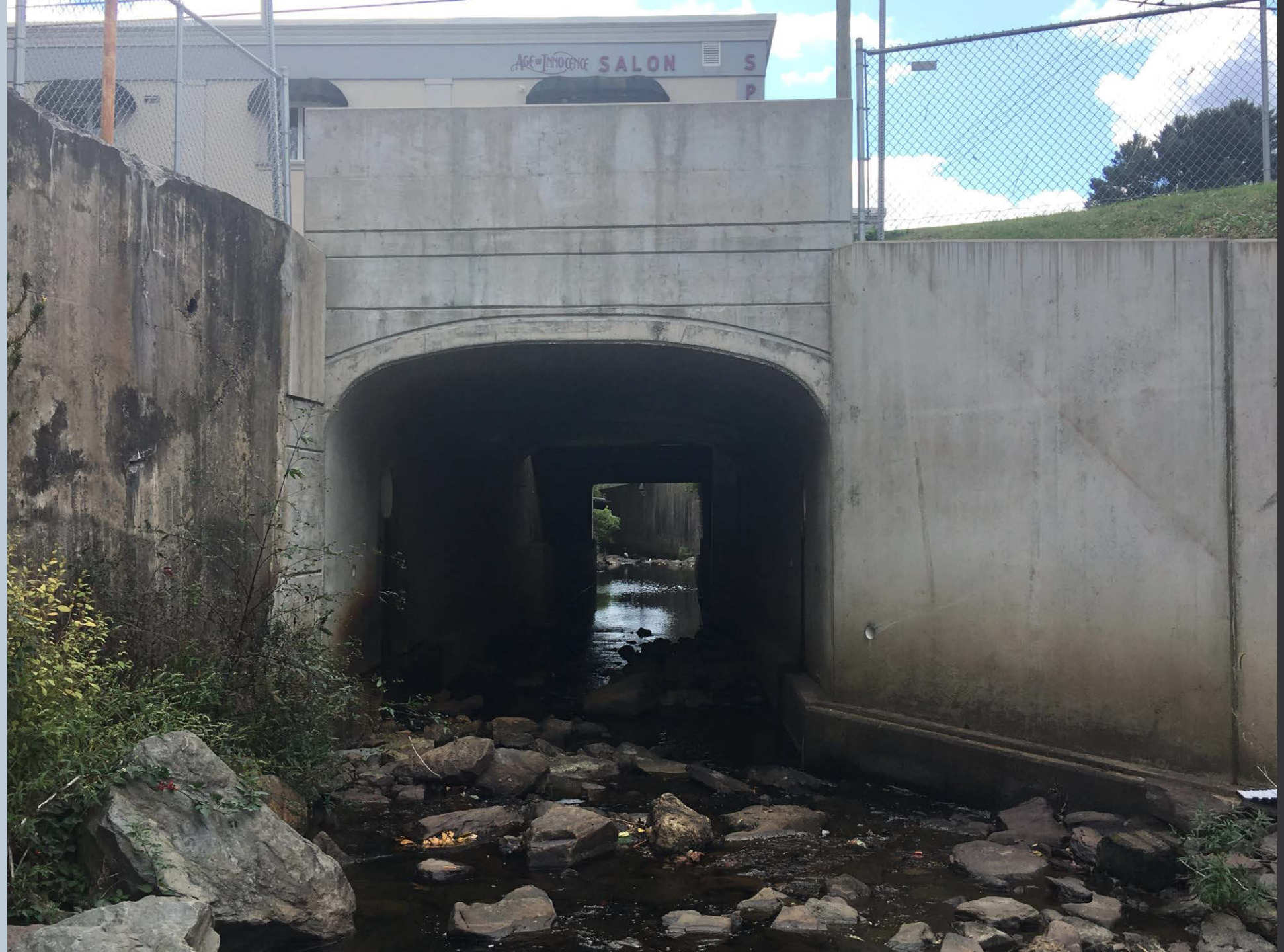
Figure 294. Looking downstream on Toby Creek along W. Center Street. Several storm drains from W. Center drop stormwater runoff along the concrete walls beneath the bridge into Toby Creek.
