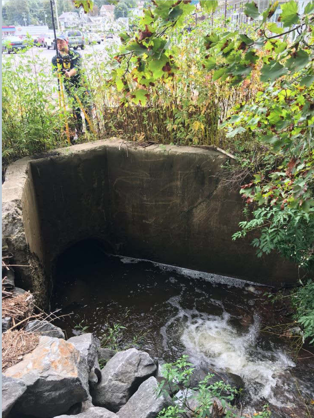
Figure 55. A wingwall box culvert. This shot shows a small plunge pool looking downstream towards the Dollar General parking lot. The culvert flows under the Dollar General Parking lot.
