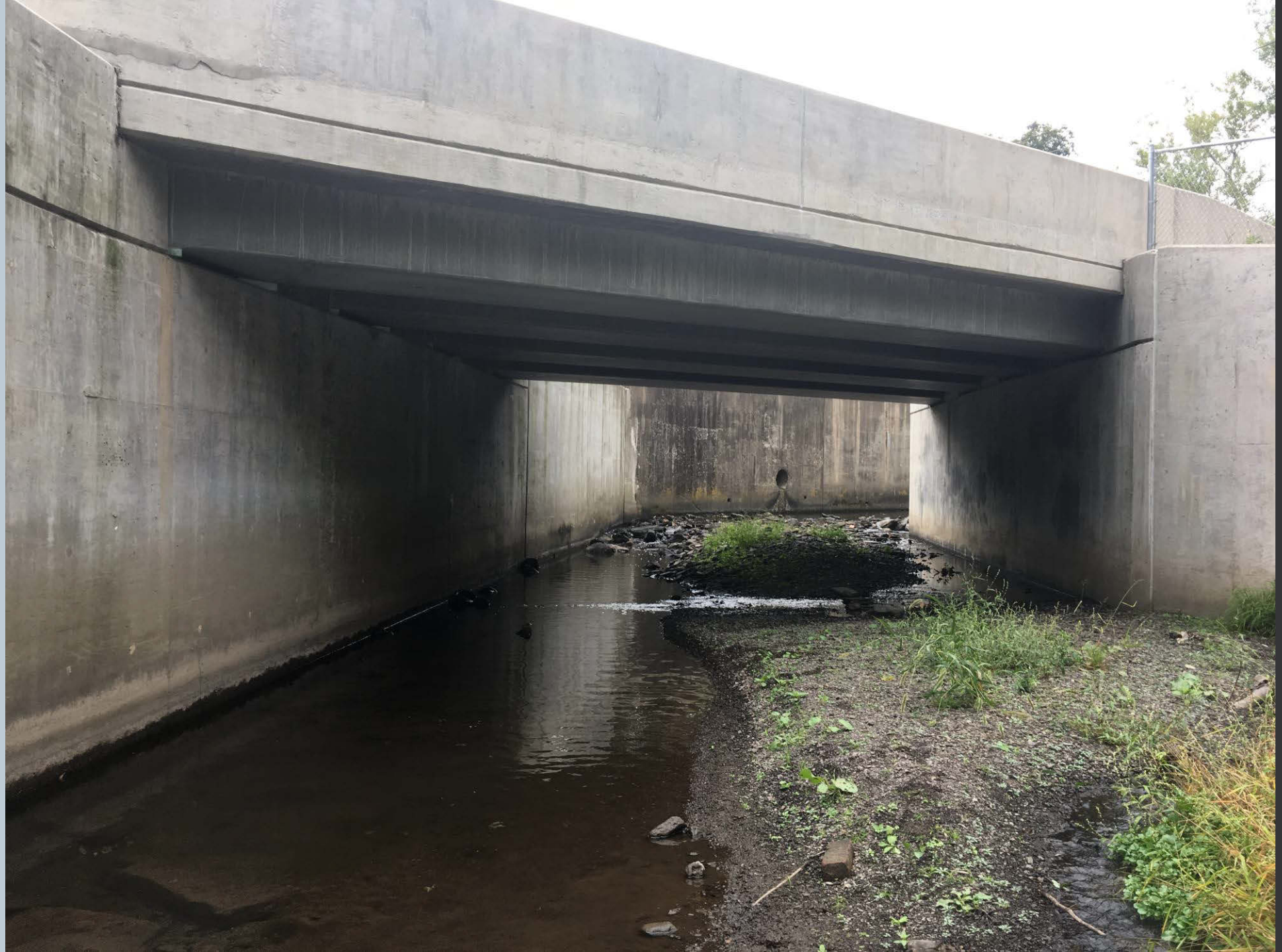
Figure 291. Looking upstream on Toby Creek along N. Main Street where the new bridge was constructed where a point bar extends from beneath the bridge from the outlet. Recommend point bar removal at the other end of the bridge.
