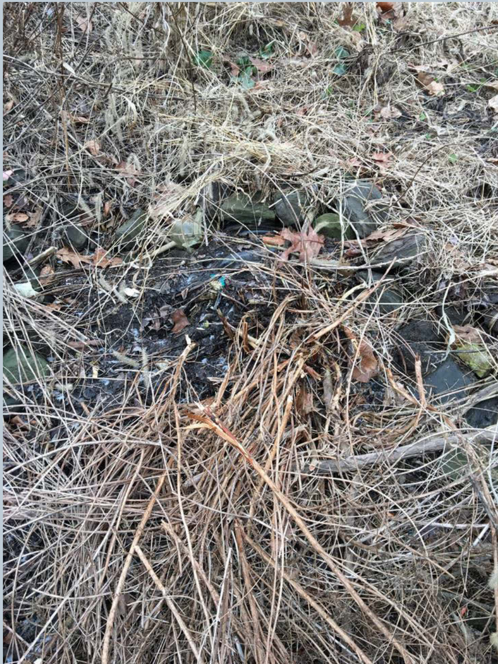
Figure 135. An 18-inch black HDPE stormwater pipe that is 100% blocked with sediment from the storm drain drop box inlet along State Route 309, that is filled and covered with leaves.
