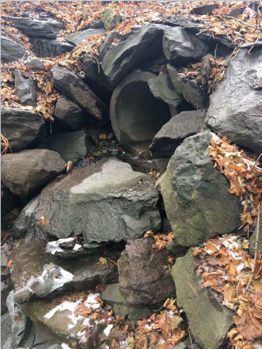
Figure 92. A shot of a dry 24-inch concrete stormwater outfall pipe structure that is located along the left bank of Toby Creek, looking upstream along State Route 309. This structure is draining stormwater from S. Pioneer Avenue and State Route 309.
