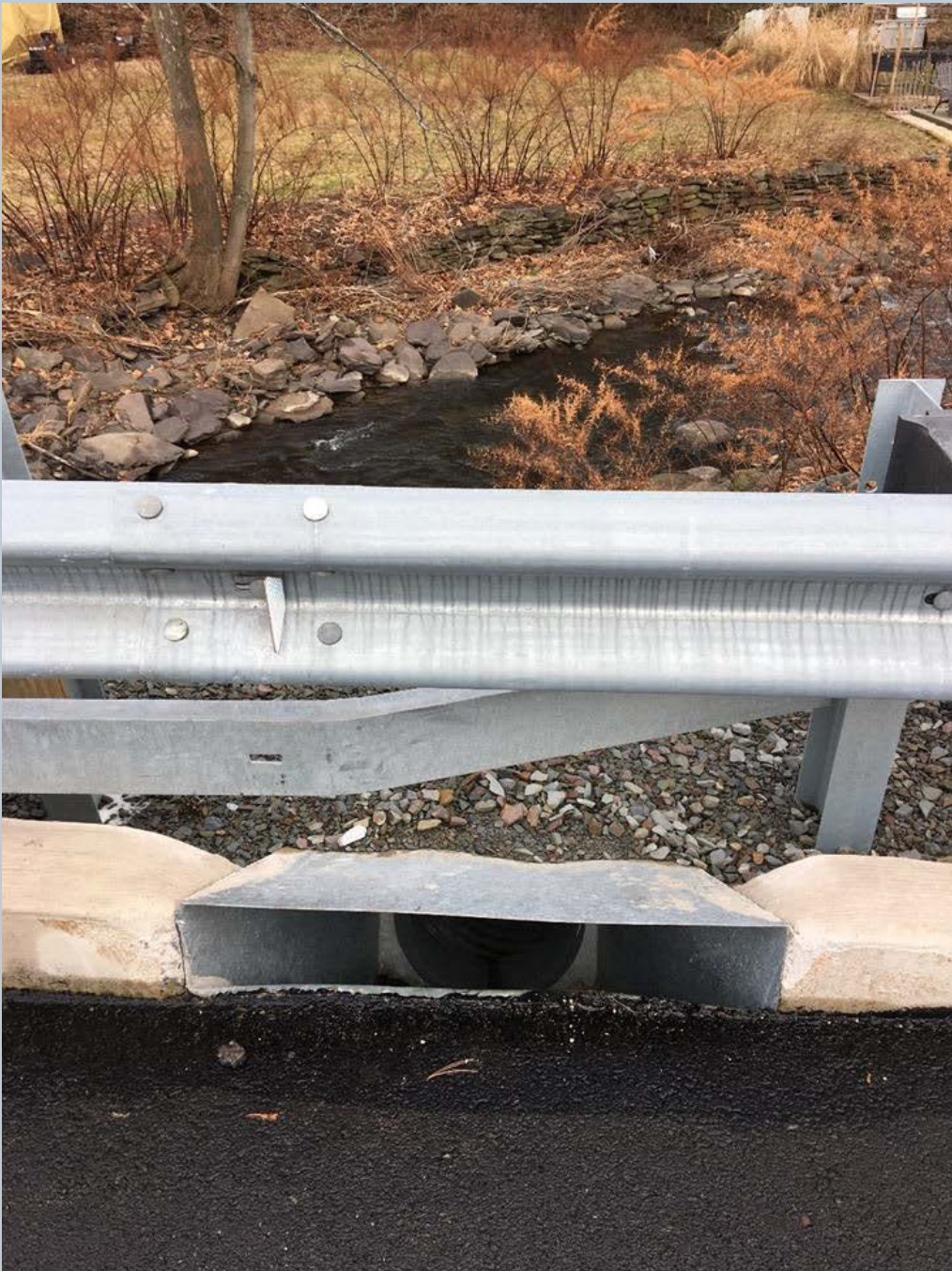
Figure 124. An image of a galvanized sheet metal drop inlet stormwater structure on the closed bridge over N. Main Street.
