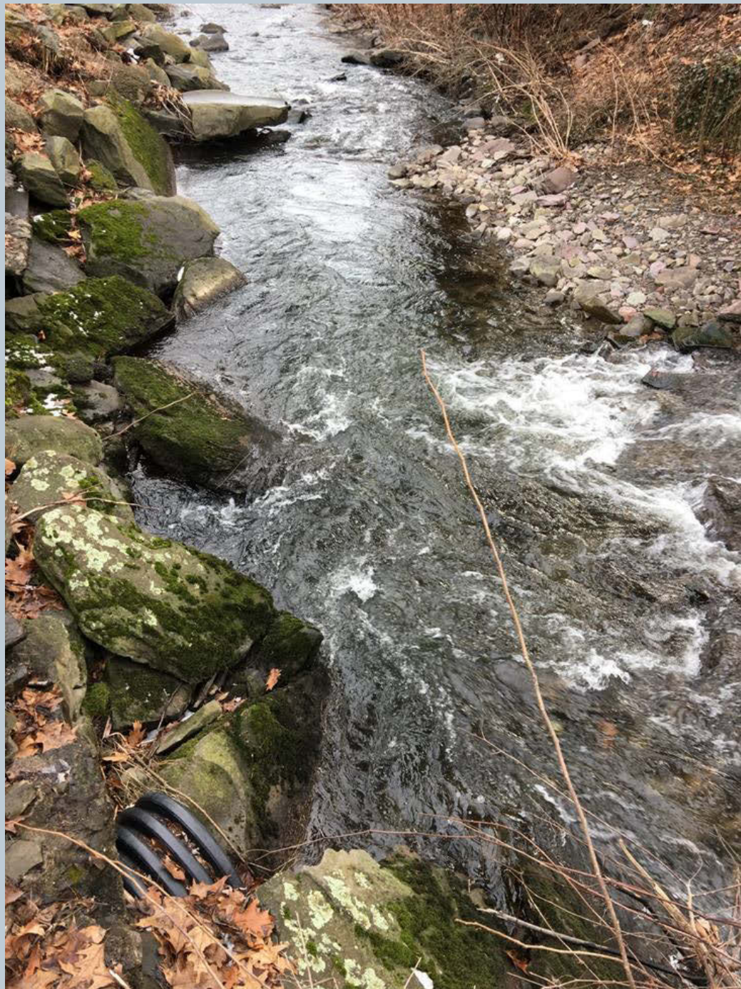
Figure 126. A 24-inch black dry HDPE pipe for stormwater across N. Main Street is aligned with Toby Creek, looking downstream. Gravel bar deposition is present on the outside bend of Toby Creek. Additionally, N. Main Street was previously undercut in this area.
