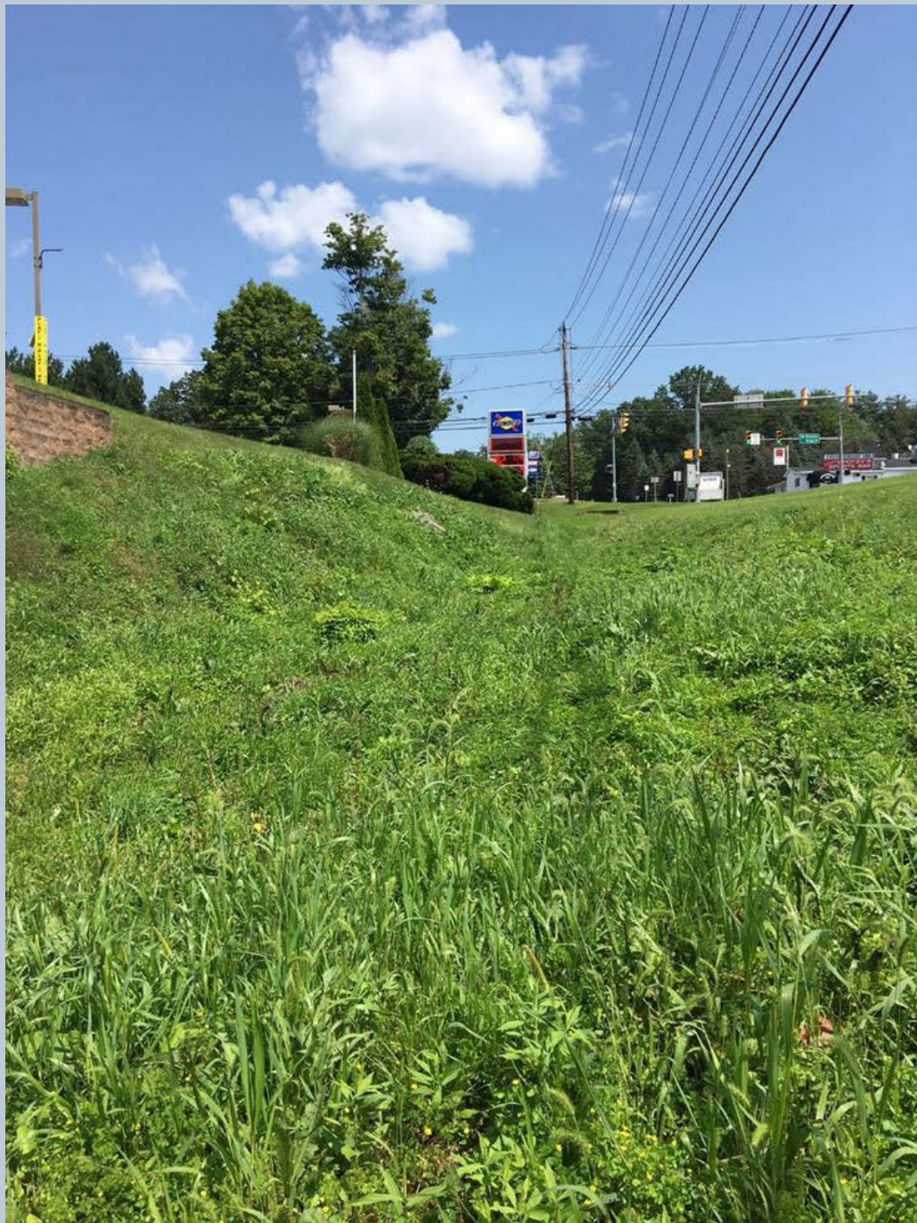
Figure 191. Two smaller stormwater headwalls with 18-inch pipes feed runoff towards a grassed waterway conveyance swale that is well vegetated and full of poison ivy.
