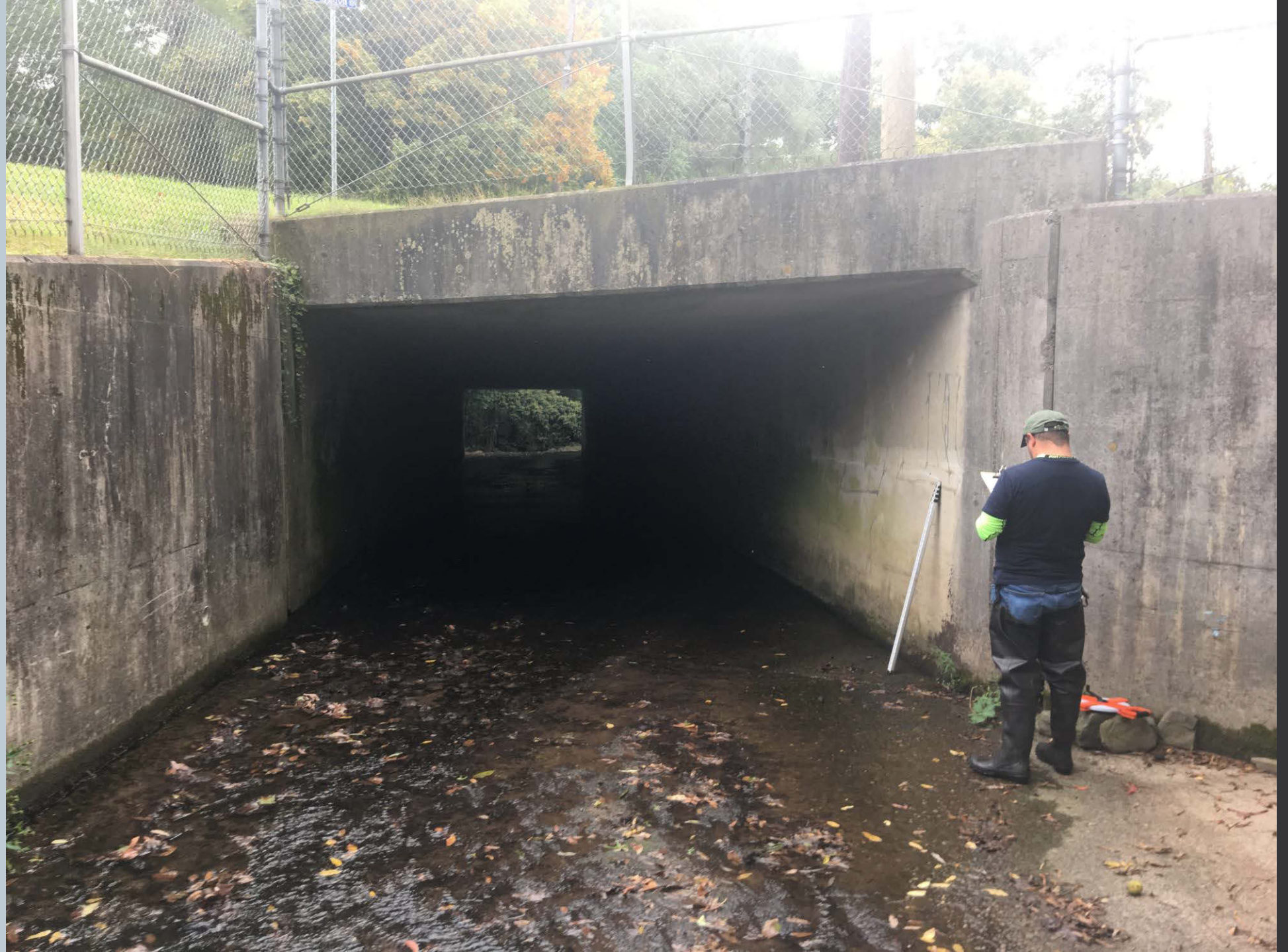
Figure 302. Bridge culvert over Carverton Road looking downstream on the unnamed tributary with Tom Mayka, DAMA Stormwater Coordinator where the concrete footer meets the unnamed tributary.
