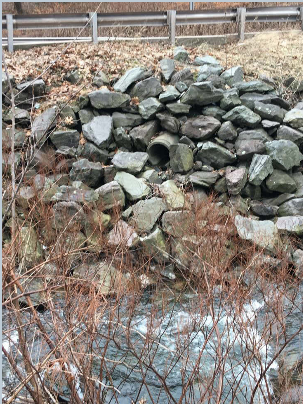
Figure 142. A shot of a 12-inch concrete outfall stormwater pipe (dry) structure aligned with Toby Creek. This is located along State Route 309 with rip-rap present.
