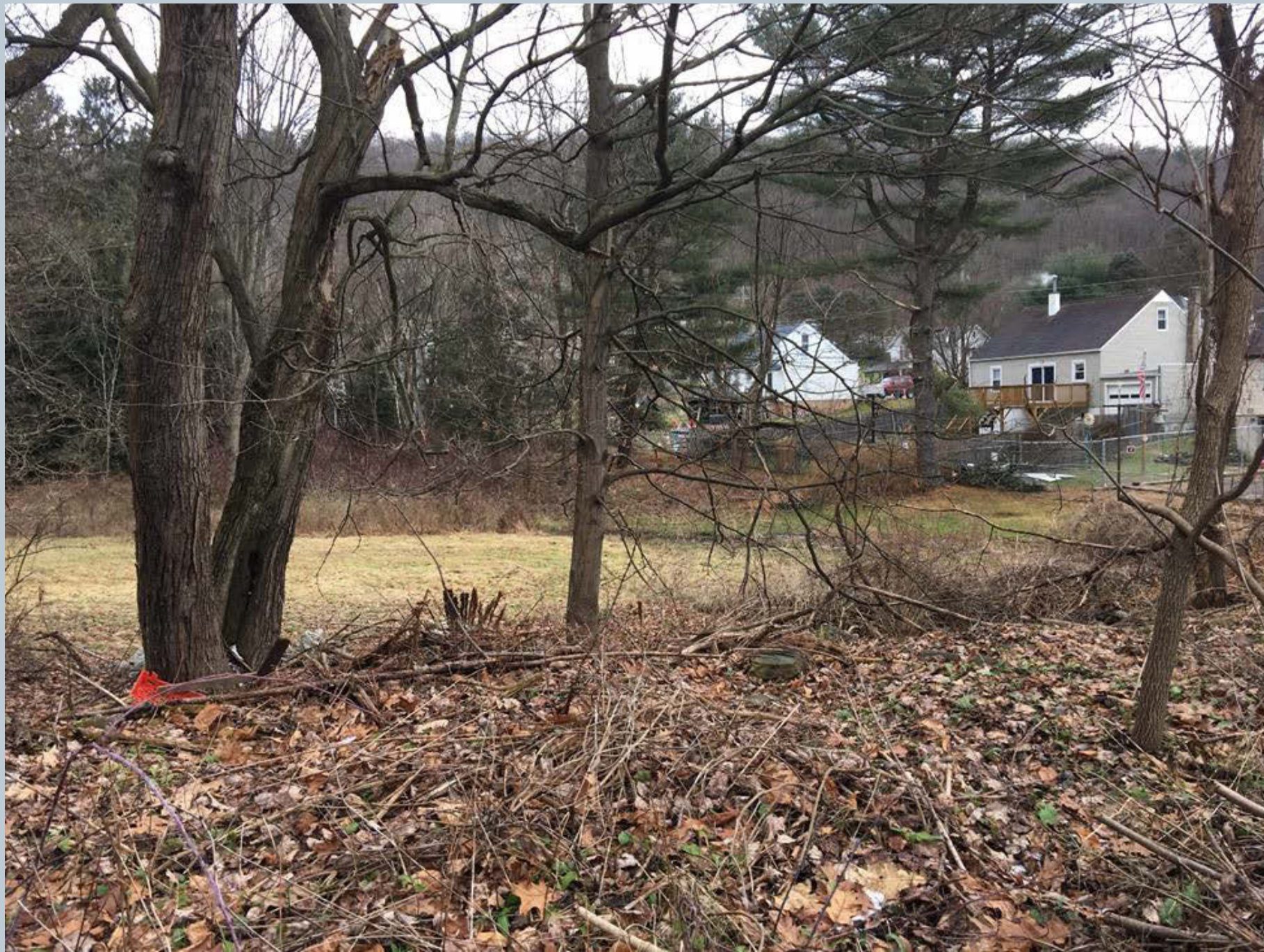
Figure 122. An UNT located upstream of Railroad Street in a wetland area, before entering the stone culvert under Railroad Street. In the future, this could possibly be a detention area and wetland enhanced basin to reduce the flow and slow down the UNT through the stone culvert. The property owner(s) will need to be identified to discuss further possibilities.
