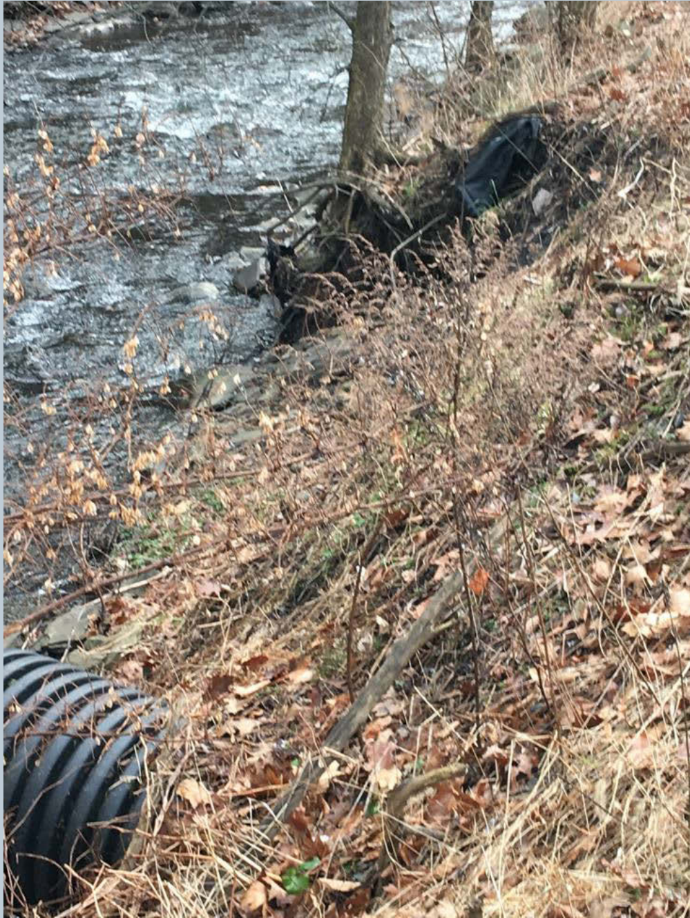
Figure 111. A shot of some minor streambank erosion on the right bank of Toby Creek, looking downstream, just beyond the broken HDPE pipe.
