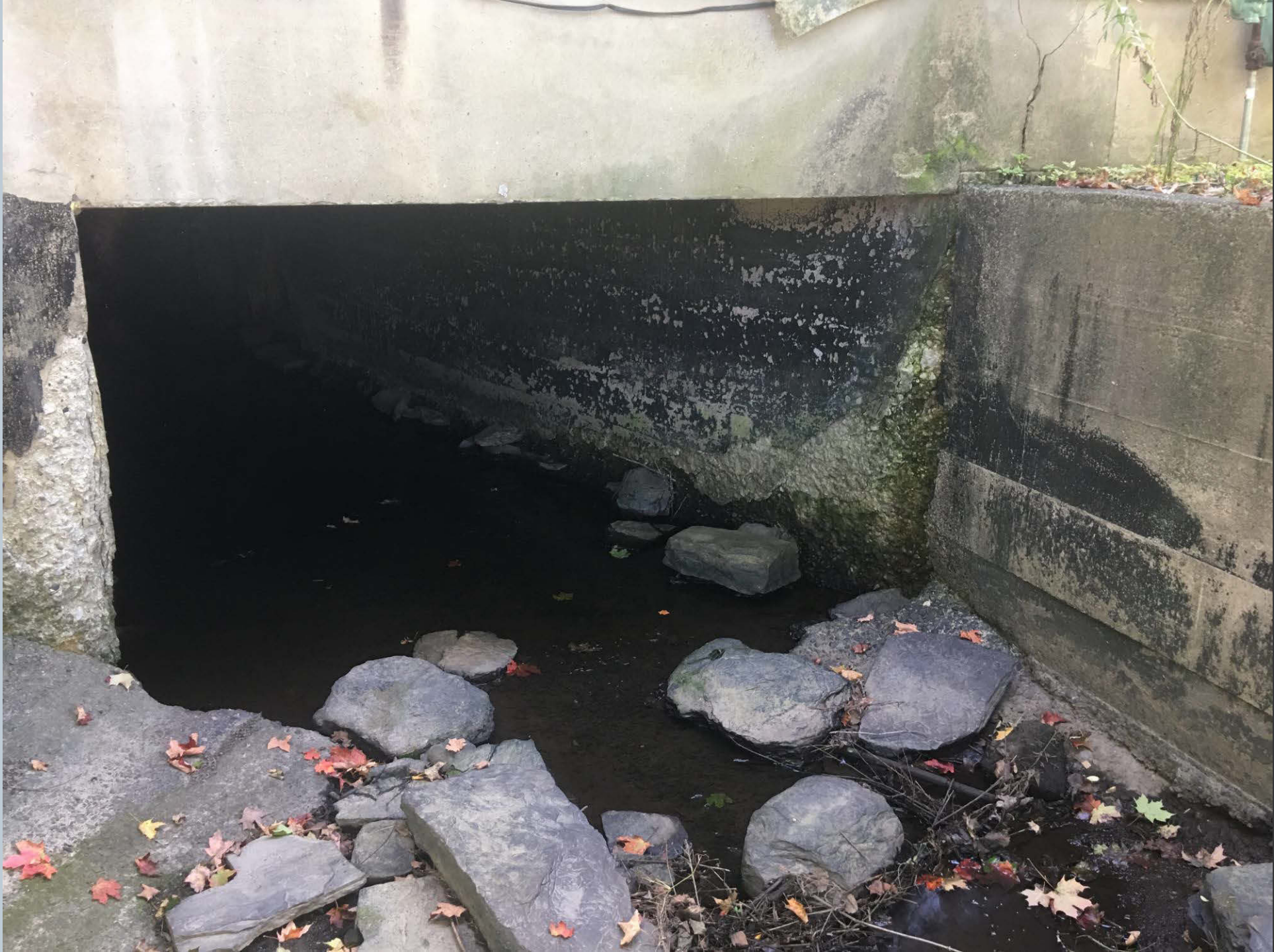
Figure 250. Culvert that directs Toby Creek from beneath Main Street, under the commercial district, until it outlets along Verve Vertu in Dallas. This is an open section before going into another culvert under the commercial district in Dallas.
