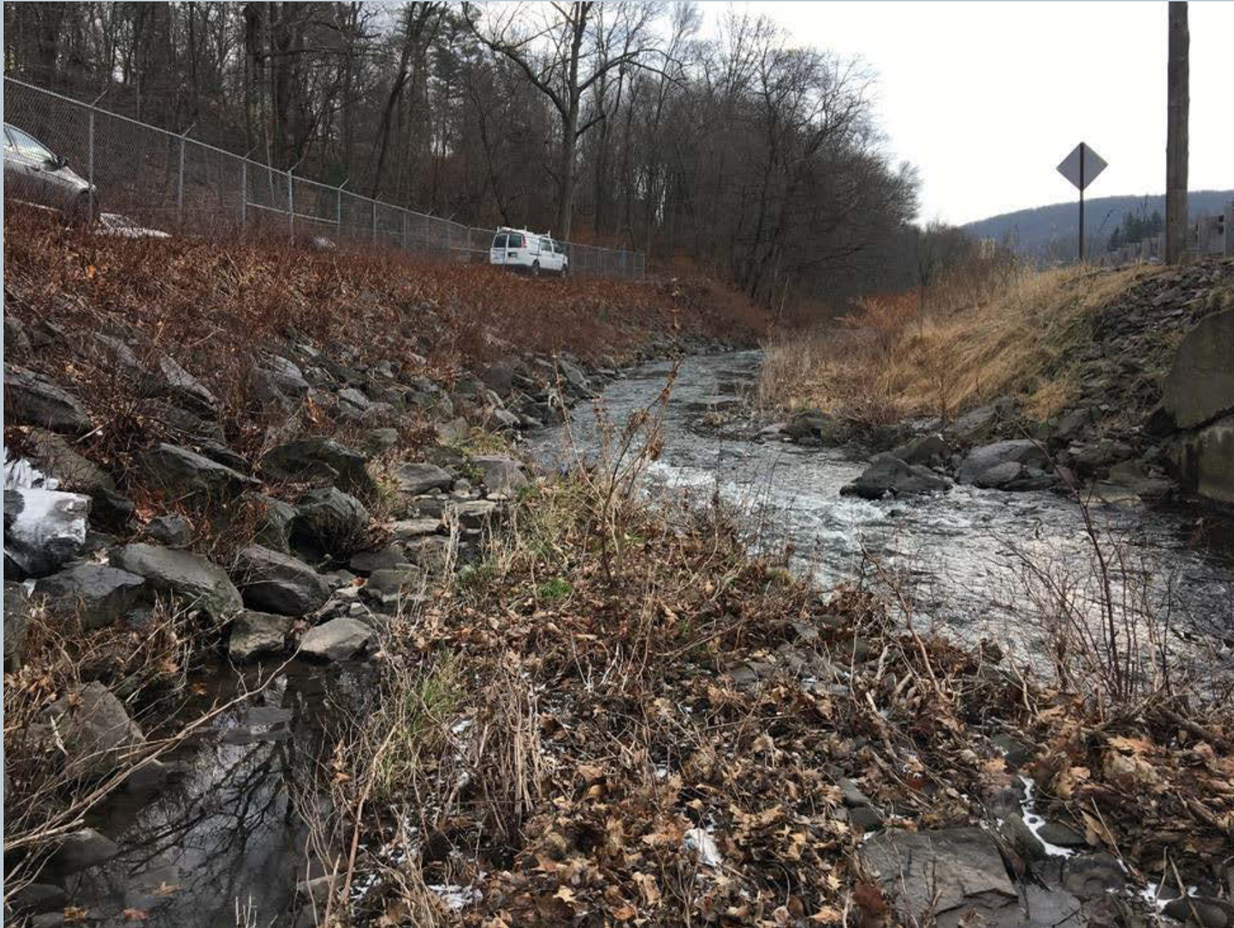
Figure 97. A shot looking downstream on Toby Creek from a historic hard-armored streambank stabilization project. Aggradation of cobble and gravel in the right box culvert, under the bridge over State Route 309, has created point bar gravel and cobble deposition.
