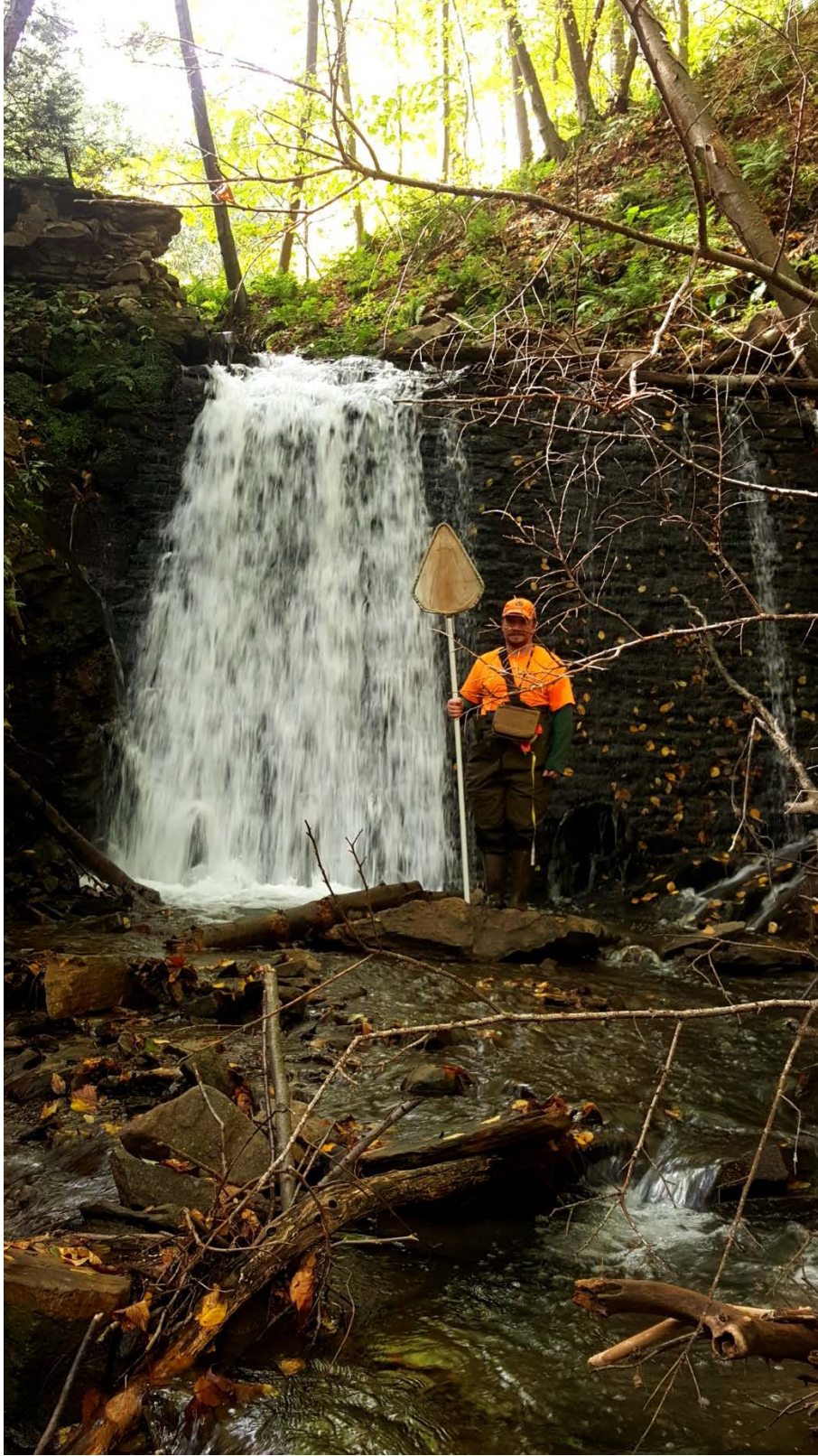
Figure 5. EPCAMR staff Michael Hewitt stands next to a structure of hand laid stone that creates a large cascade waterfall. Approximately 0.5 miles upstream from Shoemaker Avenue.
